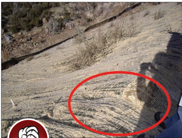
Fig. 2-5. This jute netting is physically deteriorating and requires replacement.
