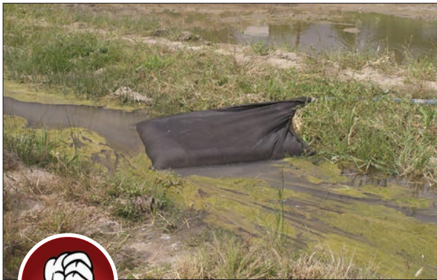
Fig. 3-17. This dewatering bag should not be located in a water course.
