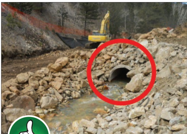
Fig. 5-4. This is a good application of a temporary culvert. Note the riprap approach to the culvert.
