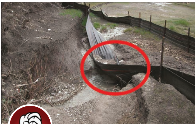
Fig. 3-14. This silt fence is poorly maintained. Accumulated sediment should be removed. Silt fence should not be installed in a water course.
