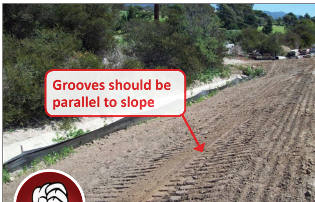
Fig. 4-3. Surface roughening is shown correct near the top of the slope; however shallow grooves in the lower half are in the wrong direction.
