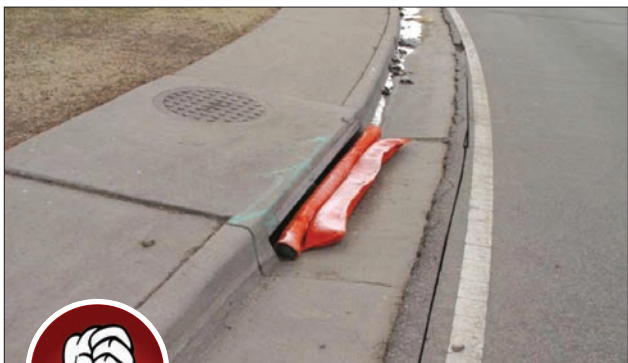
Fig. 5-14. The sock should extend at least one foot past each end of the inlet.
