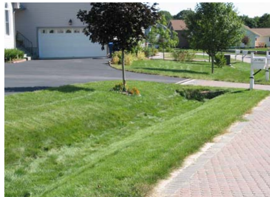
Figures 4.20 – Vegetated drainage way. Photograph courtesy of the University of Connecticut NEMO program, Kara Bonsack
