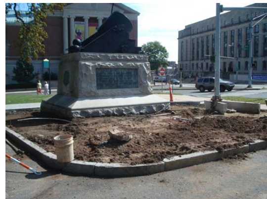
Figure 3.14 – Construction of a rain garden at Hartford Green Capitols Project. Source: Camp Dresser & McKee.
