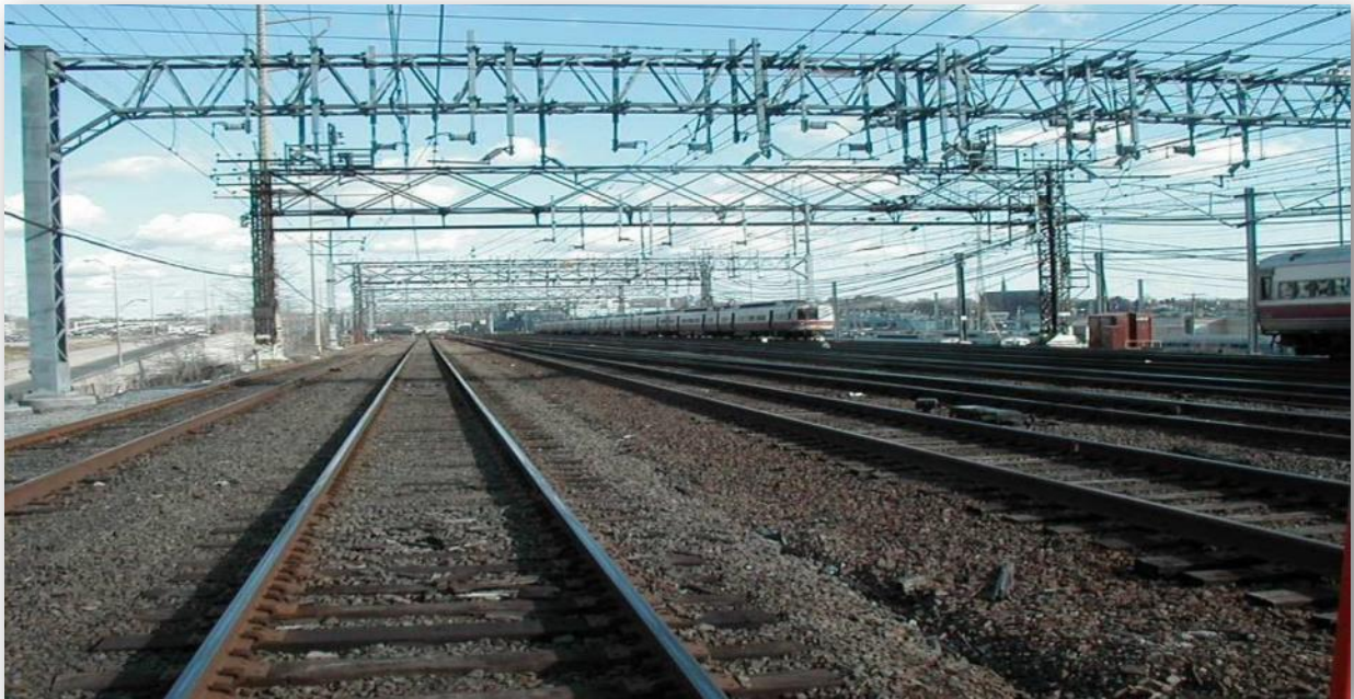
Figure 5-7. Photograph of the New Haven Line Catenary
