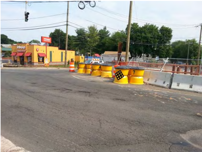
West Main Street: The Impact Attenuation System on the east side of the project site.
