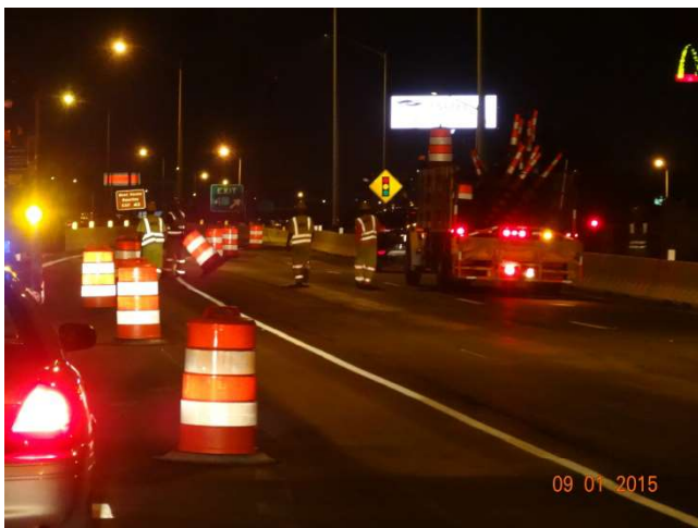
I-95 SB: The sign pattern crew placing traffic drums to take the right lane and close the next exit.
