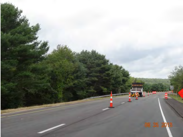
Route 11 NB: The left lane closed with the use of traffic cones and a TMA in the closed lane with a straight bar warning light to signal lane is closed.
