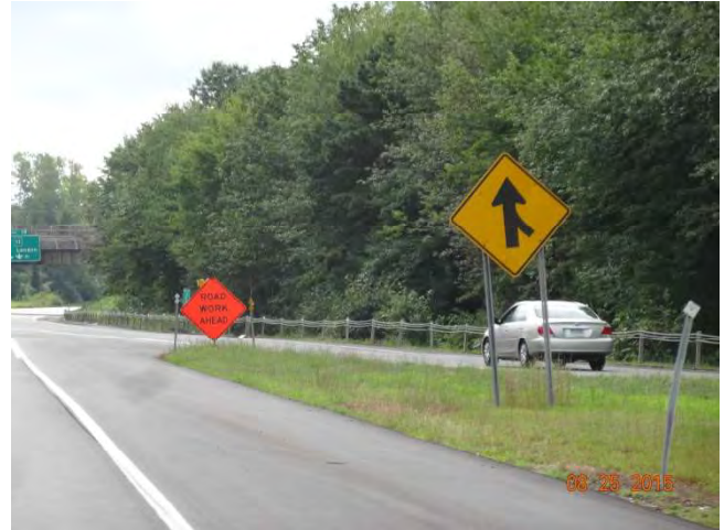
Route 11 SB: A temporary ROAD WORK AHEAD sign with a high-intensity barricade warning light attached.
