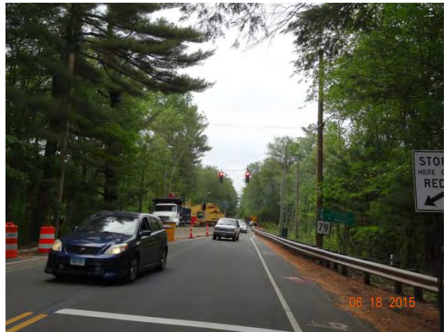
Route 79 SB: Traffic heading north signaled to go through the one-lane road.
