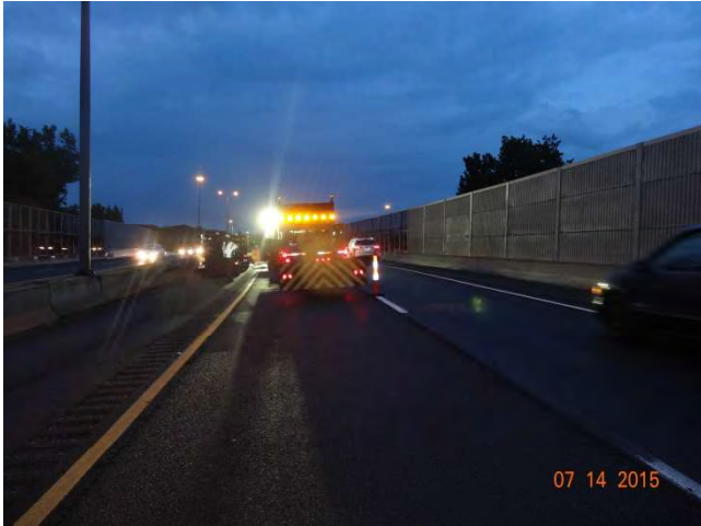
Route 15 NB: The truck-mounted attenuator with the flashing arrow signaling the lane is closed.
