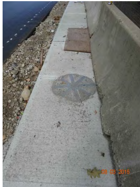
Route 73 NB: A manhole cover over with plastic and tape to prevent it being sealed from the concrete pour for the sidewalk.
