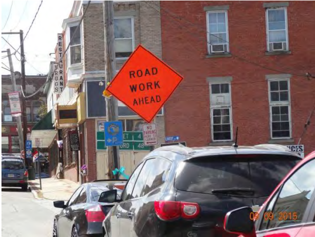
School Street (Route 44/12) WB: A post-mounted ROAD WORK AHEAD sign with a barricade warning light affixed.
