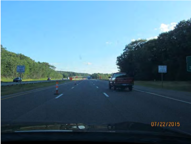
I-84 WB: Post-mounted ROAD WORK AHEAD FINES DOUBLED signs on both sides of the highway.
