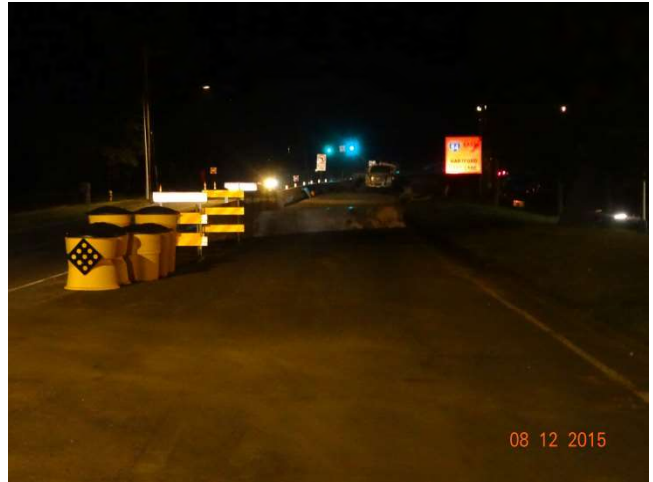
I-84 EB: A new lane that will be constructed for the traffic shift. A Type A Impact Attenuation System in front of the barrier and a construction sign that says I-84 EAST HARTFORD LEFT LANE.
