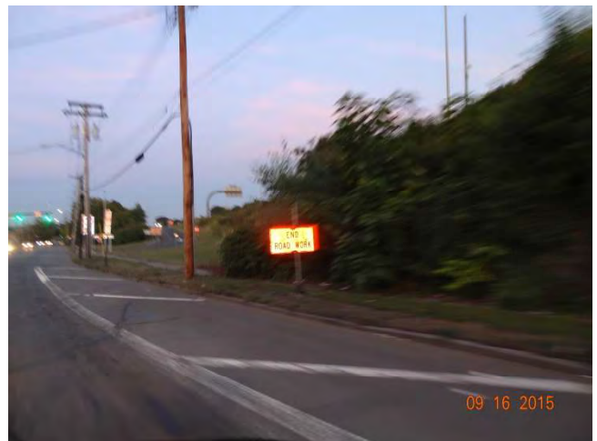
Middletown Avenue: An END ROAD WORK sign right before the Exit 7 on ramp.
