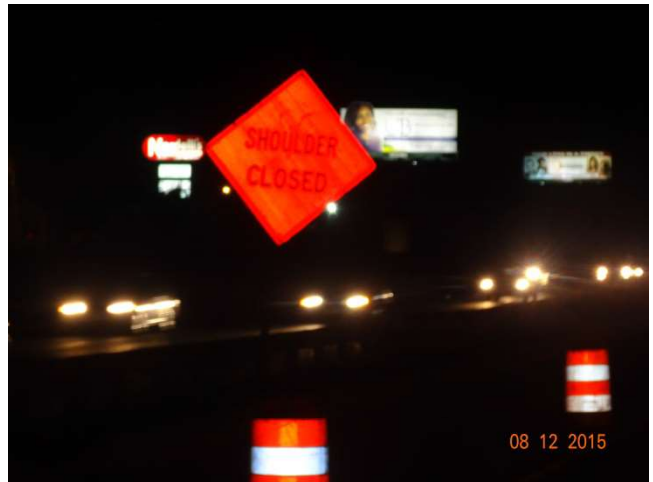
I-84 EB: A post-mounted SHOULDER CLOSED sign on the median without a warning light.
