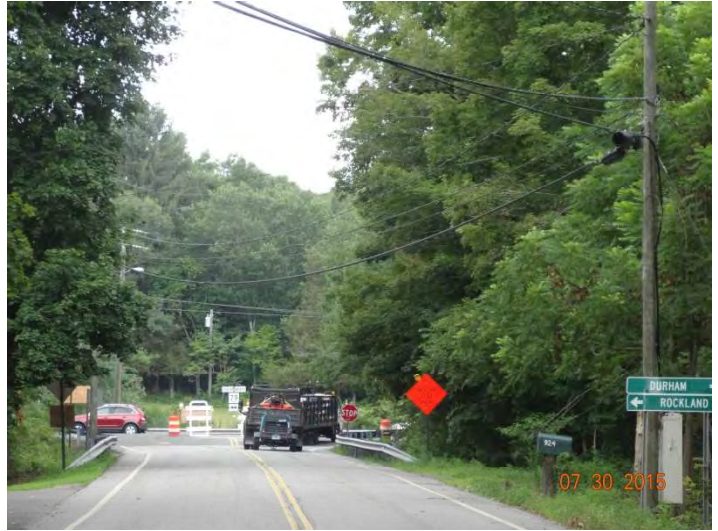
Route 148 WB: Construction trucks leaving the closed road and entering Route 79 traffic.
