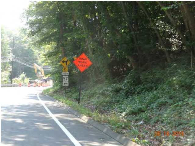
Route 57 SB: A post-mounted ROAD WORK AHEAD sign with a high-intensity barricade warning light.
