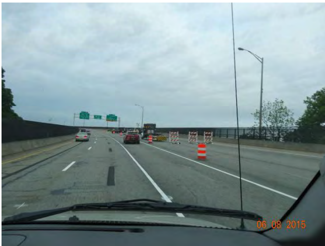
I-95 NB: Barricades and crash truck closing off lanes for work zone; traffic drums to delineate traffic for Exit 83 on ramp onto I-95
