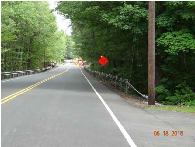
Route 79 NB: A “One Lane Road Ahead” sign with a high-intensity warning light that is flashing
