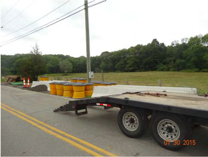
Route 148 EB: Material stored on the side of the road within the closed section of the road.
