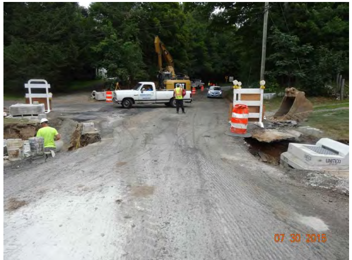
Route 148 EB: Another work crew working on the structures on the side of the road.
