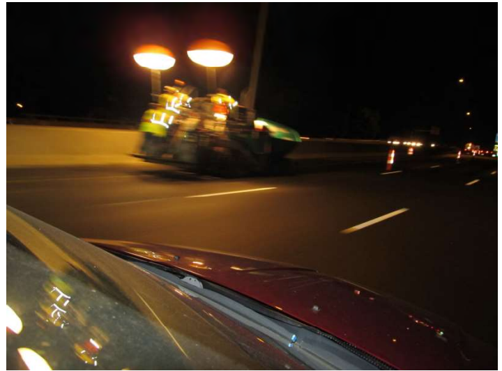
I-95 NB: The paver with balloon lights that prevents bright lighting from shining into the motorists line of sight.
