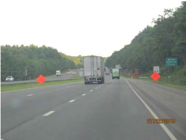
I-84 WB: ROAD WORK AHEAD on both sides of highway with the Changeable Message Sign behind them.
