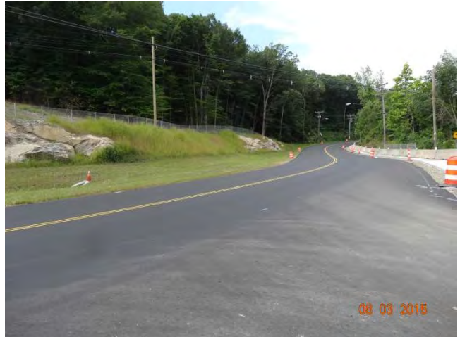
Route 73 NB: Newly paved roadway with traffic devices along the sides covering structures in the road.
