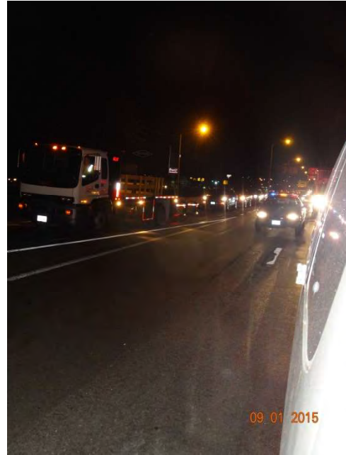
I-95 SB: State Police and the Contractor's work truck prohibiting traffic from proceeding while signs were installed.
