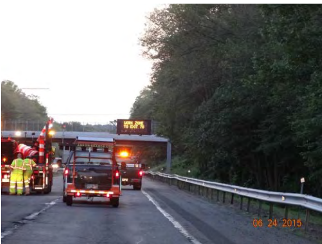
I-95 SB: The Variable Message Sign stating there's a work zone near Exit 70
