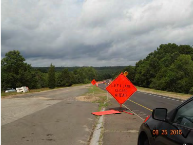
Route 11 NB: A temporary LEFT LANE CLOSED AHEAD sign with warning light and a merge right sign with warning light.
