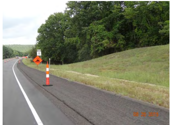
Route 11 NB: A traffic cone in the shoulder next to the uneven edge of pavement and a sign depicting UNEVEN PAVEMENT.
