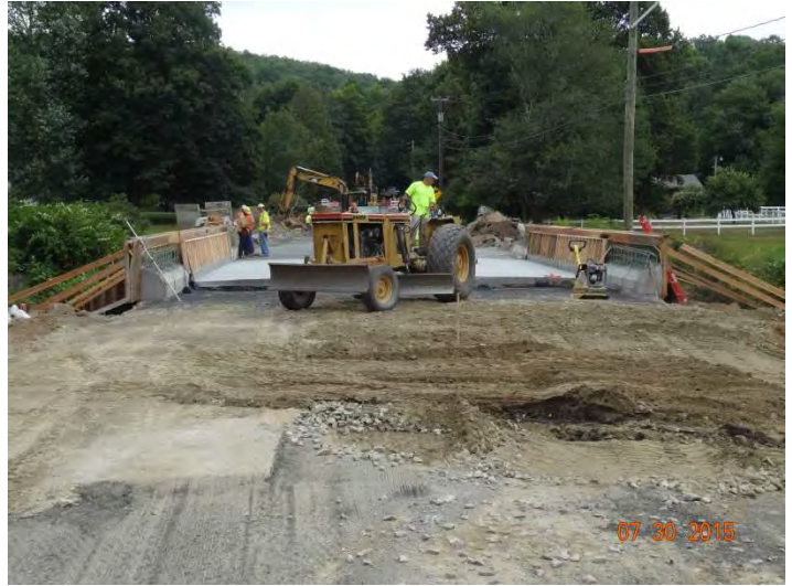
Route 148: The work crew fine grading the road for paving with the newly installed bridge in the rear.
