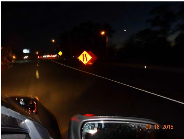
I-95 SB: A temporary merge left sign placed just before the Exit 8 off ramp since the taper starts just after the Exit 8 on ramp.
