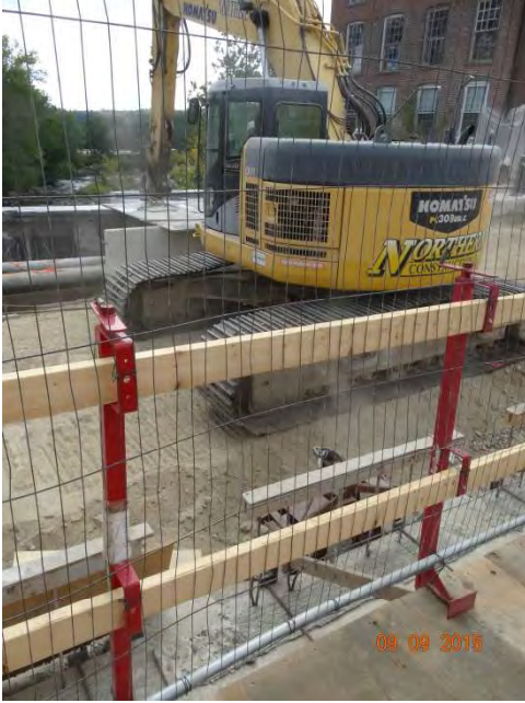
Pomfret Street (Route 44) EB: The work area on the right of the pathway.
