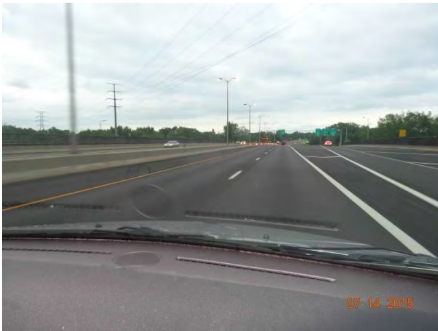
Route 15 NB: Approaching the work zone. A portable flashing arrow in the taper directing motorists to merge left.
