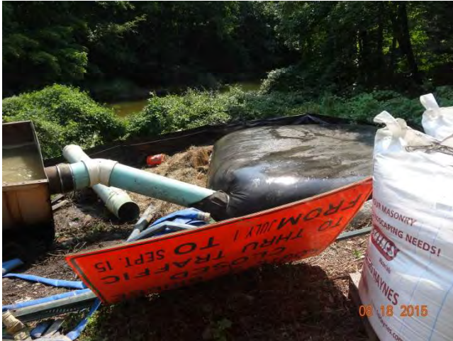
Route 57 NB: The filtration system for the water deviated from the brook.
