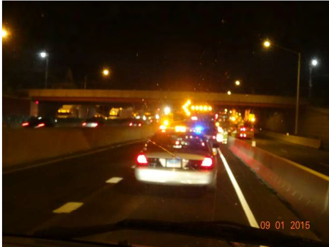
I-95 SB: State Police in the lane that is being taken, notifying the motorists of the approaching work zone.
