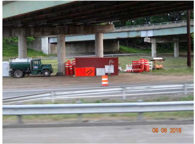
I-95 NB: The laydown yard has the proper clearance from the edge of road
