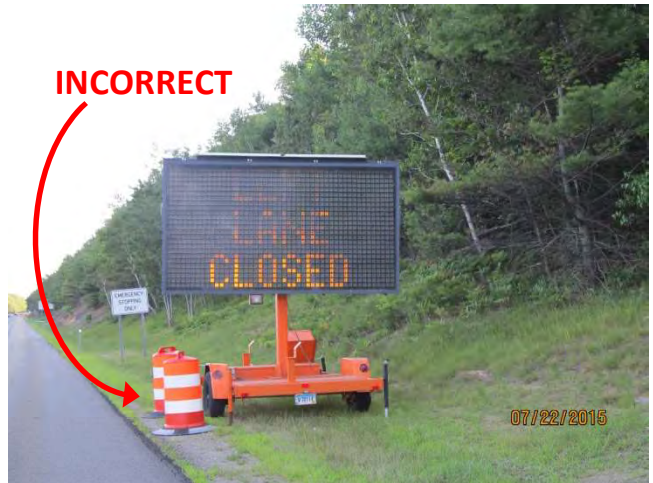
I-84 WB: The first frame for the Changeable Message Sign. The CMS is within 30 feet of the edge of the roadway and is improperly protected by two traffic drums. It should have positive protection around it if it is placed this close to road.
