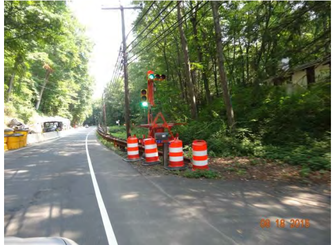
Route 53 NB: The green light of the temporary signal.
