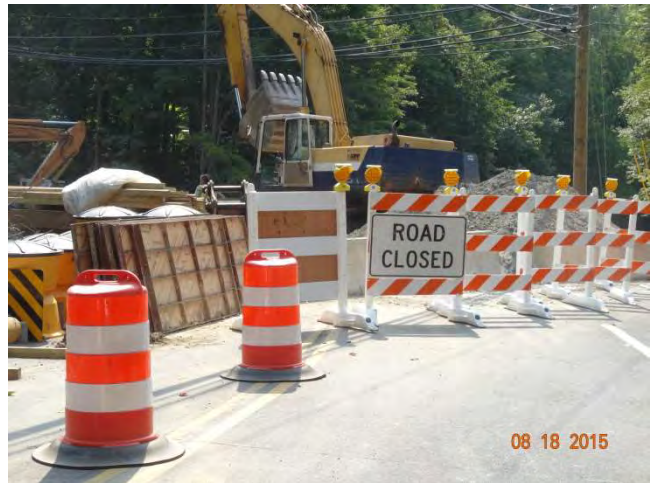
Route 57 SB: Type III barricades with high-intensity warning lights on top and a ROAD CLOSED sign attached in front. The plans called for a stop sign in front as well but with the angle of the barricades, motorists bypassing don't need to stop, they need to continue pass. A stop sign would be needed if motorists were trying to turn onto the roadway that was closed.
