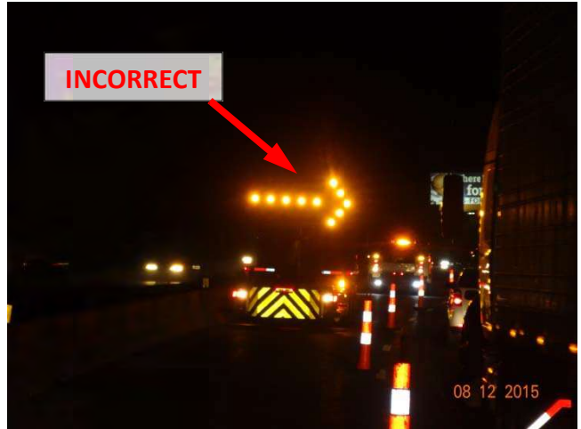
I-84 EB: An advance flashing arrow mounted on a truck-mounted impact attenuator in the closed lane signaling for traffic to merge right when it should be a straight bar to signal the lane is closed like stated in Section 4d in the M&PT special provision.
