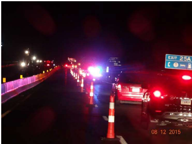
I-84 EB: The traffic being let through after the traffic pattern is finished being installed. The rolling road block start at 9:35 PM and ended at 9:54 PM.
