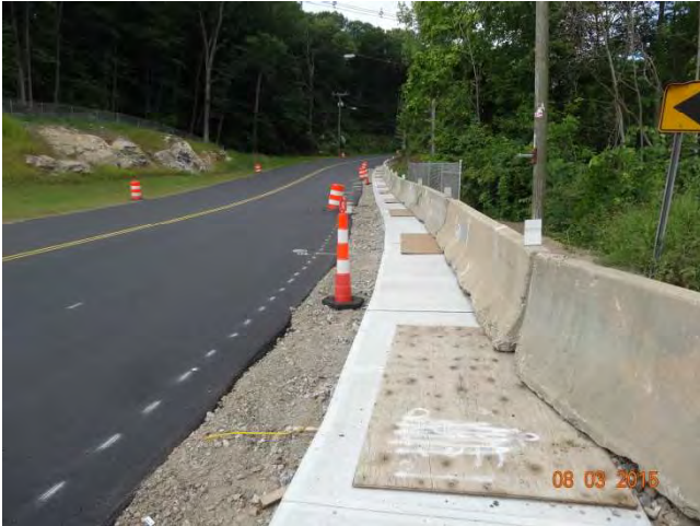
Route 73 NB: Concrete barrier that was previously separating the road from the pedestrian walkway. The Contractor put the barrier on the plywood to protect the new sidewalk but refused to cut it because they were good pieces. The large pieces of plywood were trip hazards to pedestrians using the sidewalk.
