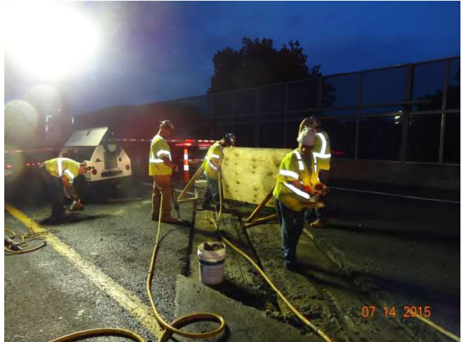
Route 15 NB: The Contractor's crew jack-hammering the concrete headers down on the bridge joint.
