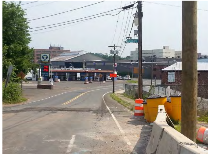
Burritt Street NB: The Impact Attenuation System on the north side of site and an END OF WORK sign mounted.
