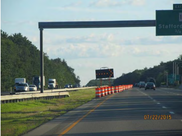
I-84 WB: The portable flashing arrow within the taper signaling to merge right.
