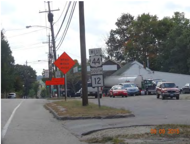
School Street (Route 44/12) WB: A post-mounted ROAD WORK AHEAD sign with a high-intensity barricade warning light attached.
