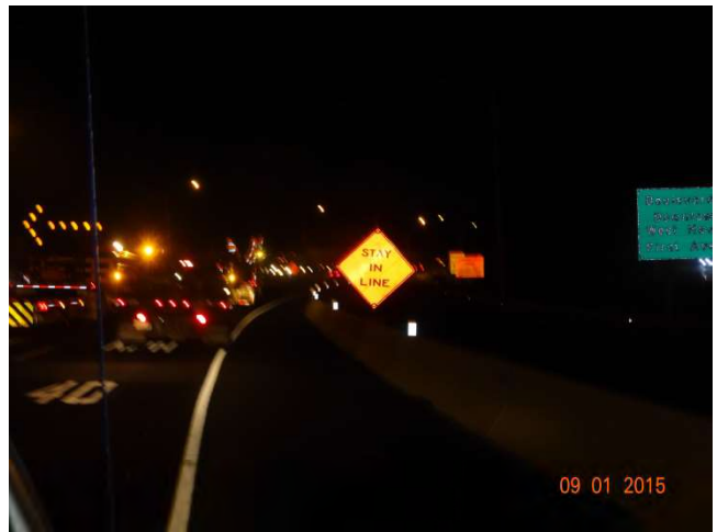
I-95 SB: A temporary STAY IN LINE sign in the right shoulder.
