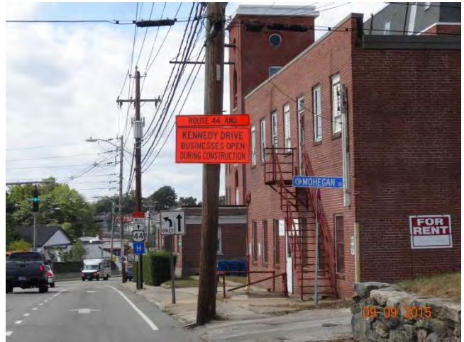
Providence Street (Route 171) NB: A construction sign posted on a utility pole states ROUTE 44 AND KENNEDY DRIVE BUSINESSES OPEN DURING CONSTRUCTION.
