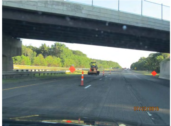
I-84 WB: OVERHEAD WIRES signs to warn truck drivers of the low wire when raising their truck beds.
