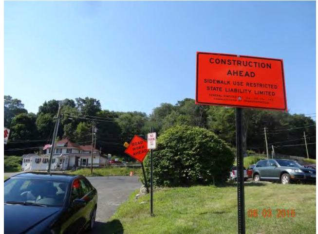
Rockdale Avenue: A post-mounted legal series sign and a post-mounted ROAD WORK AHEAD sign with a high-intensity warning light attached.
