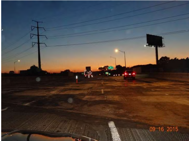
I-91 SB: The milled surface on the bridge. The reflectivity of the temporary pavement markings is poor.
