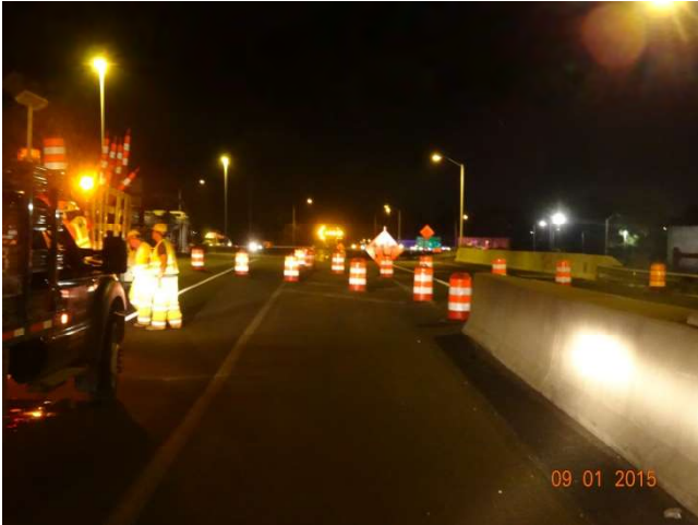
I-95 SB: Exit 45 on ramp is delineated with traffic drums to I-95 mainline and preventing motorists from taking the proceeding exit where barrier is going to be moved.
