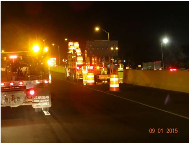
I-95 SB: A flashing arrow about to signal to merge left in the taper of the traffic pattern.
