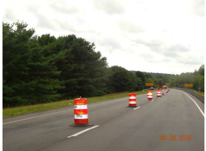
Route 11 SB: The taper of traffic drums transitioning into the lane closure using traffic cones. A TMA with a flashing arrow signaling lane closed is in the closed left lane.
