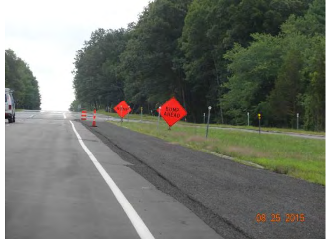
Route 11 SB: Temporary signs warning motorists of BUMP AHEAD and BUMP, respectively, as they transition from the newly paved section which is lower than the section with the existing pavement.
