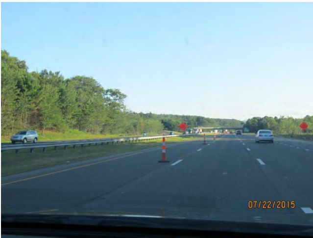
I-84 WB: Post-mounted advance warning signs on both sides of the highway and traffic cones along the work zone tangential.
