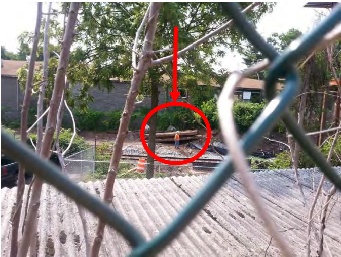
Burritt Street: The Pan-Am Railroad flagger notifying the workers to clear the rails.
