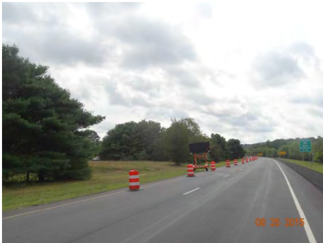
Route 11 SB: Approaching the third work zone in the left lane. The taper is comprised of traffic drums and there is a flashing arrow within. The flashing arrow is on but the lights are very dim due to the angle the board is tilted.
