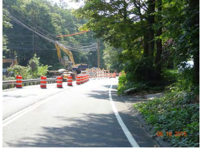
Route 57 SB: Approaching the work zone where traffic drums are closing the northbound side of Route 57.
