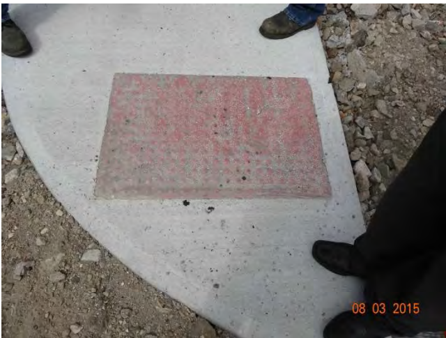
Route 73 NB: The detectable warning in the newly installed sidewalk. The width of the warning is too short. The requirement for detectable warning is a minimum of two feet in the direction of travel and the full width of the curb ramp.
