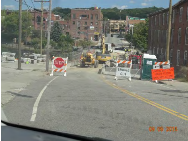
Pomfret Street (Route 44) EB: The road closure with use of Type III barricades. There is a STOP sign, BRIDGE OUT sign, and dated start to end.
