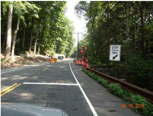
Route 53 NB: The stop bar with sign and red light on the temporary signal.
