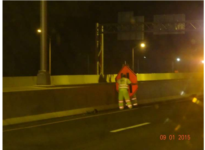
I-95 SB: A worker is installing a merge left sign on the left side of the highway. Since the sign is in a narrow shoulder, its sides are cut off to prevent motorists from hitting it and knocking it over.
