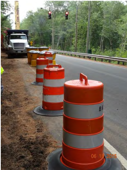
Route 79 SB: The traffic drums used for the taper leading up to the one-lane travel way.
