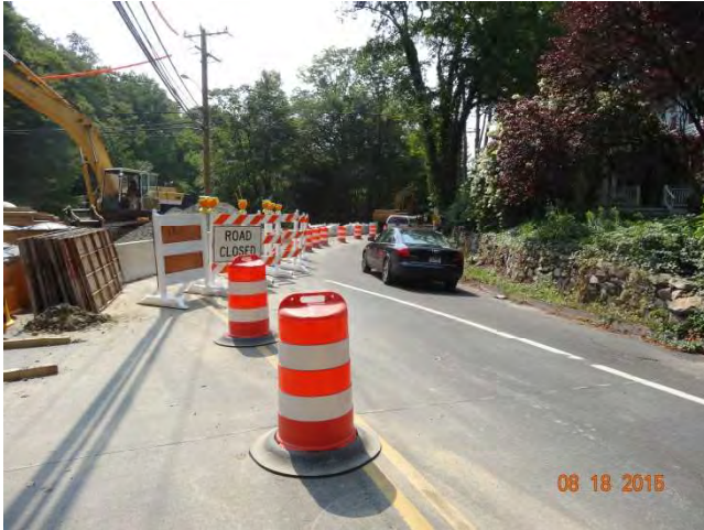
Route 57 SB: Motorists driving through the one-way portion of the detour around the project.
