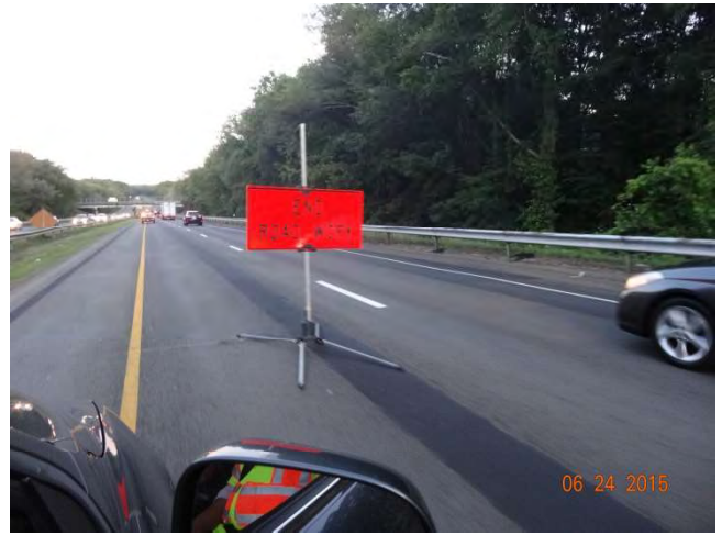
I-95 NB: "End Road Work" sign on top of patching in the high speed lane on the joint seam. The patching was done to prevent accidents especially for motorcyclists due to traffic shifts from the median work.
