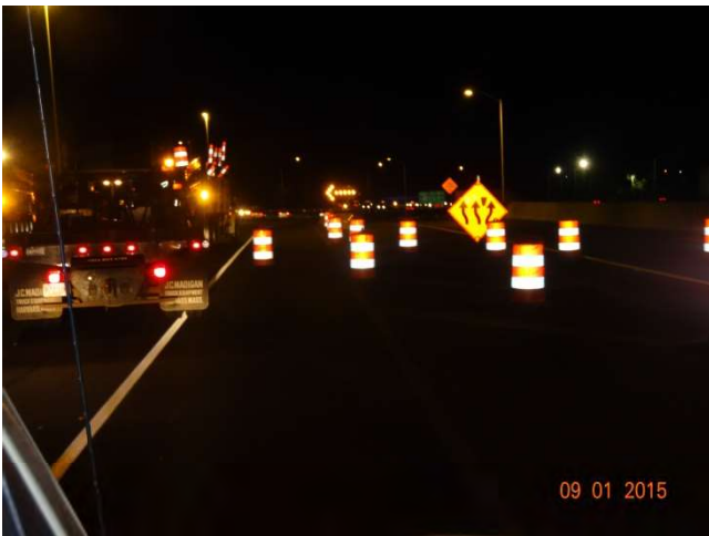
I-95 SB: A temporary traffic shift sign is installed and another portable flashing arrow signaling to merge left for oncoming traffic.
