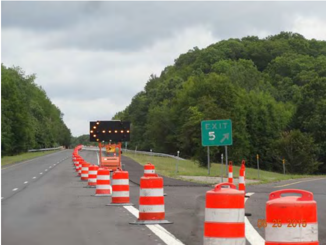
Route 11 NB: Approaching the fifth work zone with traffic drums starting the taper from Exit 5 gore area. A flashing arrow is signaling to merge left. However, on the Exit 5 off ramp the gore area is closed with traffic cones.
