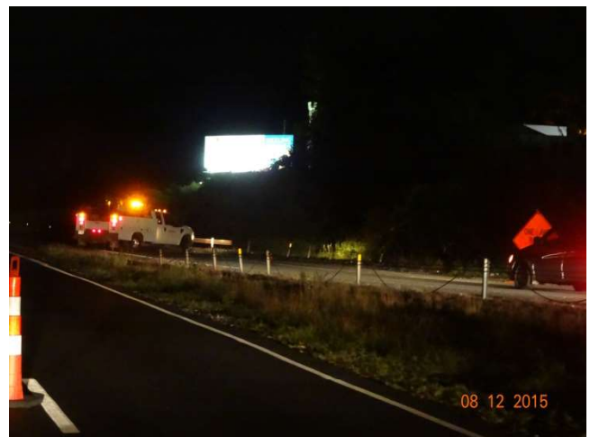
I-84 EB: The Contractor is using his work truck to temporarily stop traffic on the on ramp as the sign crew is setting up the pattern on the mainline.
