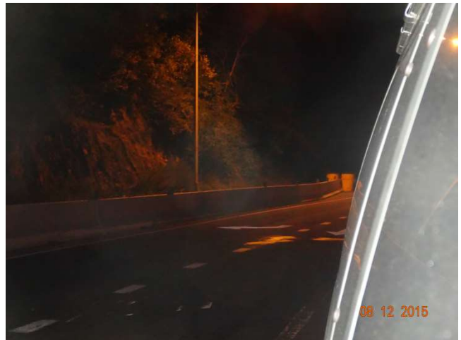
I-84 EB: A Type A Impact Attenuation System at the end of concrete barrier along the right side of Exit 23.
