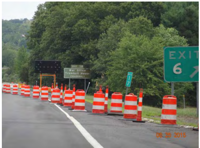
Route 11 NB: Approaching the sixth work zone starting at Exit 6. The taper is comprised of both traffic drums and traffic cones. The flashing arrow within is on and signaling to merge left but wasn't captured in the photo.
