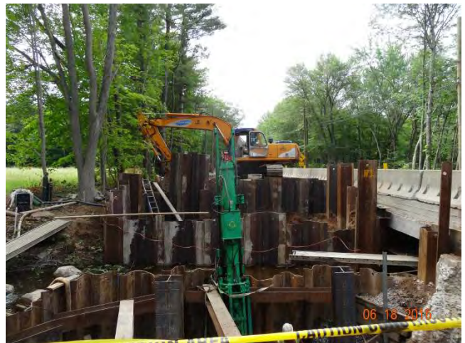
The work area where piles were being drive is behind the TPCB
