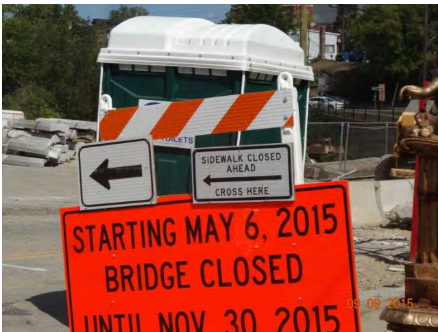
Pomfret Street (Route 44) EB: There is a SIDEWALK CLOSED AHEAD sign with arrows to notify pedestrians to cross the street to the temporary pedestrian walkway on the other side. There is a sign notifying all road users that the bridge will be closed from May 6, 2015 to November 30, 2015.
