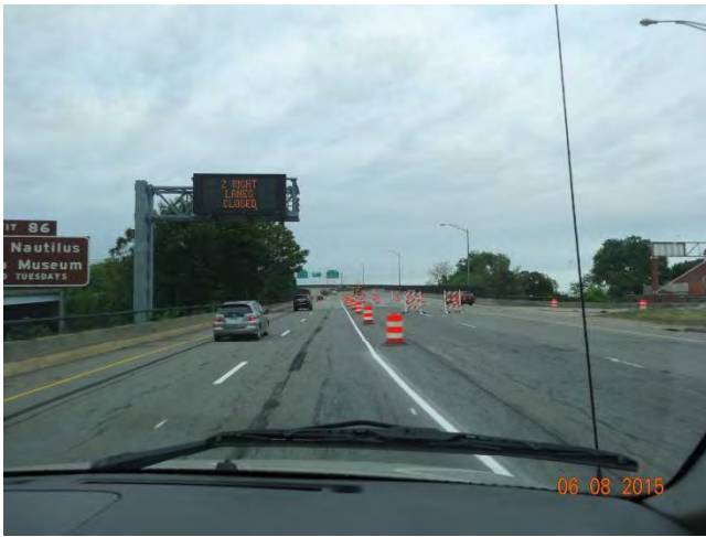
I-95 NB: Variable Message Sign (VMS) with a message stating the right two lanes are closed.
