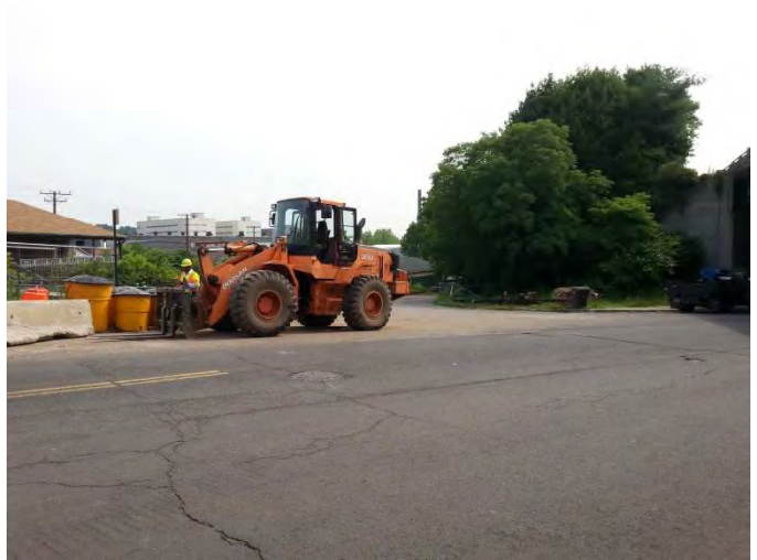
West Main Street: A pay loader parked in front of the attenuation system. When the inspection staff was told that it should be parked elsewhere to prevent a serious accident they said that it was temporarily there to move the barrier for the Contractor to get in and out of the work site.
