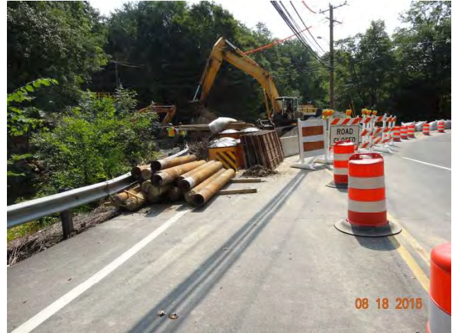
Route 57 SB: Materials stored in the northbound side of Route 57 behind the traffic drums. The materials should be stored in an area that is positively protected.
