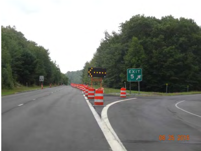
Route 11 SB: Approaching the second work zone with a lane closure starting at Exit 5. The taper is comprised of traffic drums and has a flashing arrow signaling to merge left.
