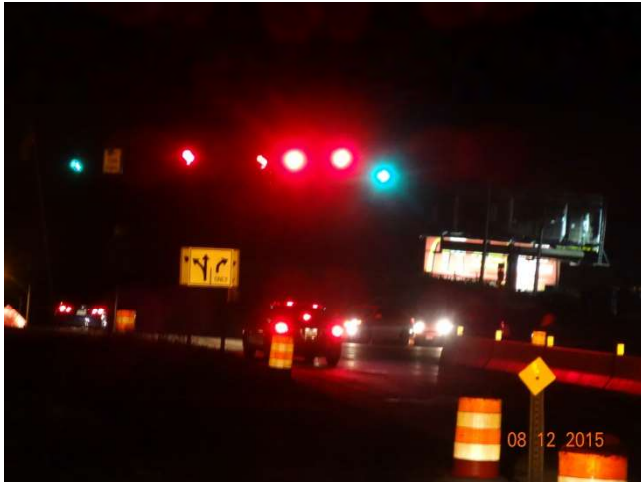
I-84 EB Exit 23: The traffic signal that has been modified temporarily for the traffic impacts from the construction on Hamilton Avenue.
