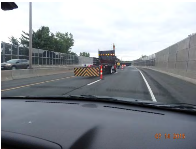
Route 15 NB: Truck-mounted attenuator protecting the work area with a flashing arrow signaling the lane is closed.
