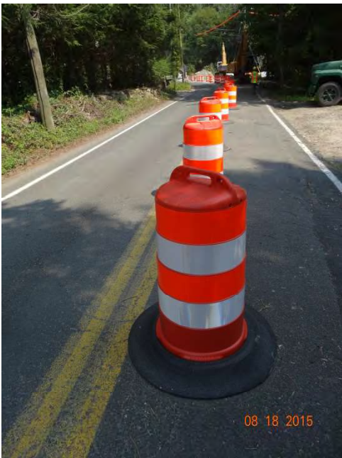
Old Mill Road NB: Traffic drums closing the northbound lane and guiding traffic in the southbound lane down Route 57.
