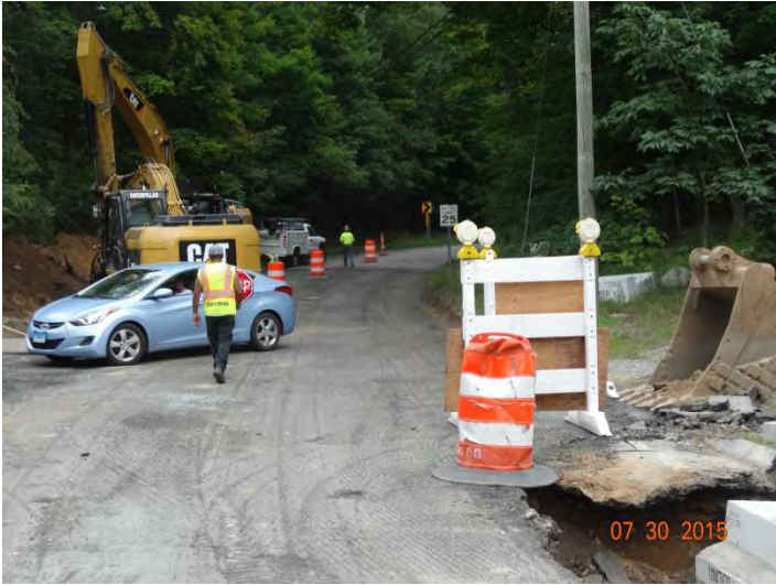
Route 148 EB: Two flaggers with safety gear and paddles to direct traffic around the closed lane on the bend the in the road on westbound side.
