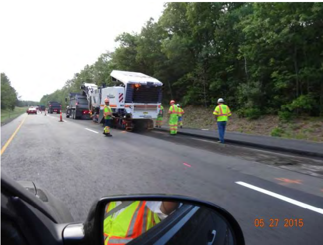
WB: The rubblizing crew working within the pattern; all the workers are wearing their Type III reflective gear
