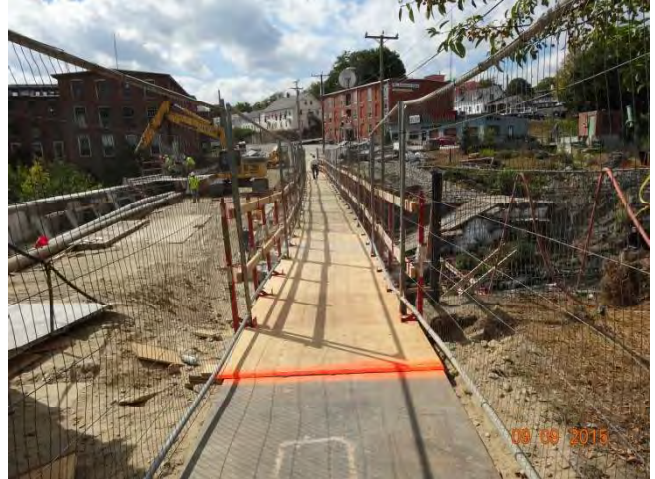
Pomfret Street (Route 44) WB: A pedestrian using the temporary pathway crossing over the work area.
