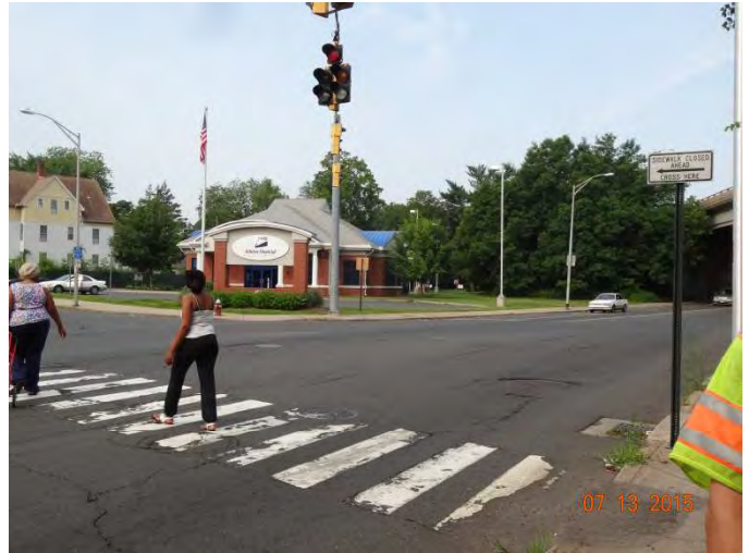
West Main Street EB: A Sidewalk Closed Ahead sign directing pedestrians to use the available crosswalk before proceeding through the work zone.
