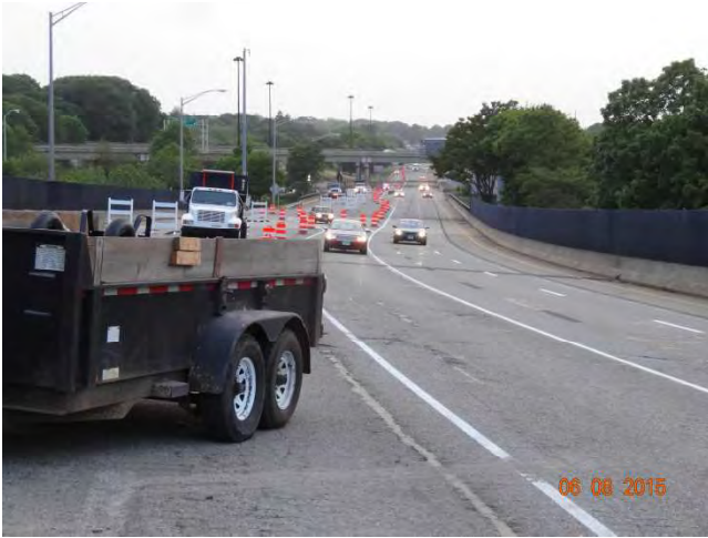
I-95 NB: The Contractor's work truck just before the work zone adjacent to travel lanes
