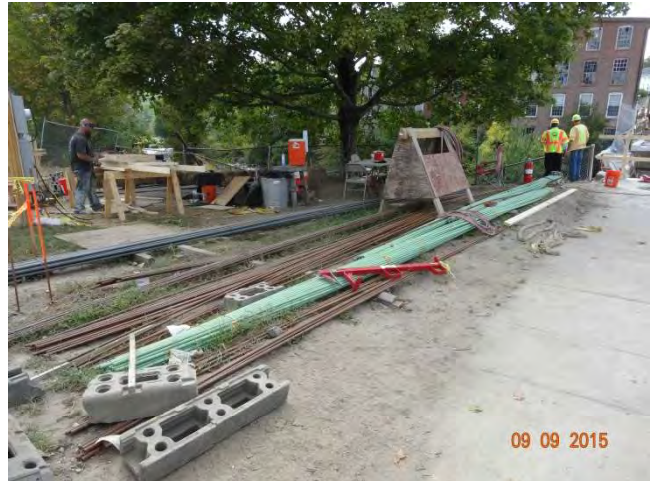
Pomfret Street (Route 44) WB: Material stored at the southeast corner of the project and a work table for the workers to craft forms.
