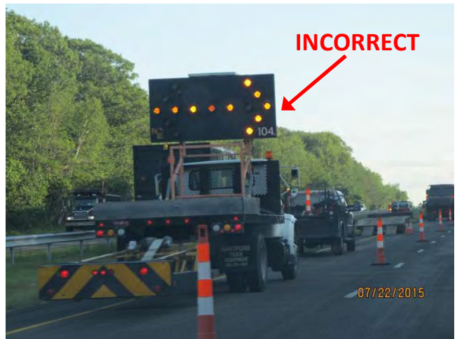
I-84 WB: The Truck-Mounted Attenuator with a flashing arrow incorrectly signaling to merge right. Since the truck is in a closed lane not a taper the arrow should have a straight bar to signal the lane is closed.
