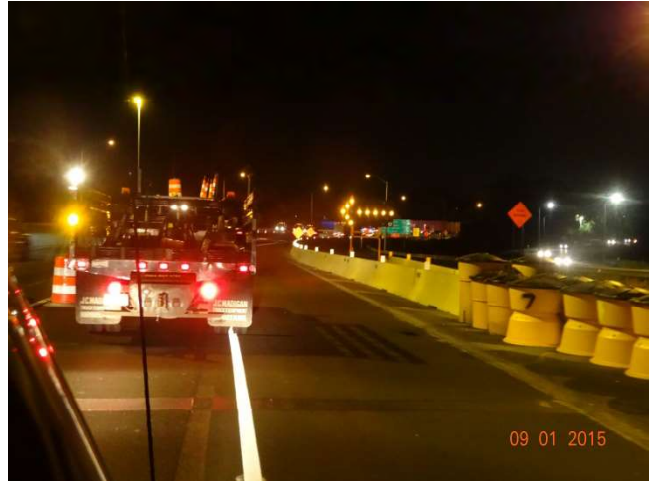
I-95 SB: Type A Impact Attenuation System in front of the TPCBC and a portable flashing arrow in the gore of the off ramp.
