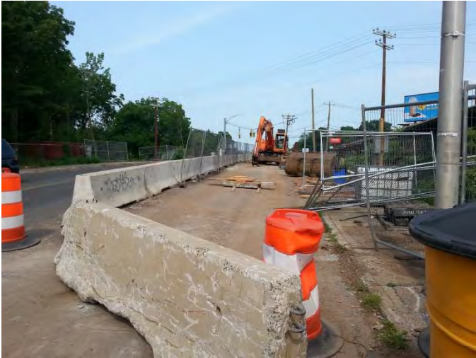
West Main Street EB: Project site on north side of the bridge behind barrier.
