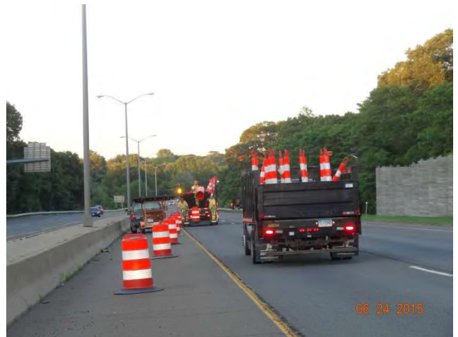
I-95 NB: Deployment of the traffic pattern. The taper extending out to close the high speed (left) lane.
