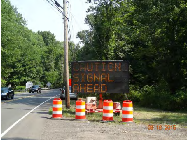
Route 53 NB: A Changeable Message sign with one frame notifying motorists CAUTION SIGNAL AHEAD. The CMS is only behind traffic drums but should be positively protected since it is a blunt end.
