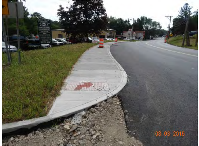
Route 73 SB: A new sidewalk with the detectable warning. There are traffic drums moved onto the sidewalk so the road could get paved.
