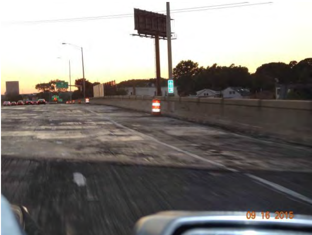
I-95 SB: This section of the road is the work site being repaired. The surface has been milled and temporary pavement markings placed but are faded. Traffic drums are lined up on the bridge parapet where work is being done.
