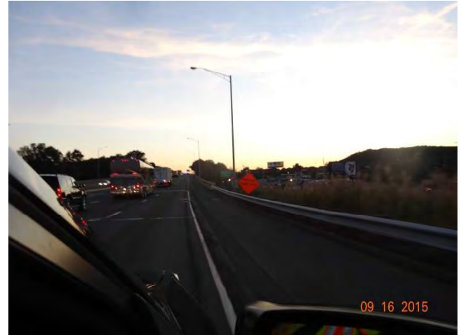
I-91 SB: A temporary construction sign behind the guiderail saying ROUGH SURFACE with a barricade warning light attached.
