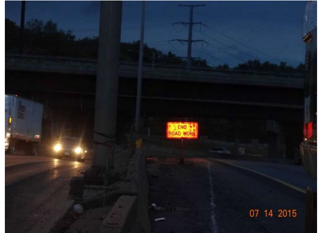
Route 15 NB: A temporary END ROAD WORK sign located just beyond the work area.
