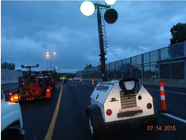
Route 15 NB: Illumination for the work area which is facing away from traffic.
