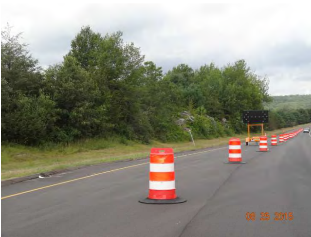
Route 11 NB: Approaching the fourth work zone with a taper of traffic drums. An advance flashing arrow in the taper is not on.
