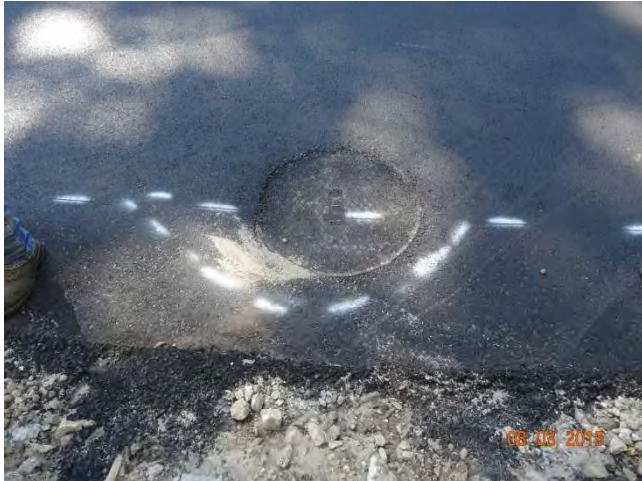
Route 73 NB: The mark out curved around the manhole to ensure that the bituminous curb is placed behind the structure and not over it.
