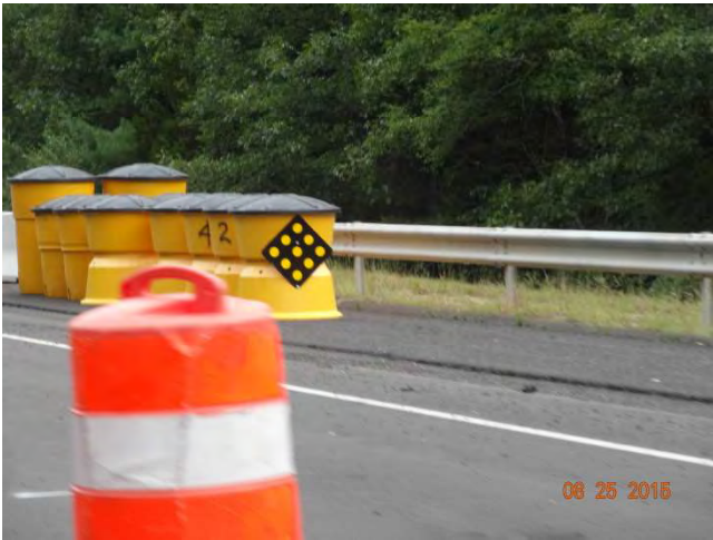
Route 11 NB: A Type A Impact Attenuation System with a DE-9 delineator on front protecting the end of the TPCBC used to close the right lane.
