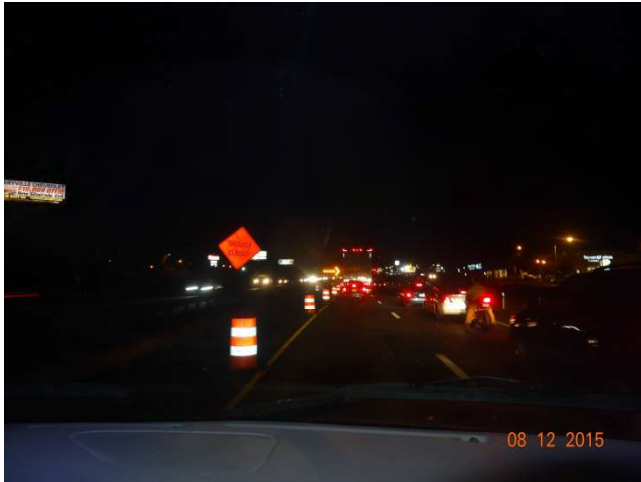
I-84 EB: Traffic merging right when approaching the traffic pattern. A construction sign saying SHOULDER CLOSED and traffic drums for the taper.
