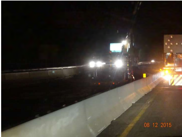
I-84 EB: The work crew working in the median with an excavator.
