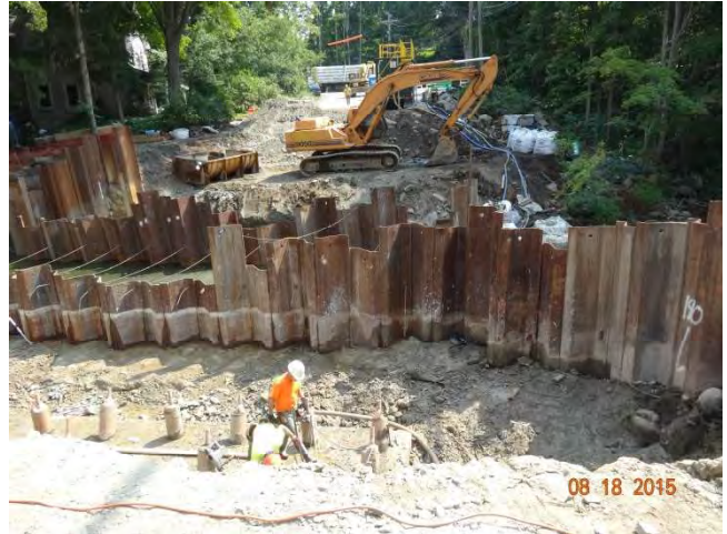
Route 57 NB: The work area with sheet piling installed and the work crew working on the southbound side of Route 57.
