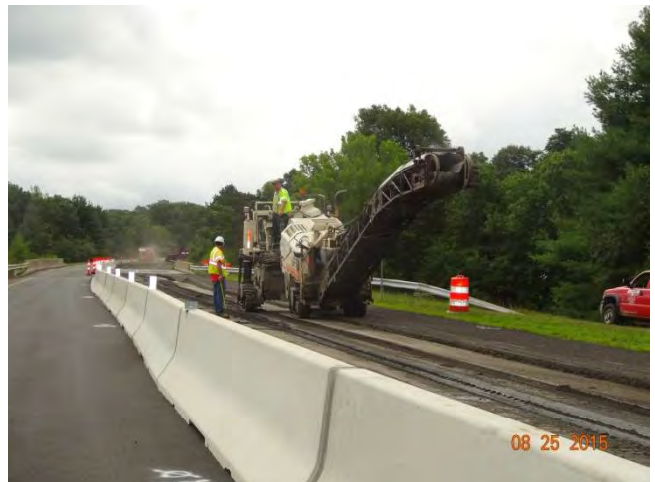
Route 11 SB: The Contractor's work crew milling the roadway adjacent to a bridge.
