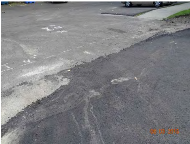
Route 73 NB: Asphalt that was temporary placed in an adjacent driveway to Route 73 to make a transition from the higher roadway to lower lot. The mark out is where the Contractor will sawcut and take out the existing pavement and replace with new pavement.
