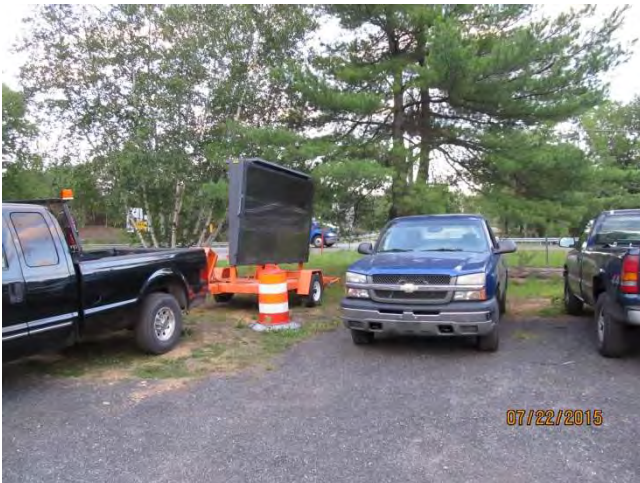
The other Changeable Message Sign for the eastbound side stored in the Contractor's laydown yard.
