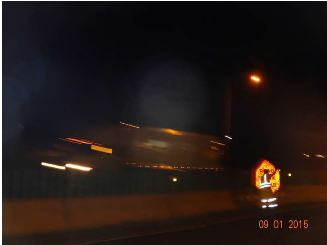
I-95 SB: A worker installing a ROAD WORK AHEAD sign in the narrow left shoulder with the edges cut off to avoid the sign being hit by motorists.
