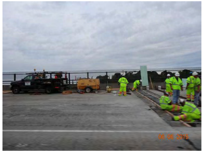
I-95 NB: Work area where bridge joints are being repaired; two right lanes are taken; workers are sitting or bending over to do the work
