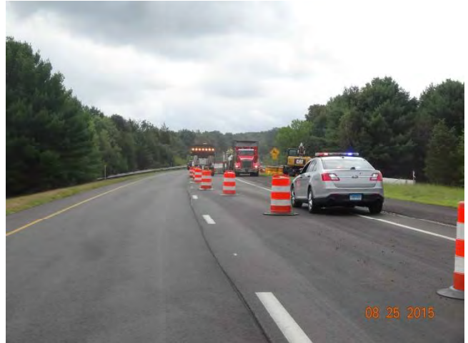
Route 11 SB: State Police within the taper and a truck-mounted attenuation system in the closed right lane. The flashing arrow on the TMA is signaling a bar meaning lane closed.
