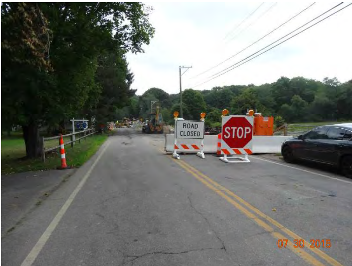
Route 148 EB: Another concrete barrier closing the road with Type III barricades in front with ROAD CLOSED and STOP signs on them.
