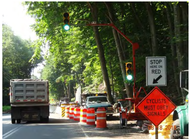
Route 53 SB: The green light of the temporary signal.
