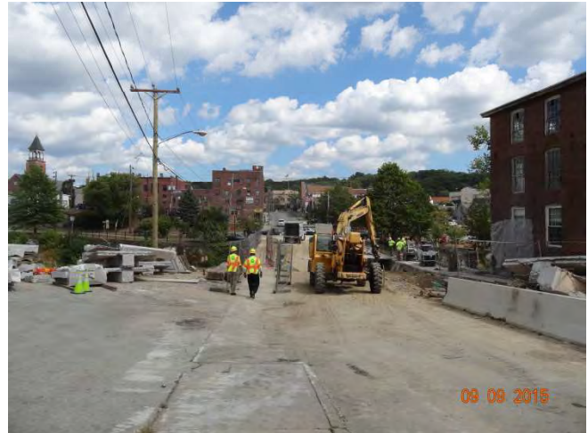
Pomfret Street (Route 44) EB: The temporary pathway built over the work area allowing pedestrians to still use Route 44. To the left,, material is stored in the parking lot of the local radio station.
