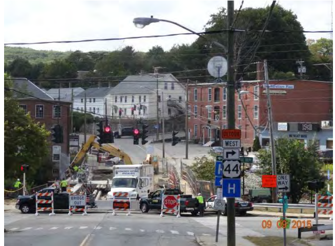
School Street (Route 44/12) WB: The bridge closure from the west side. Detour signs posted to route traffic down Bridge Street.
