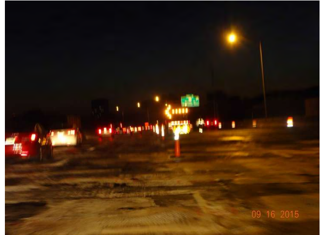
I-91 SB: The other flashing arrow is mounted on a Truck-Mounted Attenuator in the closed lane. It is signaling for motorists to merge left but since it is in the closed lane it should signal lane closed using a straight bar.
