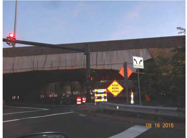
Ferry Street: At the intersection with Middletown Avenue is the work zone beneath I-91. A temporary ROAD WORK AHEAD sign with a barricade warning light next to a height clearance sign which is blocked by a pole from this view. There is a Type III barricade closing the sidewalk with a SIDEWALK CLOSED, CROSS HERE sign pointing to the crosswalk. Along the street are traffic cones and traffic drums. Although it is dark, there is a bicyclist riding past the work zone.
