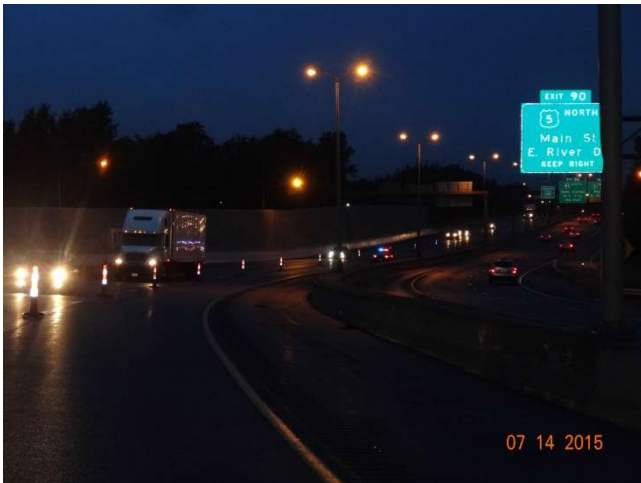
Route 15 NB: The State Police Officer in the closed lane with lights flashing to advise motorists of the work area ahead.
