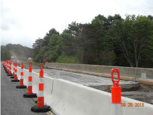
Route 11 SB: The bridge structure behind Temporary Precast Concrete Barrier Curb (TPCBC) and traffic cones along the curb.
