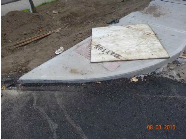
Route 73 NB: Plywood covering a detectable warning pad. This poses as another unnecessary trip hazard.
