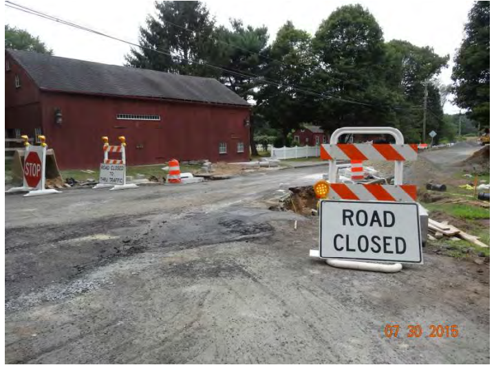
Route 148 WB: Barricades indicating the road is closed. Signs with high-intensity warning lights on them saying ROAD CLOSED or STOP.
