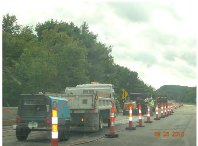
Route 11 SB: The work crew doing bridge repairs within the closed lane.
