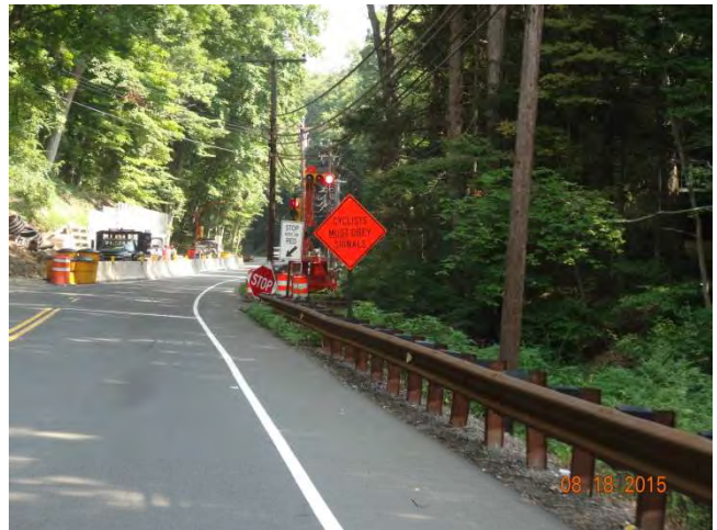
Route 53 NB: Approaching the work zone which has an alternating one-way traffic pattern with a temporary signal.
