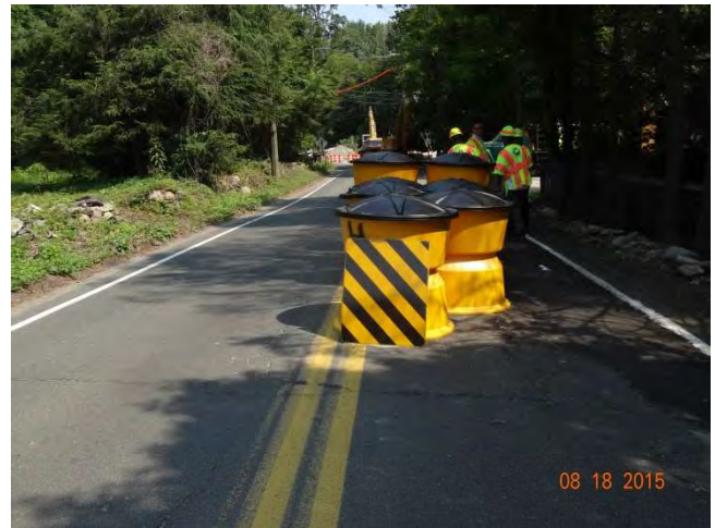
Old Mill Road NB: An impact attenuation system with a chevron sign on front in the northbound side just beyond the barricades.
