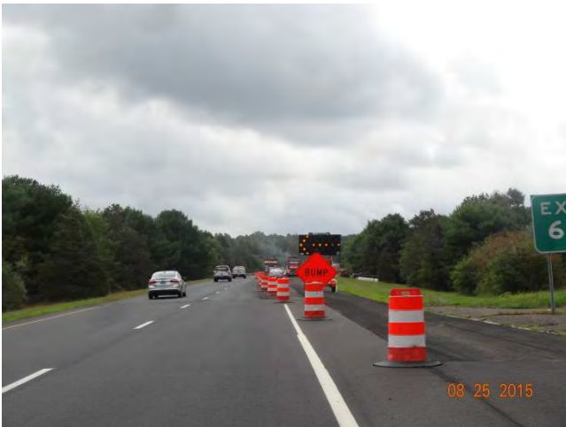
Route 11 SB: Approaching the first work zone starting at Exit 6. The taper is comprised of traffic drums. A temporary BUMP sign and an advance flashing arrow are in the taper.
