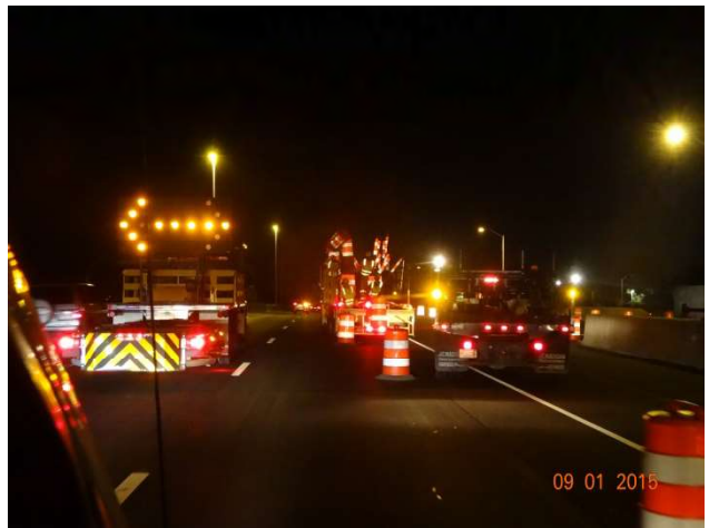
I-95 SB: The left lane is opened for motorists to proceed through.
