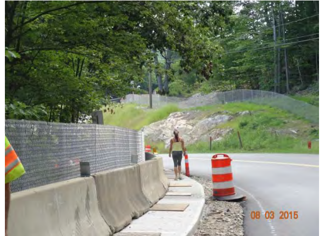
Route 73 SB: A pedestrian using the sidewalk and walking over the wood boards.
