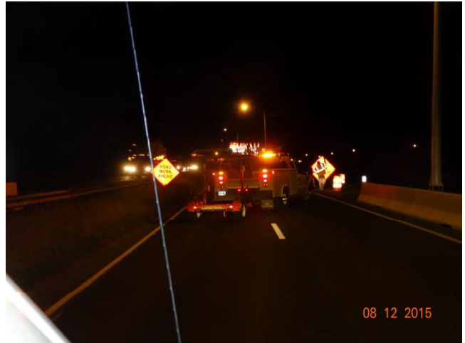
I-84 EB: ROAD WORK AHEAD signs installed on both sides of the road.
