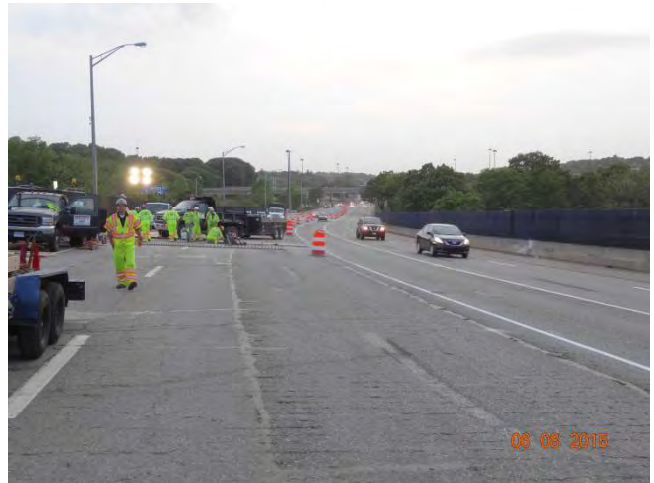
I-95 NB: Facing south at work zone; traffic drums are the only protection against the traffic
