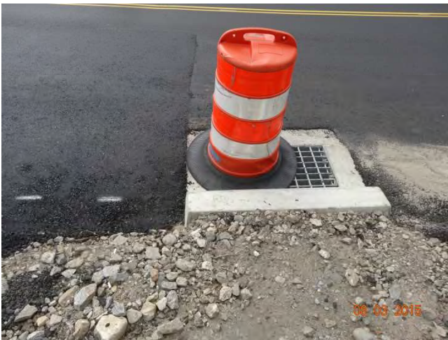
Route 73 NB: A traffic drum over a catch basin to inform motorists of structure when it was raised higher than the roadway before paving.
