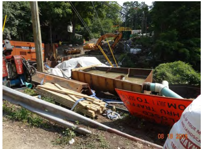
Route 57 NB: The dewatering system and material stored adjacent to the project.
