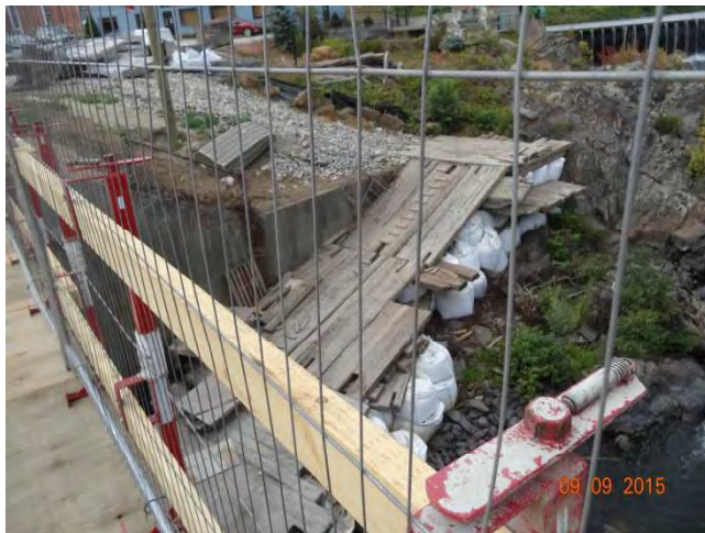
Pomfret Street (Route 44) EB: The Contractor built a temporary walkway for workers to access the work surface below on the north side of the bridge.
