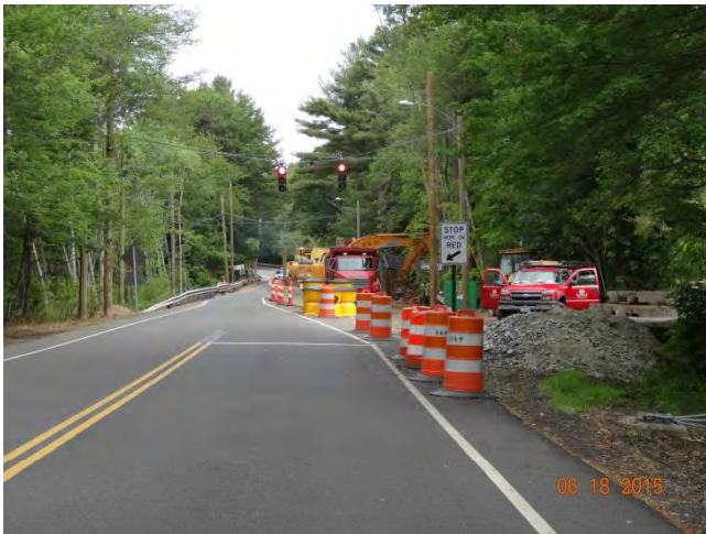
Route 79 NB: The hard-wired temporary signal and the stop bar and post-mounted stop bar sign
