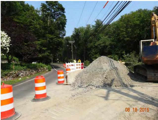
Route 57 NB: A pile of gravel next to an excavator behind a concrete barrier curb in the closed northbound lane.
