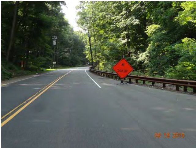
Route 53 SB: A temporary NO SHOULDER sign. The project staff stated that if there are pedestrians on the route they would use the shoulder. The work zone causes the shoulder to be closed.
