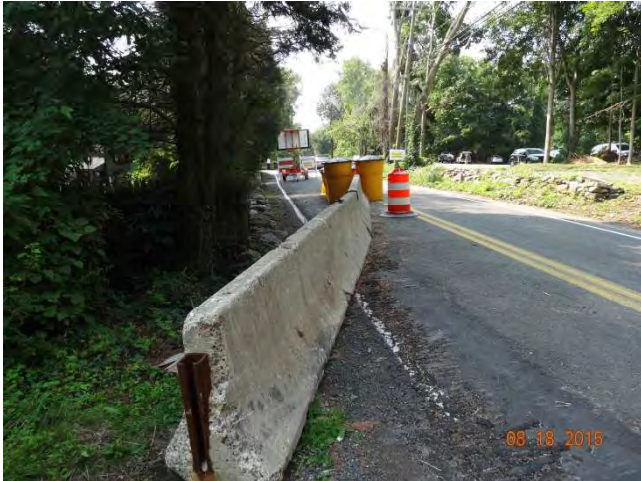
Old Mill Road SB: A concrete barrier curb in the northbound lane with end protected by impact attenuation system.
