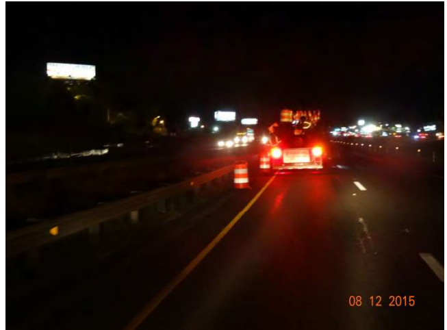
I-84 EB: The work crew setting up traffic drums for the taper of the traffic pattern.
