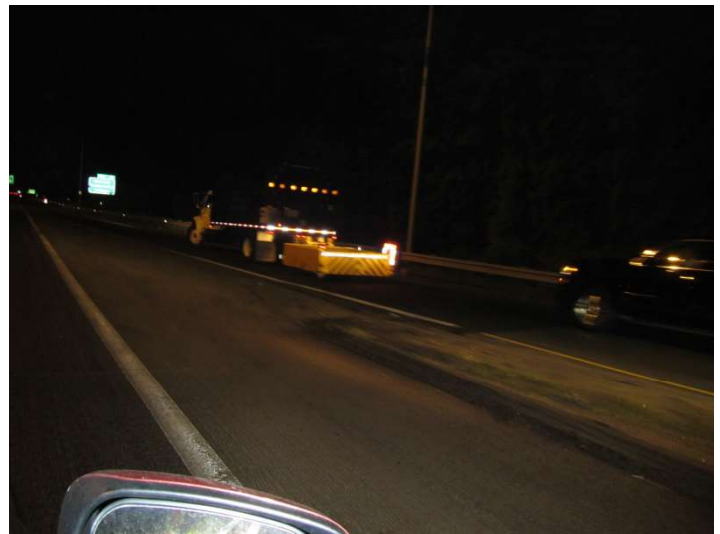
I-95 NB: An truck-mounted impact attenuator with a flashing arrow at Exit 12 on ramp.
