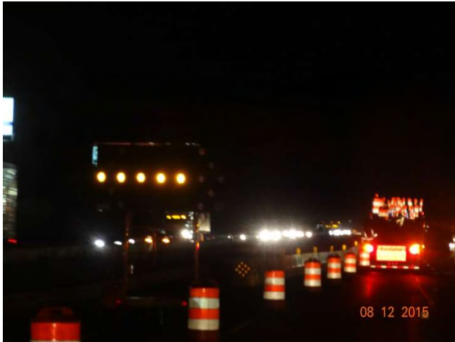
I-84 EB: An advance flashing arrow signaling to merge right (right arrow wasn't captured in photo) within the taper. Also another Type A impact attenuation system on the blunt end of the concrete barrier just beyond the arrow.
