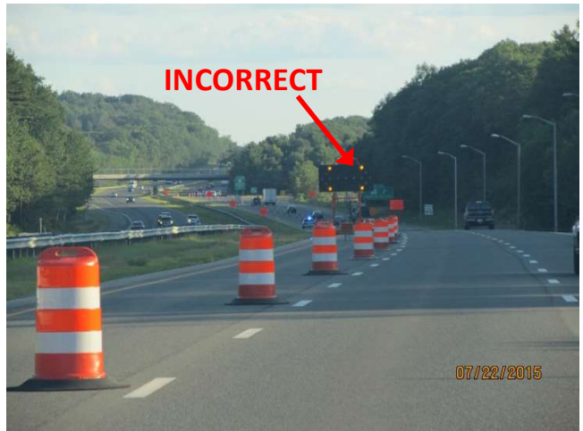
I-84 WB: Another portable flashing arrow placed within the closed lane incorrectly signaling that the shoulder is closed instead of having a straight bar to signal that the lane is closed.
