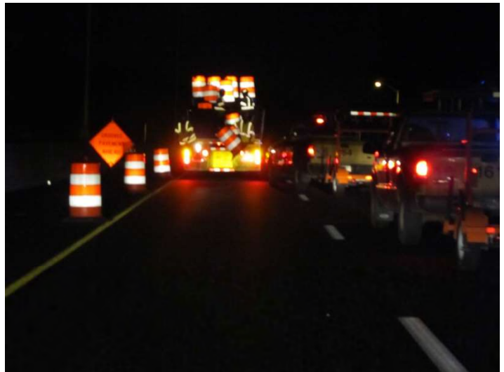
I-95 NB: The work crew is placing the traffic drums for the traffic pattern taper.
