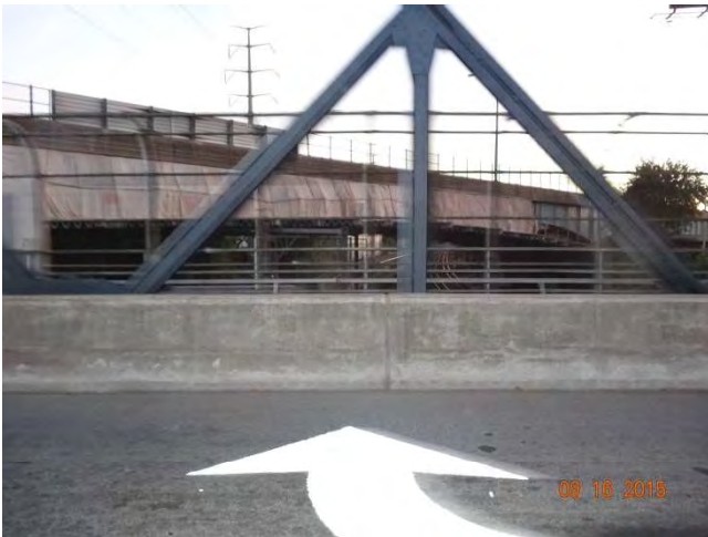
Ferry Street: The bridge that carries I-91 over Amtrak railroad. There is debris shield over the bridge to protect the travel ways below.
