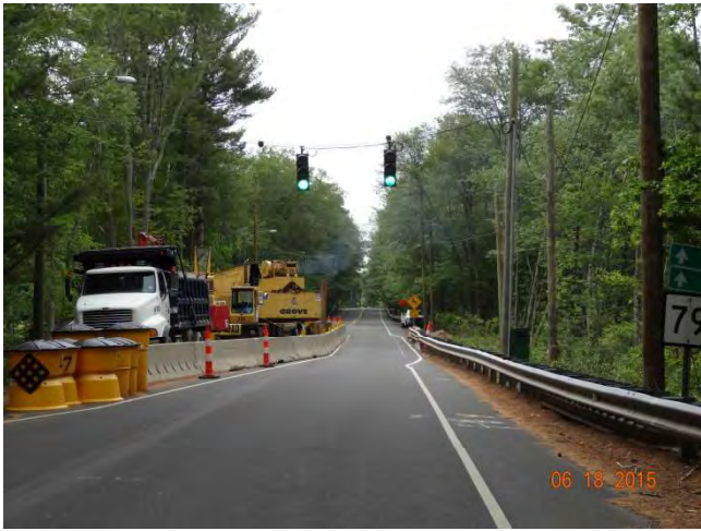
Route 79 SB: The temporary signal that the Contractor installed and hard wired.
