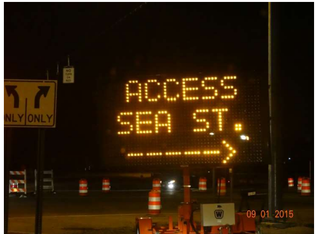
Ella Grasso Boulevard: A CMS at the end of the Exit 44 off ramp advising motorists how to access Sea Street which now has limited access during construction. Behind the CMS the intersection has a number of traffic drums and barricades blocking access to the street from the ramp.
