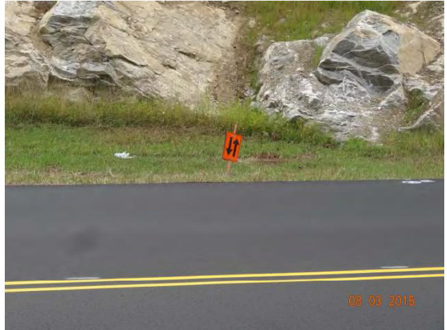
Route 73 NB: A temporary lane divider moved to the side of the road so it could be paved.
