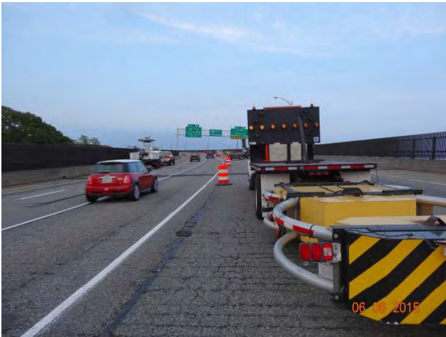
I-95 NB: Facing north towards the work zone behind crash truck placed at the end of on ramp
