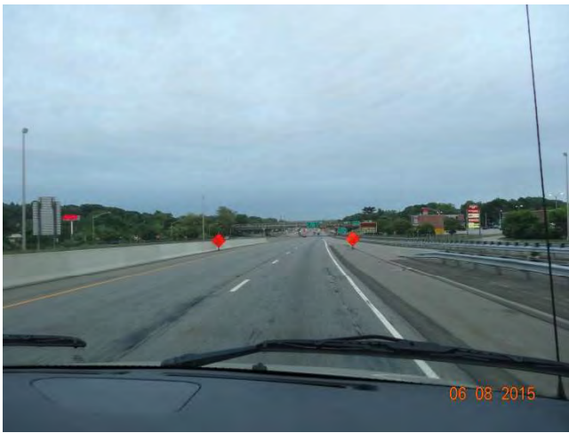
I-95 NB: Advance warning signs on both sides of the road saying "Right Lane Closed Ahead"
