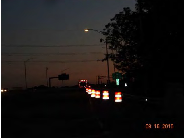
I-91 SB: The work crew starting to set up the taper using traffic drums. The taper starts just after motorists come on to I-91 from Exit 8.
