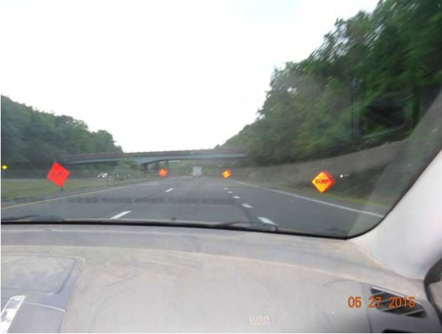
Westbound (WB): Signs are set up on both sides of the road
