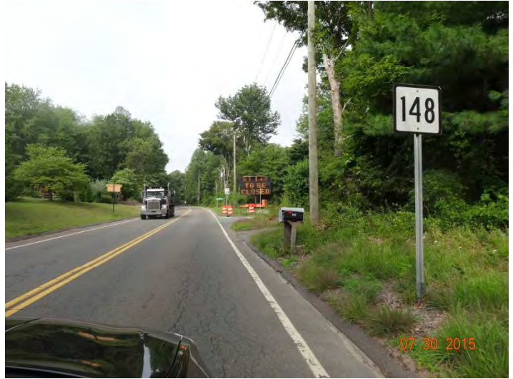
Route 148 WB: A Changeable Message Sign with the first frame saying RT 148 TO BE CLOSED. The CMS is not 30 feet off the travel way and is behind traffic drums which aren't adequate protection.
