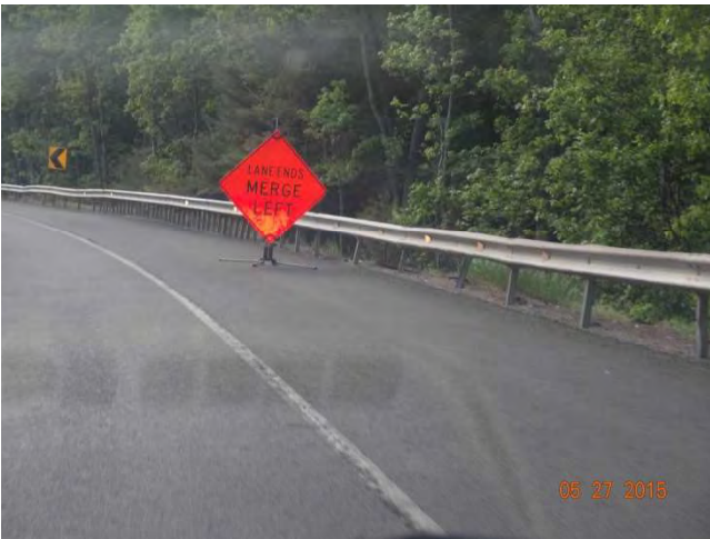
WB: The condition of the signs being used is acceptable
