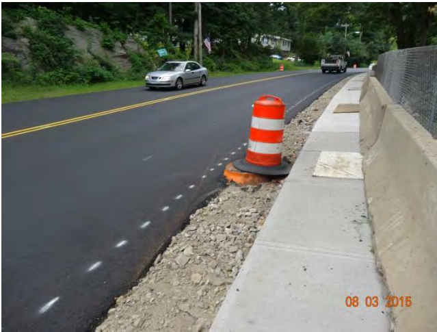
Route 73 NB: A traffic drum on a raised manhole and the mark out on the road where the bituminous concrete curb will be installed.
