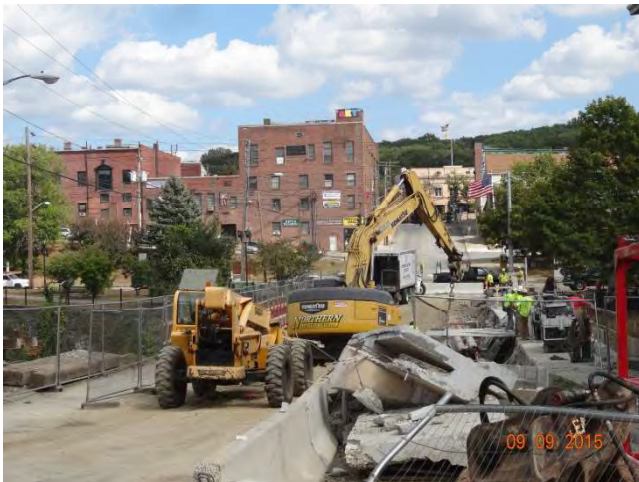
Pomfret Street (Route 44) EB: The construction site where the bridge over the Quinebaug River is closed.
