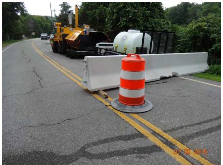
Route 148 EB: Concrete barrier propped on wooden posts.
