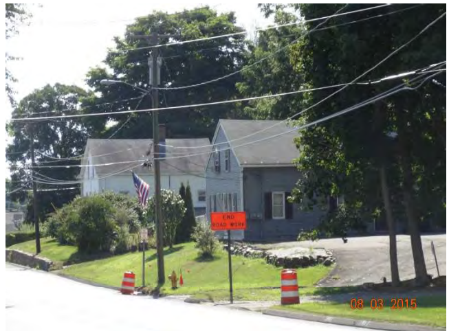
Route 73 SB: A post-mounted END ROAD WORK sign at the south end of the project.
