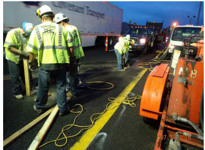
Route 15 NB: The work crew working next to live traffic. They are building a shield to block any concrete chips that may propel into the live traffic lanes.
