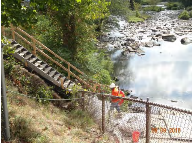
Pomfret Street (Route 44) WB: A temporary stairway built for workers to access the area beneath the south side of the bridge.
