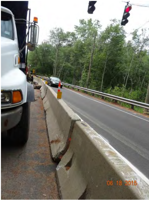
Route 79 SB: Within the work zone behind the Temporary Precast Concrete Barrier (TPBC) with the delineators attached on top. The yellow side of the delineator facing the southbound traffic is correct to be on the motorists' left side. A car is seen coming through the one-lane travel way after being signaled to do so.
