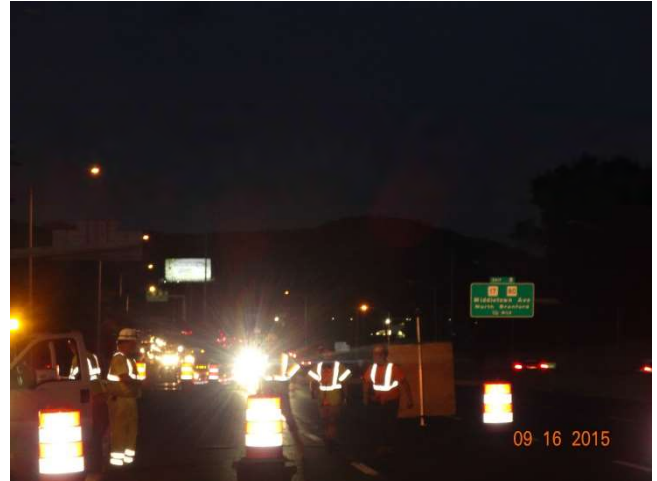
I-91 SB: Beyond the work crew setting up the pattern is the traffic queue from the rolling road block.
