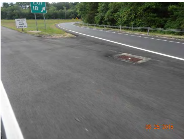
Route 11 SB: A temporary fines doubled sign.
