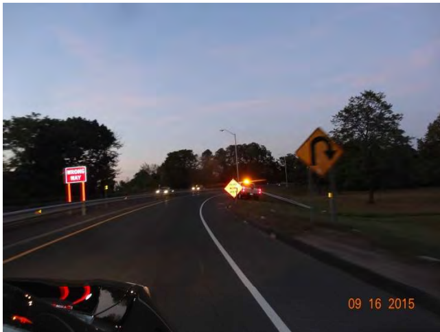
I-91 SB Exit 8 On Ramp: A temporary ROAD WORK AHEAD sign. Behind it is the Contractor's work truck parked behind the curb.
