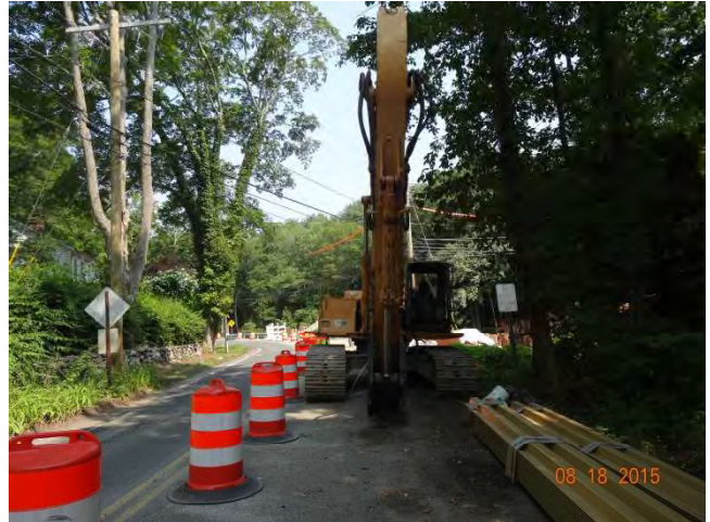
Old Mill Road NB: Fiberglass bracing and an excavator within the closed northbound lane.
