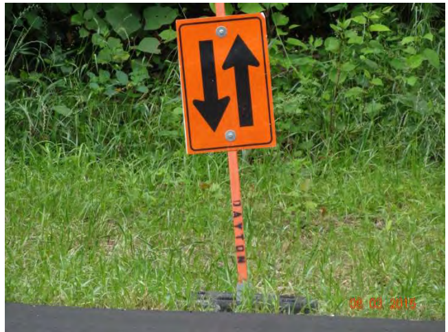
Route 73 NB: The lane divider to advise motorists of two-way traffic on the road before paving and line striping was done.
