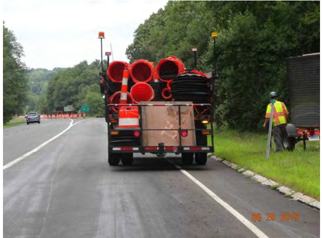
Route 11 NB: A worker from the sign pattern crew turning the CMS to face traffic and turning the device on.
