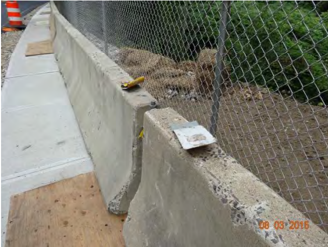
Route 73 NB: The delineators on the concrete barrier were in poor condition. They were bent over and misshapened. Some were facing the wrong direction or didn't have the second color on the opposite side.
