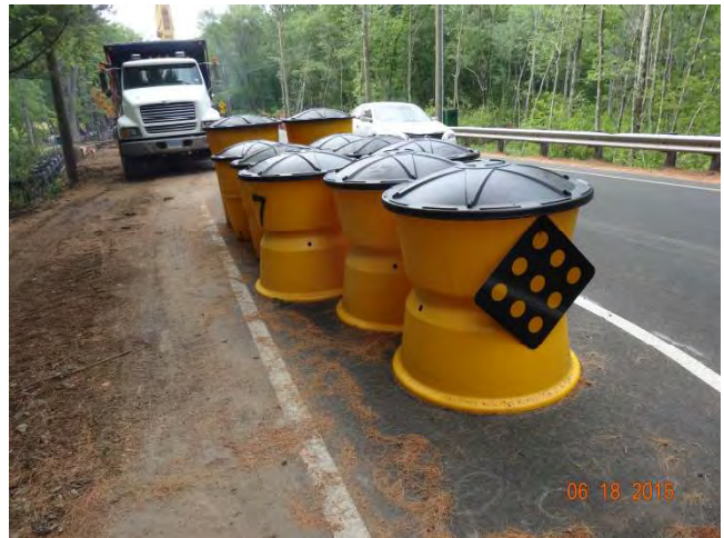
Route 79 SB: The Type I Attenuation System with the DE-9 delineator in front
