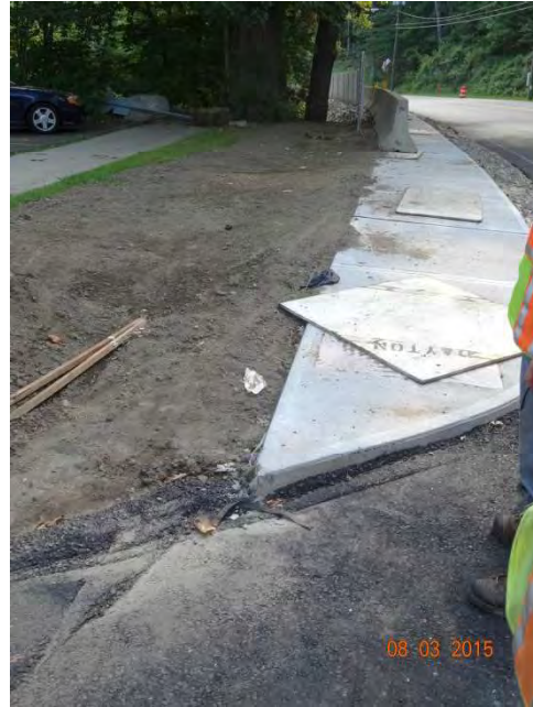
Route 73 SB: The sidewalk curb lip is higher than the half inch requirement from the roadway. Although this is a new sidewalk on the route, it still needs to meet ADA requirements during construction not just at the finished state.
