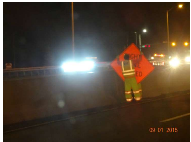
I-95 SB: Another RIGHT LANE CLOSED sign being installed but on the left side of the road.
