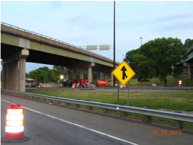
I-95 NB: Laydown yard underneath Williams Street Bridge where material and equipment are stored
