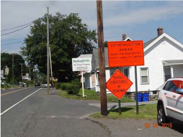
Route 73 NB: A post-mounted legal series sign and a RAISED STRUCTURES IN ROADWAY at the south end of the project.
