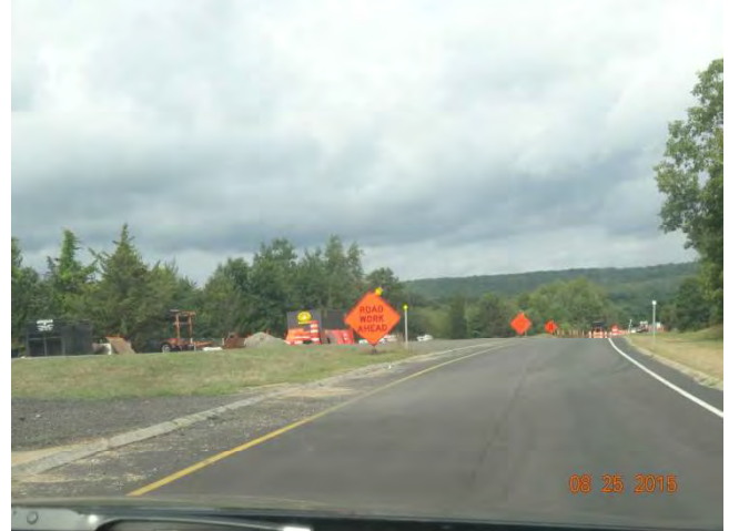
Route 11 NB: The laydown yard for the materials and equipment on the left. In front of it is a temporary ROAD WORK AHEAD sign with a high-intensity barricade warning light.
