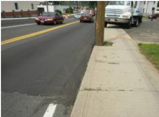
Utility pole at edge of road could benefit from additional delineation.
