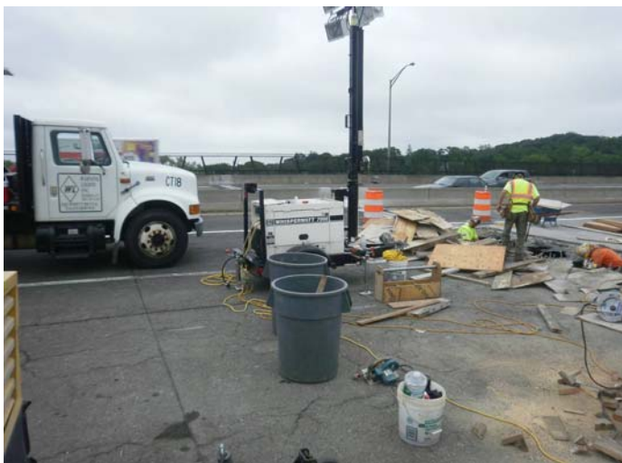
Figure 7: Cluttered Work Area
