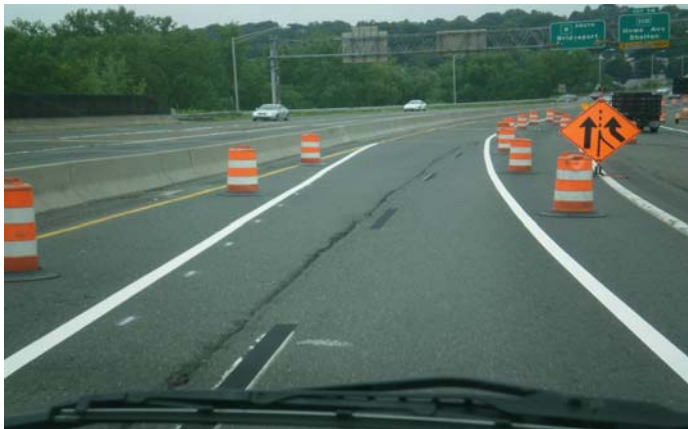
Figure 6: Improper Tape Color
