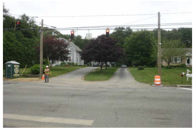
Temporary signalization for driveways
