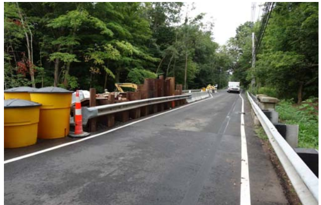
Plan details note the height of temporary earth retaining system shall not extend above the height of the TPCBC.
