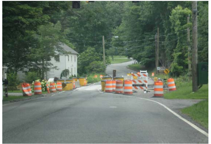
Type III Barricade with chevrons in wrong direction. Traffic Drum blocking DE-9.
