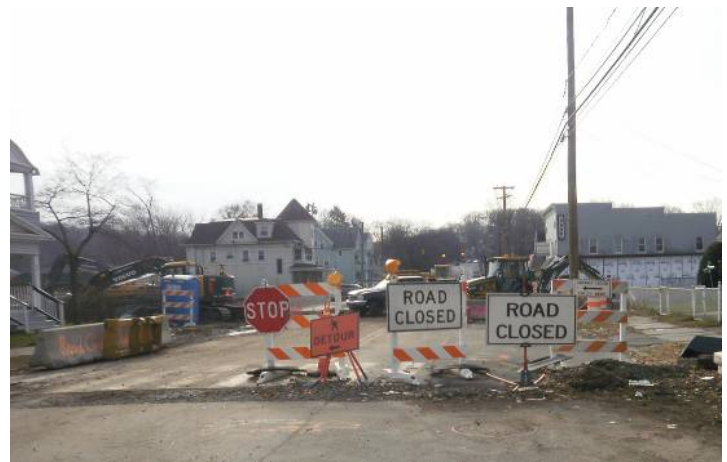
Sign No. 80-9929 to inform the public of the bridge closure. In accordance with Note 9 on the plans, this sign should have been removed once the detour was in effect.
