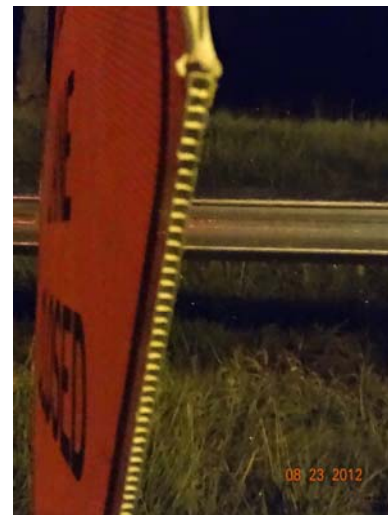
Appears to be waffle board substrate. Poor Retroreflectivity.
