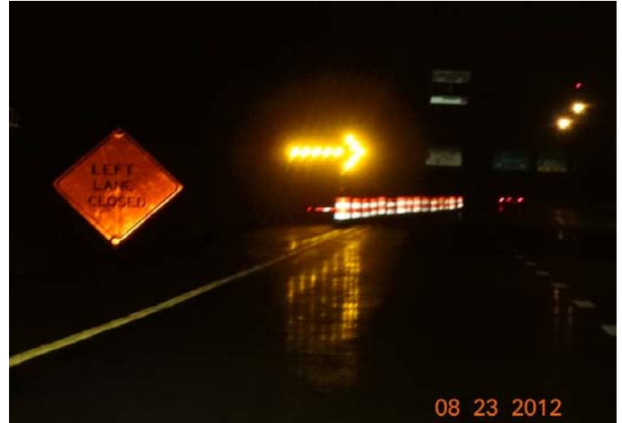
Sign too close to lane closure.
