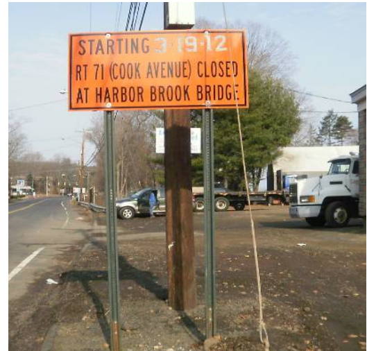
Sign pattern for the road closure at north end of bridge. Barricades were moved to allow for construction equipment access. Barricade stripes should all be sloping downward to the left.
