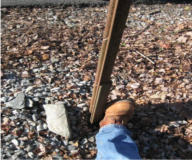
Improper breakaway post height.
