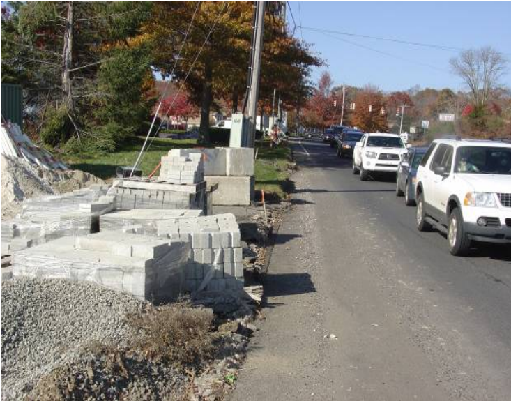
Material too close to Roadway
