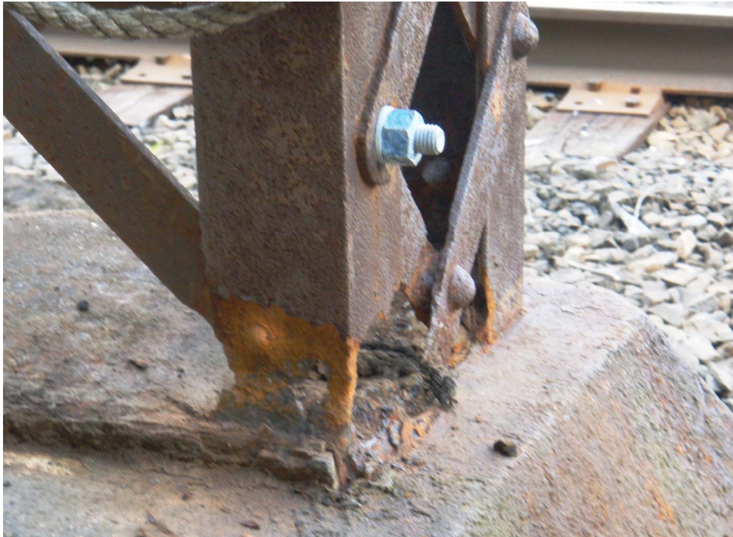
Catenary foundation base with severe deterioration of structural steel.
