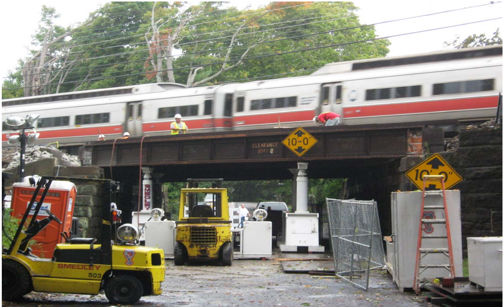
Setting up of the four hydraulic jacks leading up to the removal of first of two tracks.
