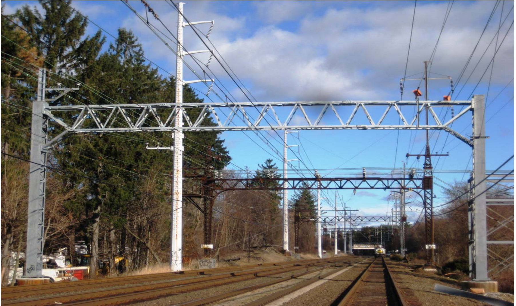
New catenary Truss type portal
