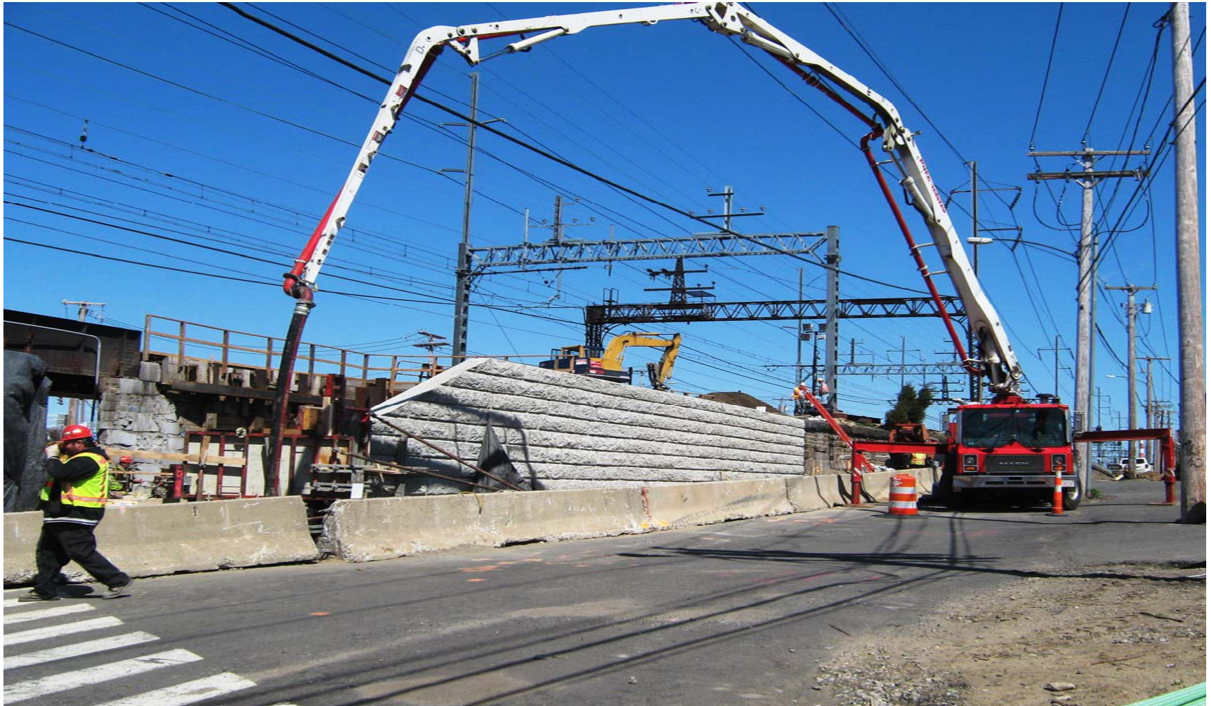
Use of a Crane-Concrete Pumper Truck to place concrete for the new abutment foundations.
