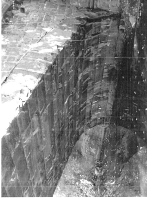
Photo # 14: East end of span 1: Areas of heavy efflorescence and areas of water leakage through the arch intrados.
