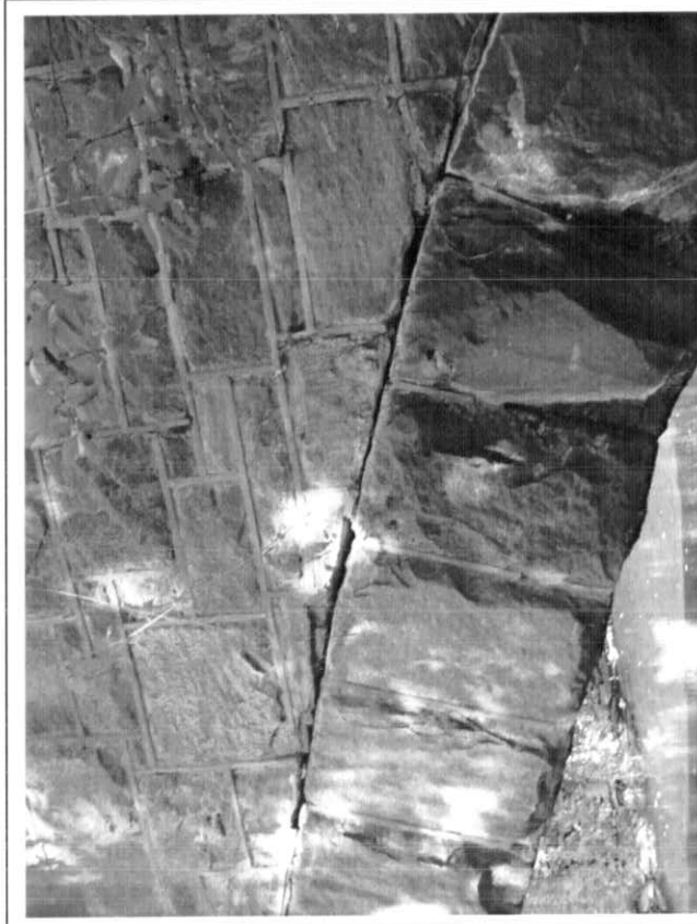
Photo # 16: Span 1, south elevation, east end: Deteriorated mortar between the arch ring stones and the spandrel wall.
