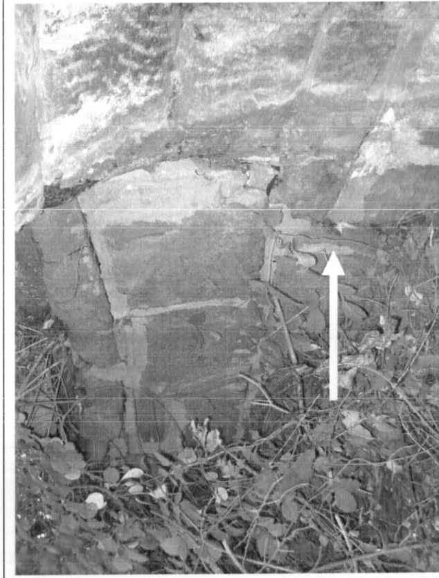
Photo # 19: Northeast wingwall: Stones shifted out at the base.
