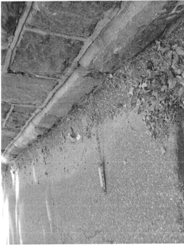
Photo # 10: Bridge overlay ramps up approximately 3" near the base of the north parapet.
