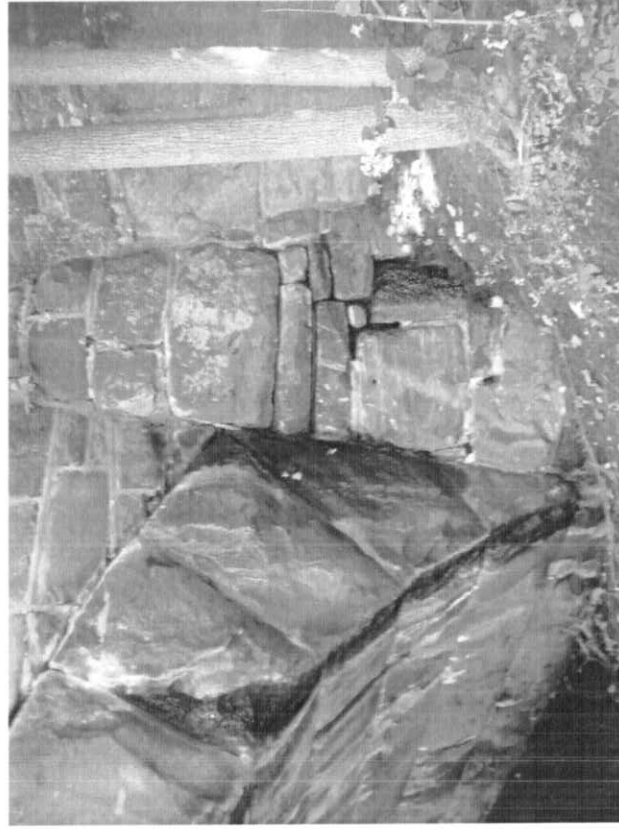
Photo # 18: Span 1, southeast corner: Architectural stone treatment at the corner of the span has deteriorated mortar/voids between the stones. Also note the leakage through the arch ring.
