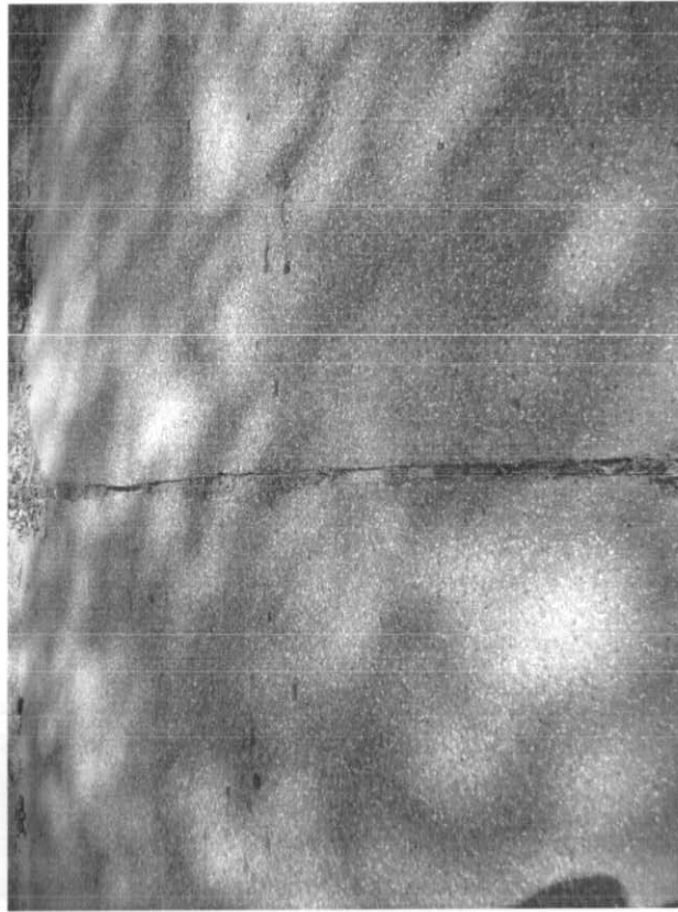
Photo # 11: Typical sawcut in the bridge overlay. Note that there is no sealant. Sawcuts are filled with dirt and have random vegetation.
