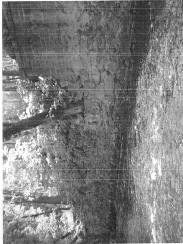
Photo # 21: Southwest retaining wall: Shifted stones and tree growing out of the wall.
