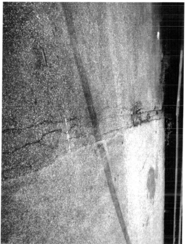
Photo # 9: TRANSVERSE CRACKS AT EAST DECK END.
