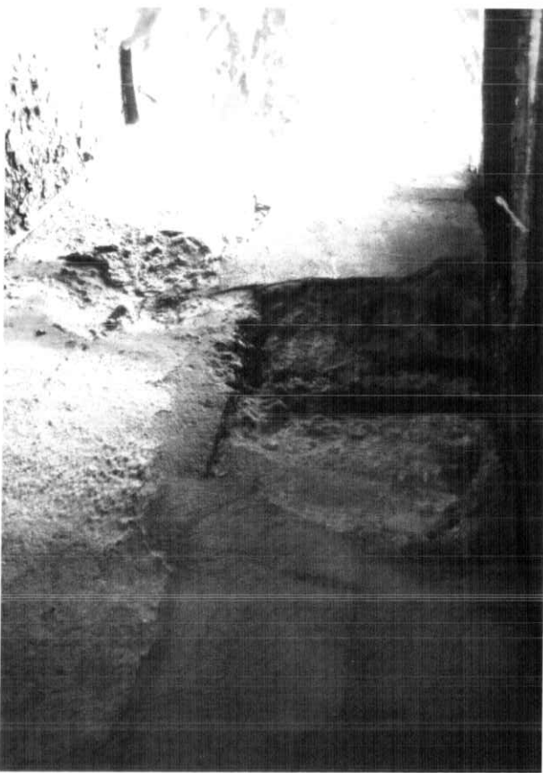
Photo # 23: EAST FACE OF PIER WITH A 30 IN. X 15 IN. X 4 1/2 D. SPALL WITH EXPOSED REBAR UNDER BEARING # 8.
