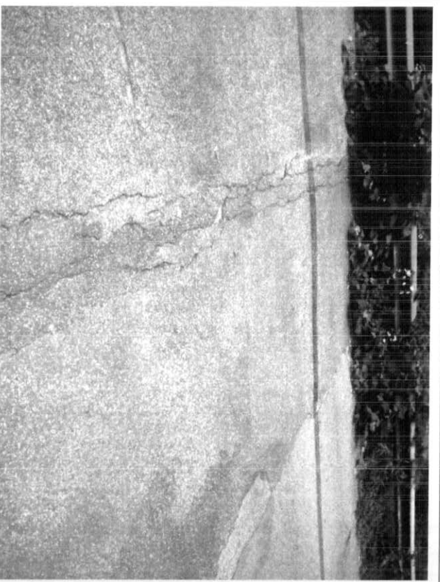
Photo # 10: TRANSVERSE CRACKS AT WEST DECK END.
