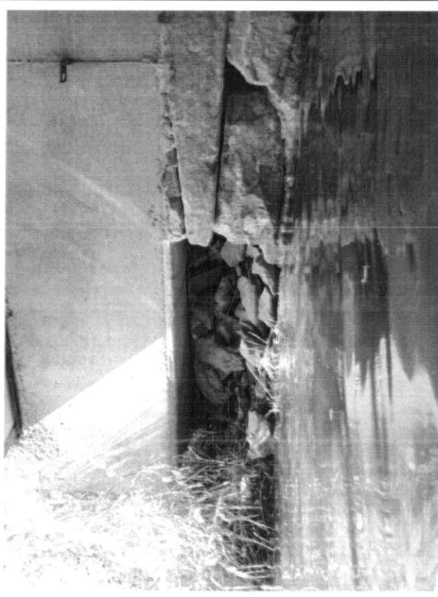
Photo # 16: Downstream (west) end of north abutment stem with showing 3'-8" long x 2' high void with 30" penetration underneath the cap and unconsolidated fill material ✓
