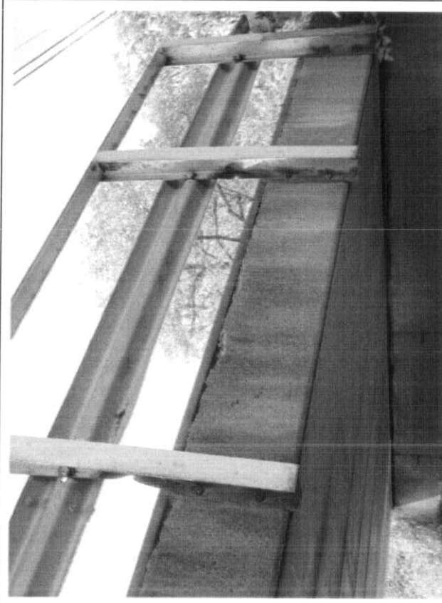
Photo # 8: Condition of west fascia concrete with edge spalling
