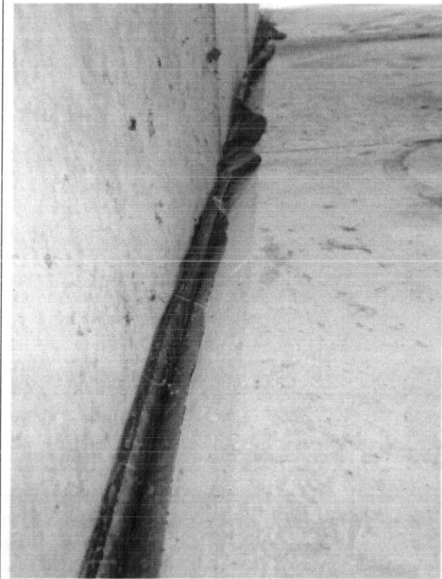
Photo # 13: Bulging bearing material for bridges at the west abutment.
