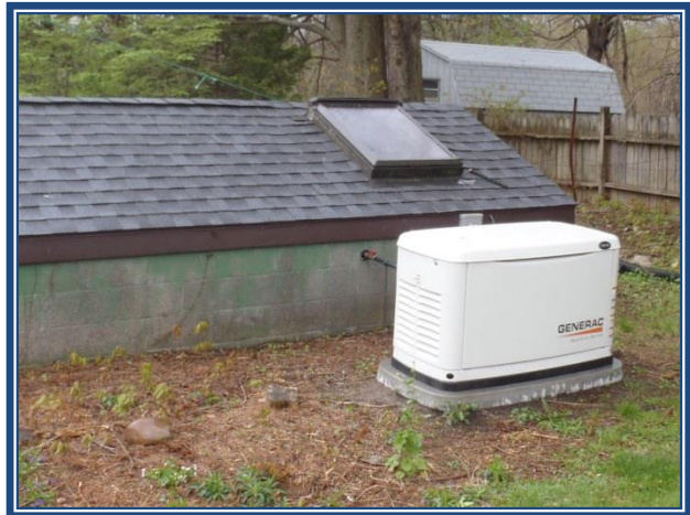
Sharon Heights Emergency Generator
