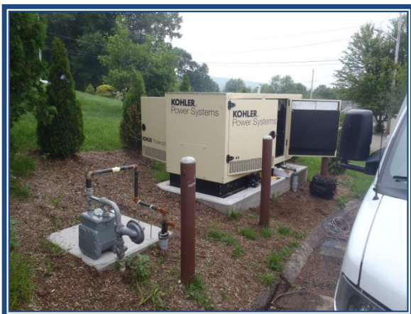
Regional Water Authority Emergency Generator
