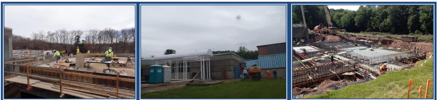
Meriden – Construction and near completion of upgraded Broad Brook Water Treatment Plant. This improved plant will help protect public health through the delivery of potable water
