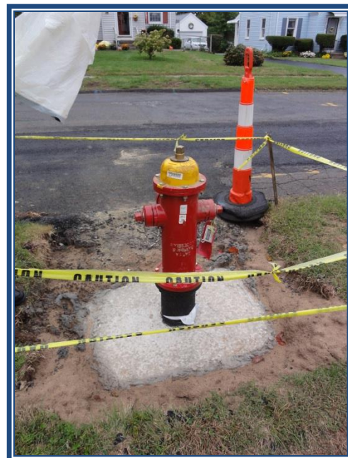
Newly installed fire hydrant
