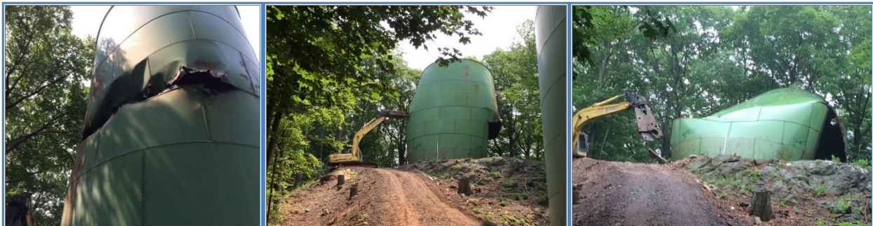
Bristol - Grove Street Tank (#2013-7023) – Elimination of Deteriorating Water Storage Tank- Protects Public Health
