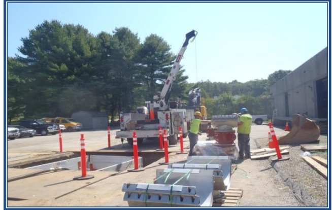
Norwich-Deep River WTP Rehab - Installation of a new isolation valve on the transmission main
