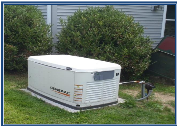
Kugeman Village Emergency Generator
