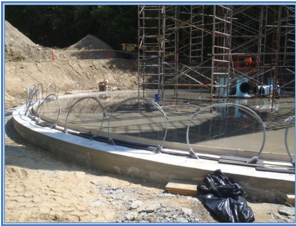
Storage Tank Foundation-Installation of scaffolding in preparation for tank wall panel installation
