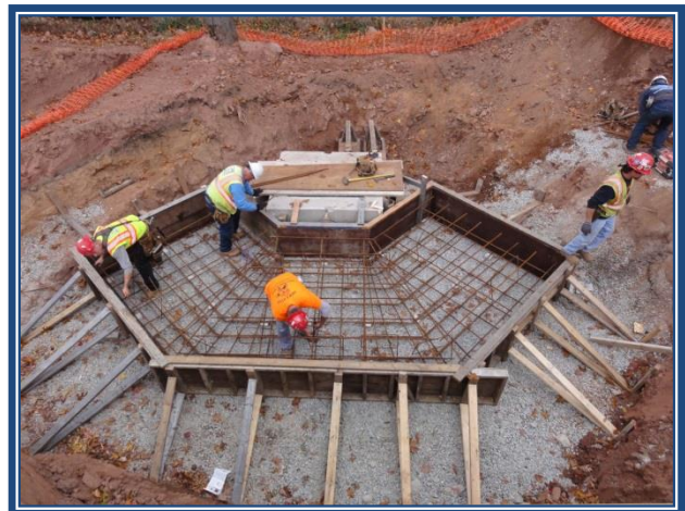
MDC Wickham Hill Storage Basins: Constructing the rebar for a concrete slab. This slab will be the foundation for an electrical building.
