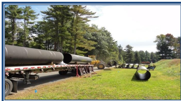
MDC - North Storage Basin - New pipes connecting new storage tank to the existing system
