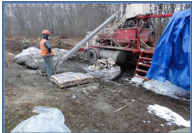
Norwich-Deep River WTP - Cement grout being injected to seal the void around the newly inserted HDPE pipes and the old transmission main
