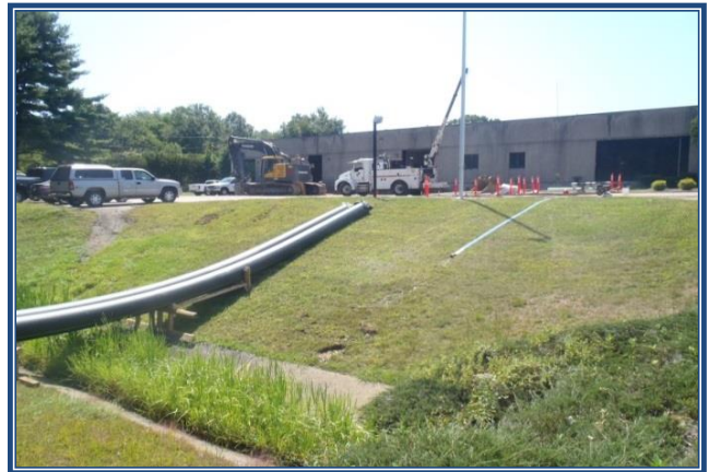
Norwich-Deep River WTP -Twin temporary High Density Polyethylene Pipe (HDPE) pipes installed to serve the distribution system while the transmission main is out of service during the rehab
