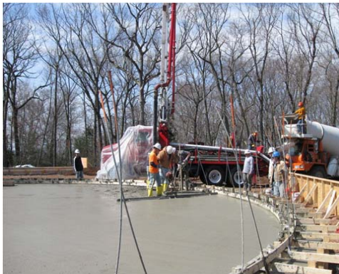
Town of Portland DWSRF Project - installation of tank floor to wall to stabilize cables embedded in concrete. Concrete floor was mechanically floated during placement of concrete.
