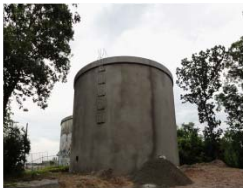
Town of Portland DWSRF Project - Water tank with shotcrete finish over wire wound pre-stressed concrete tank panels.
