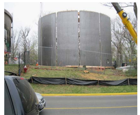
Town of Portland DWSRF Project - – Precast concrete water tank vertical panels being placed by crane.
