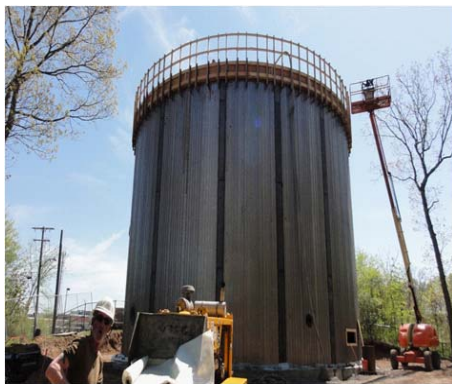
Town of Portland DWSRF Project - Pre-stressed concrete tank panel installation completed, ready for wire wound process to secure panels.
