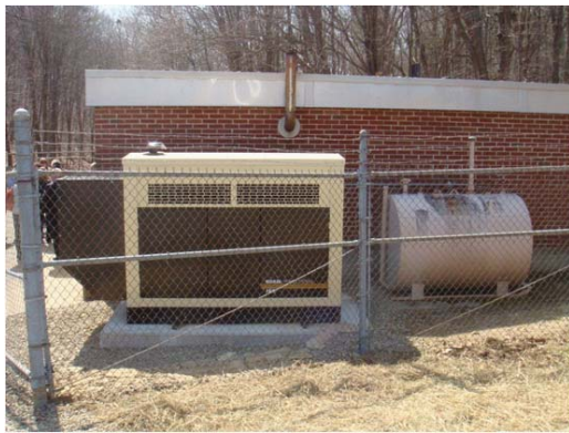
City of Norwich - Fairview - New Generator
