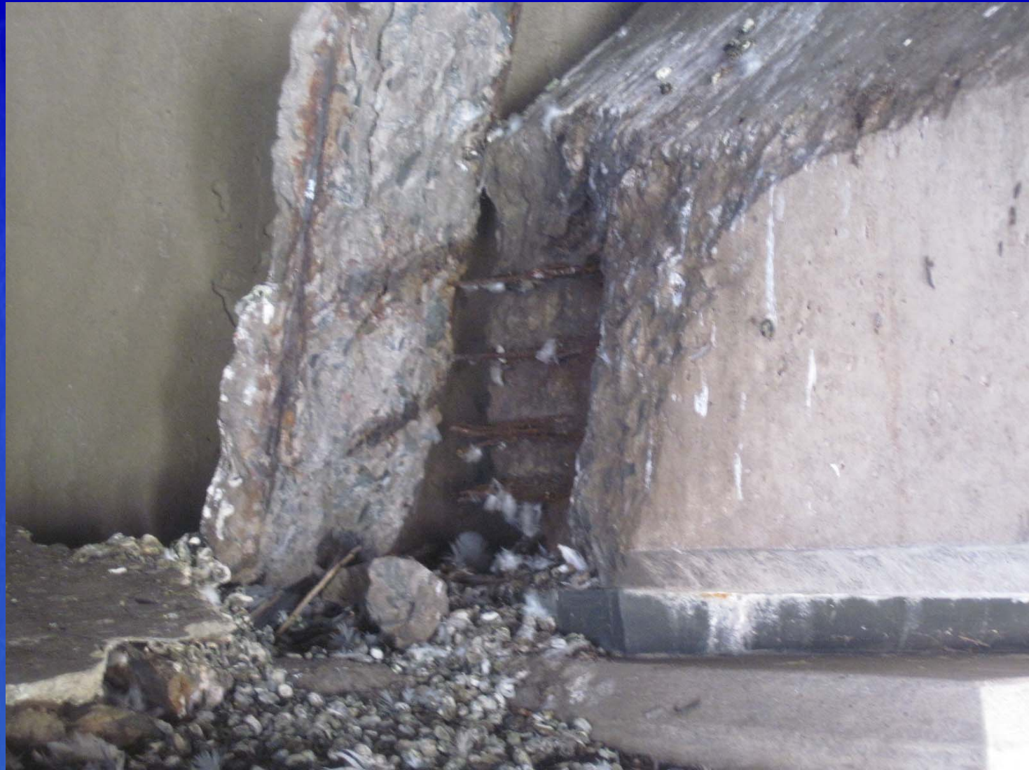
Bridge 01236 G7 spall beam end
