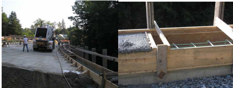
Figure 6.14: Curb Concrete Placement and Cold Joint
