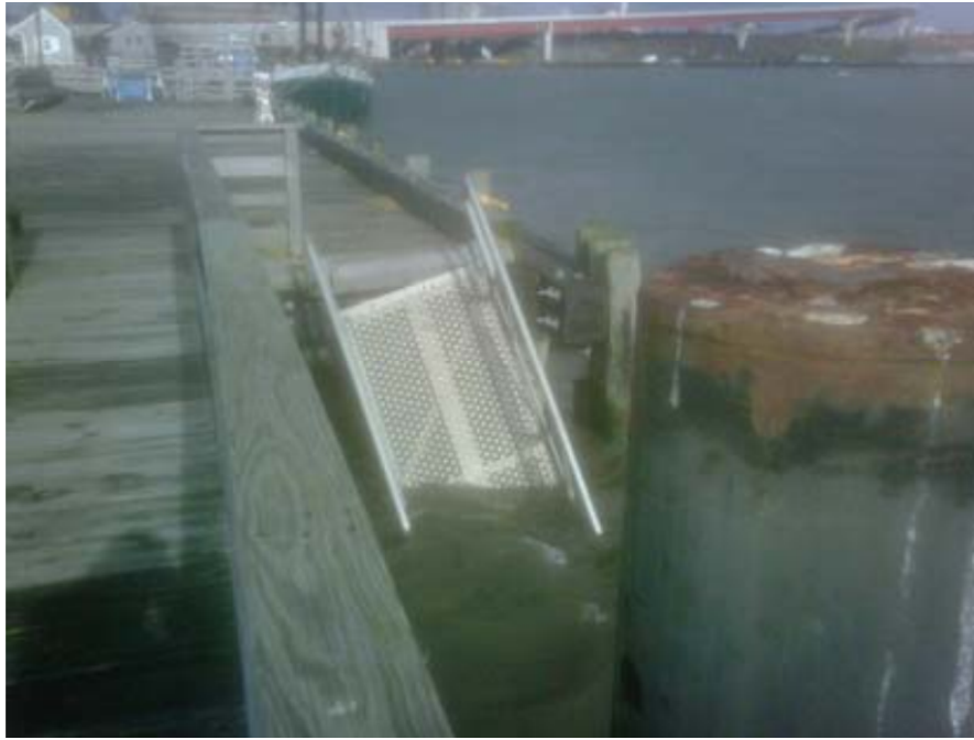
Fig. 1.2 Damage to Long Wharf Pier in New Haven, due to Superstorm Sandy (Source: City of New Haven Engineering Department).
