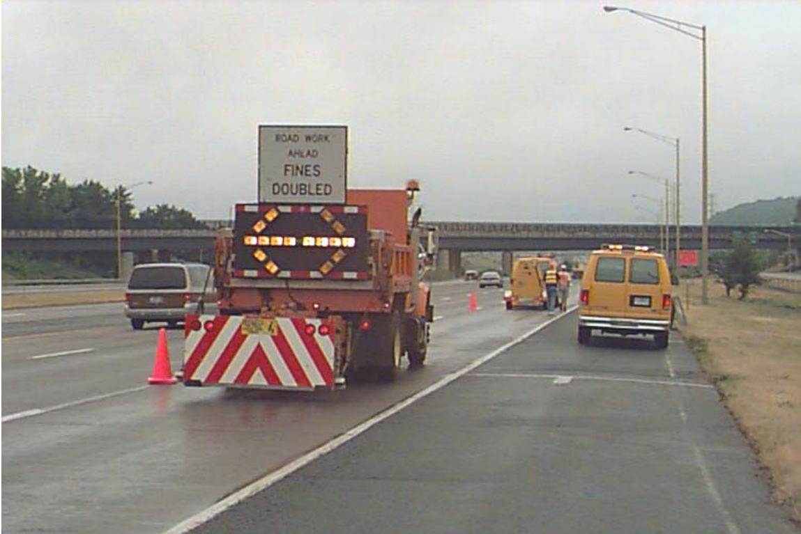
Image 10: ConnDOT Providing Lane Closure for LTPP FWD and Distress Survey Manchester, CT (Site 094008)
