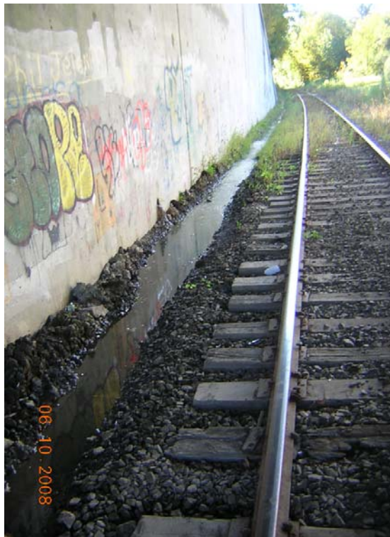
Standing water by tracks under Whisconier Road Bridge (HRR – Berkshire Line)
