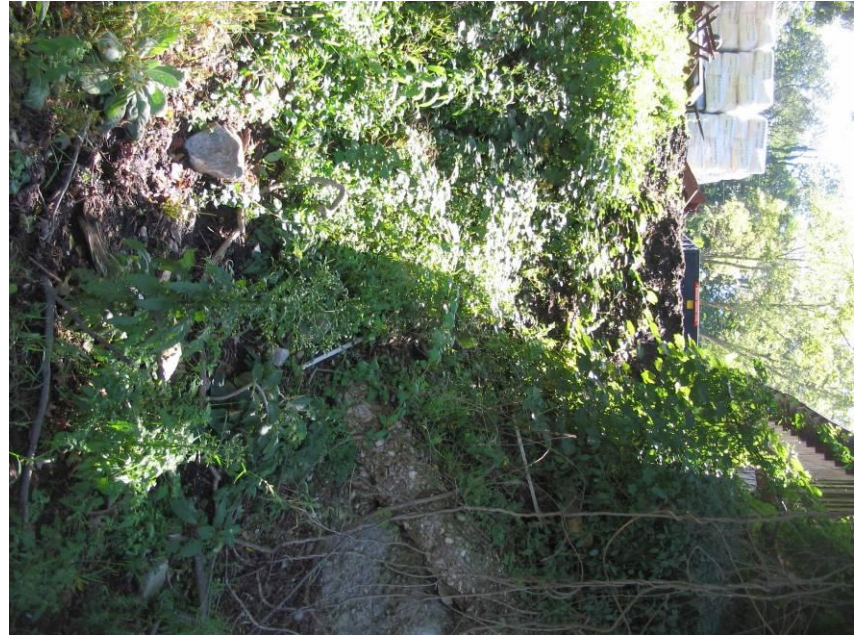
MP 7.82 (E) MNR - Washout
