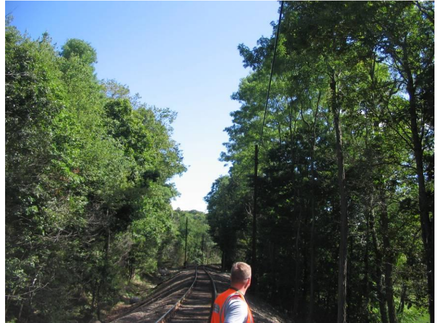
MP 14.75 (S) MNR – OH fiber optics cable crossing
