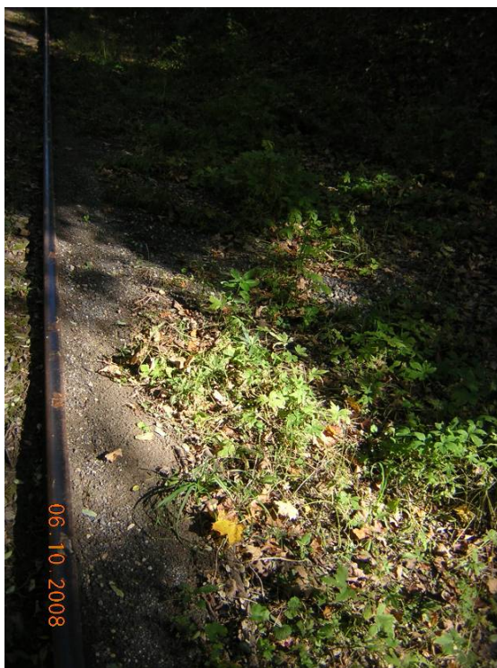
Sediment Build-up at Tracks (HRR - Berkshire Line MP 1.5)
