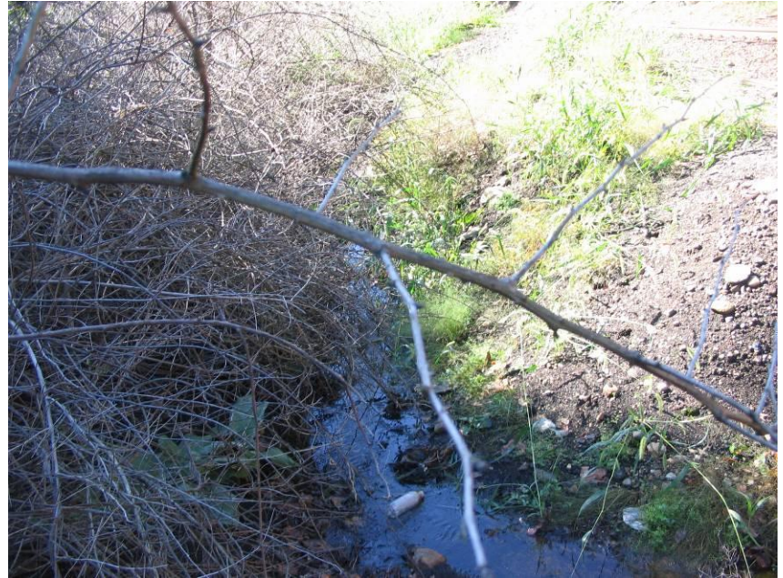
MP 9.2 (S01) MNR – Drainage by tracks
