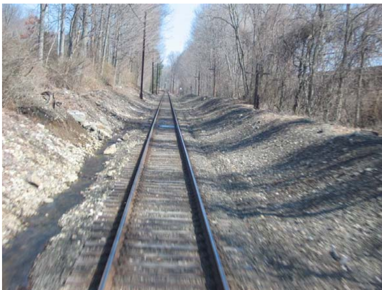
Standing Water along West Side of Tracks (MNR MP 4.70)
