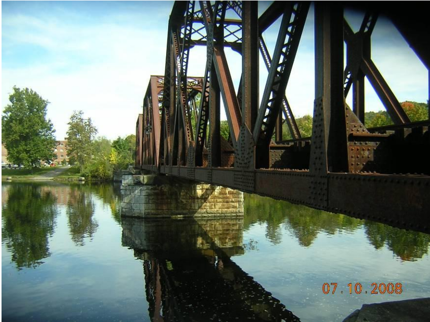
MP 10.16 (N) HRR – UG Housatonic River
