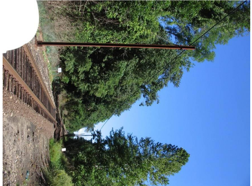
MP 8.5 (N) – OH fiber optic cable crossing
