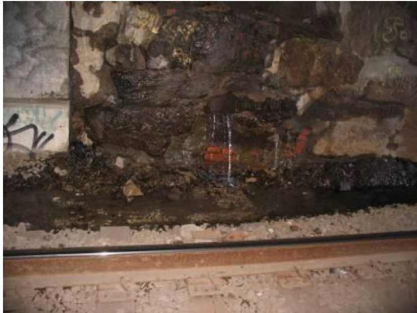
Figure 2 - Water seeping through retaining wall at south entrance of Wall St. Tunnel (MNR MP 1.5)
