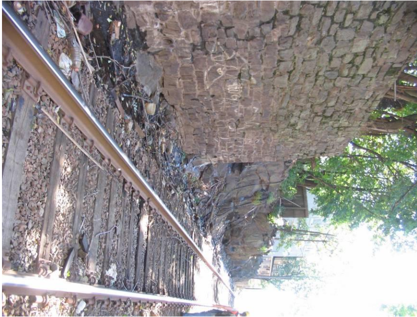
MP 1.4 (SE02) MNR – State of tracks south entrance of tunnel
