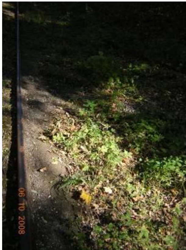
Figure 5 - Sediments washed down to tracks to TOR (HRR - Berkshire Line MP 1.5)
