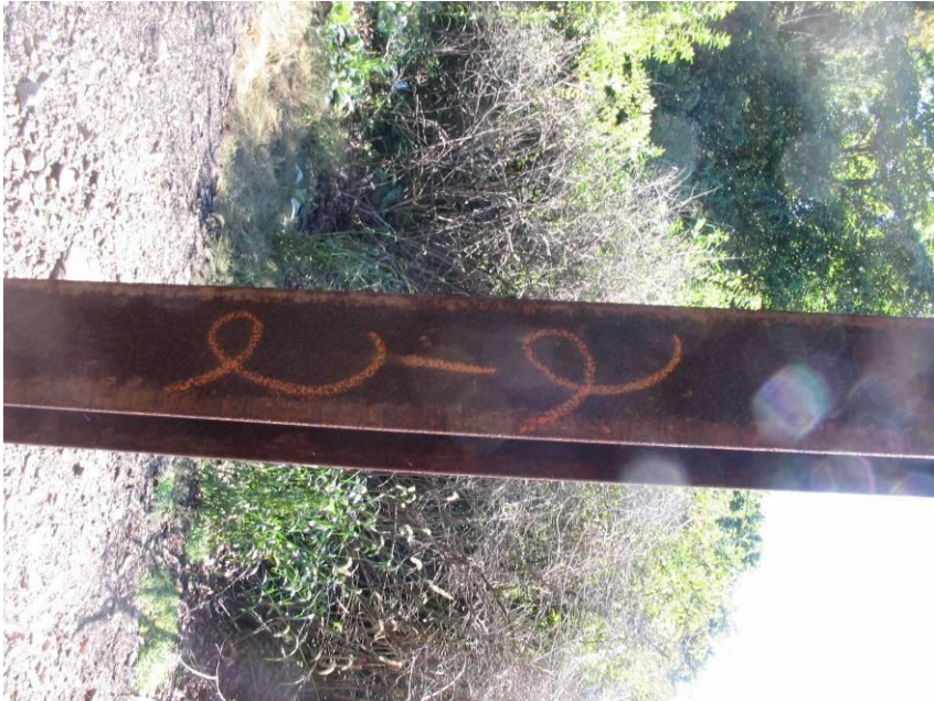
MP 9.0 (E) MNR – Existing Cat. Pole
