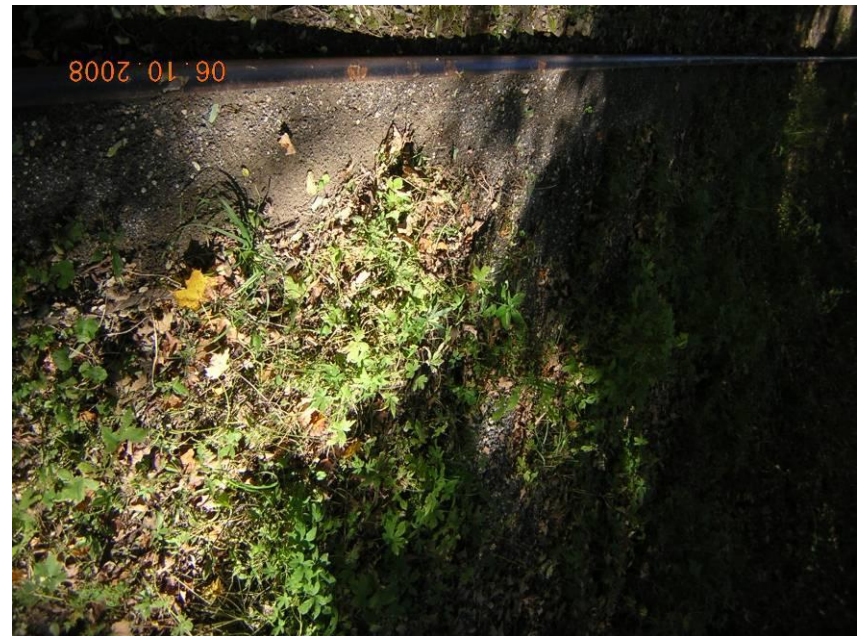
MP 1.5 (NE) HRR – Washout (Soil/debris to TOR)
