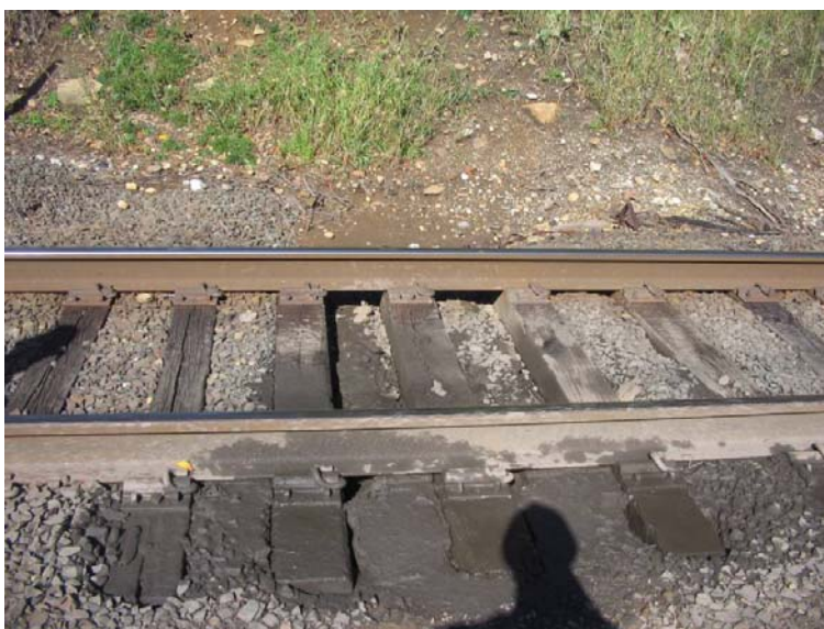
Poor Drainage (MNR MP 9.40)
