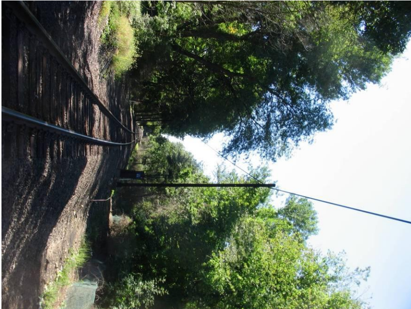
MP 8.4 (S) MNR – OH fiber optics cable crossing
