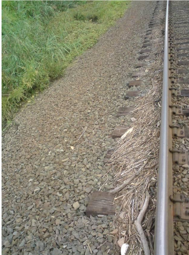
Figure 6 - Debris on tracks due to flooding (MNR MP 21.3)
