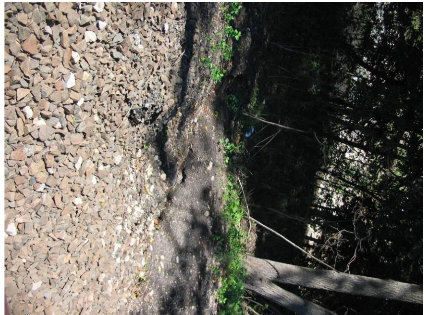
MP 3.2 (W) MNR - Washout
