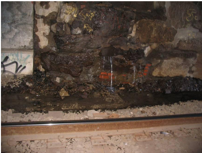
MP 1.4 (NE03) MNR – Drainage at south entrance of tunnel
