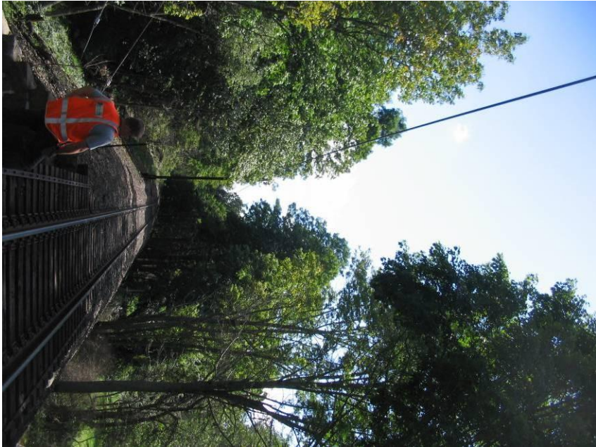
MP 14.16 (S01) MNR – OH Fiber optics cable crossing
