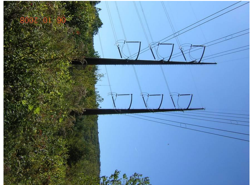
MP 5.7 (W) HRR – OH Power lines
