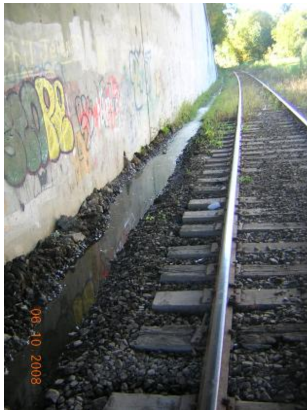
Figure 3 - Standing water by tracks under Whisconier Rd Bridge (HRR – Berkshire Line MP 4.4)
