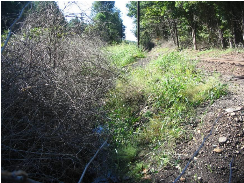
MP 9.2 (S02) MNR – Drainage by tracks
