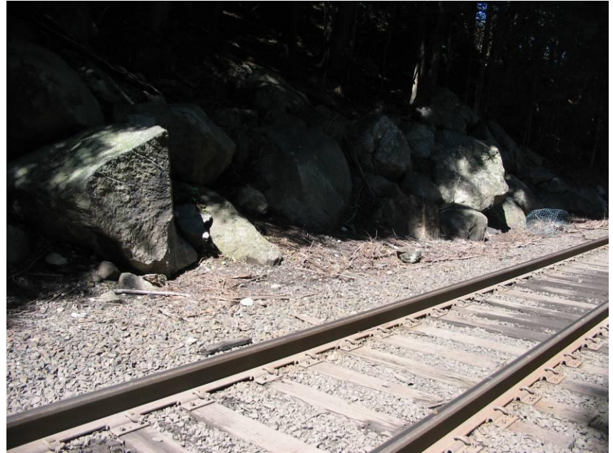
MP 11.65 (N02) MNR – State of tracks & washout
