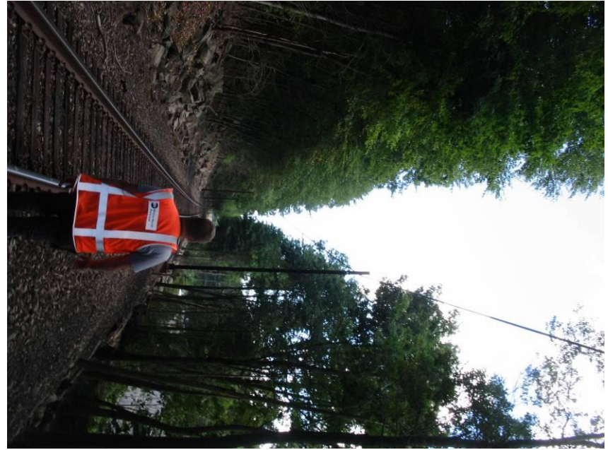
MP 13.2 (S) MNR – OH Fiber optics cable crossing
