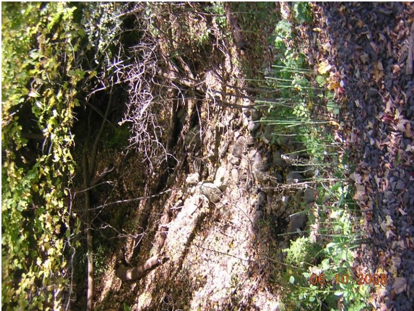
MP 5.0 HRR – Drainage by tracks
