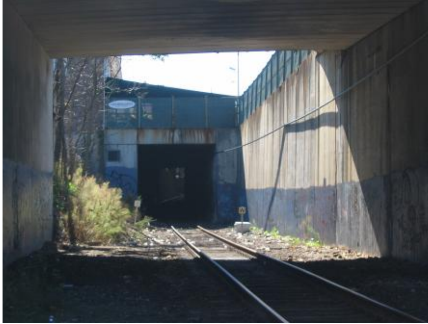
Figure 19 – North entrance of Wall Street Tunnel (MNR MP 1.5) Restrictive horizontal clearance at South Norwalk tunnel.
