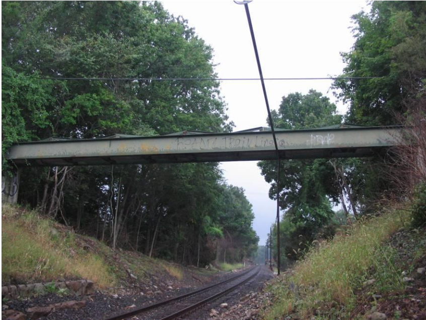
MP 6.25 (N) MNR – Utility over tracks
