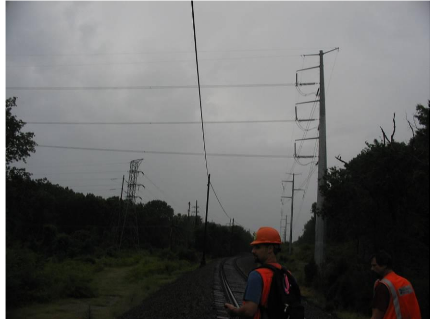
MP 5.59 (S01) – OH Power lines
