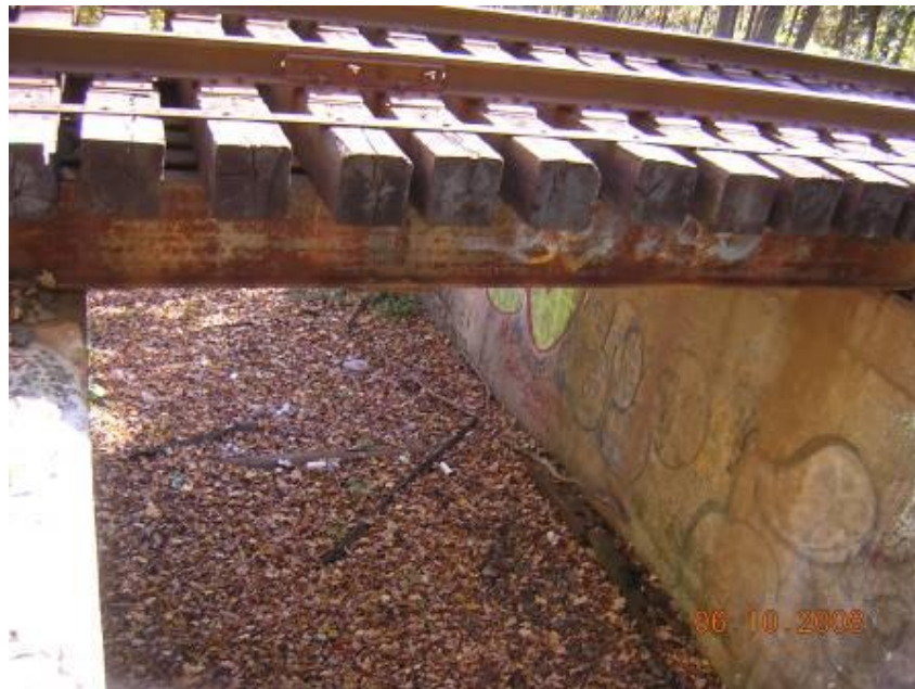
Figure 11 - Cattle Pass (HRR – Berkshire Line MP 2.96) Steel support beam rusted and in need of painting.
