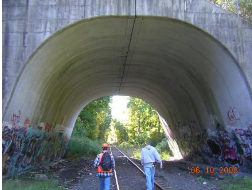
Figure 8 - Gray's Bridge Rd (HRR – Berkshire Line MP 1.59) Overhead bridge is in good condition.
