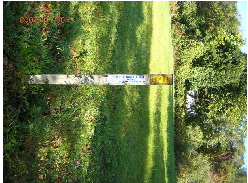
MP 3.3 (E) HRR – Gas pipeline by Oak Grove Rd.
