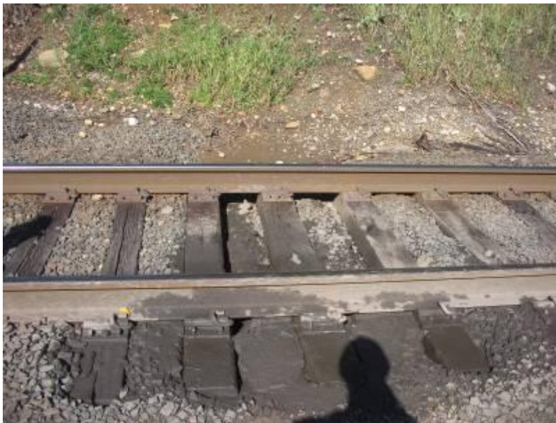
Figure 7 - Poor maintenance of grade and ballast (MNR MP 9.40)
