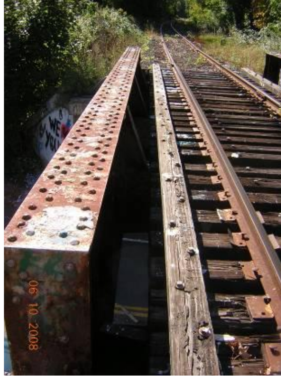
Figure 14 - Junction Rd (HRR – Berkshire Line MP 2.51) Deteriorating timber and rusting at truss were observed.
