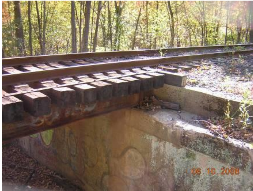
Figure 10 - Cattle Pass (HRR – Berkshire Line MP 2.96) Concrete spalling observed on abutment wall.
