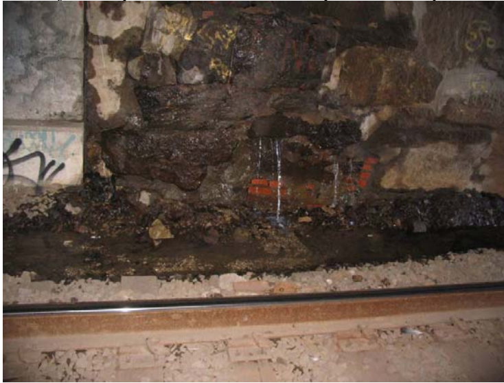
Water Leakage at East Abutment at Wall Street Tunnel (MNR MP 1.50)
