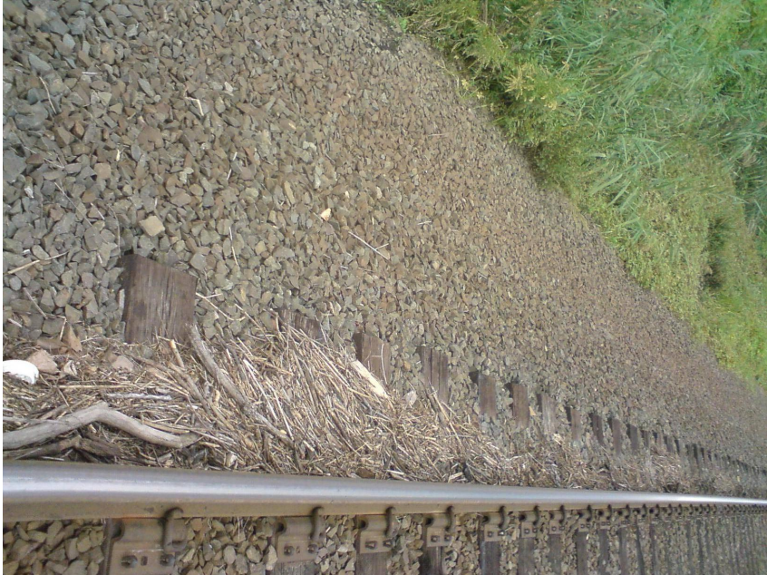
MP 21.3 (S) MNR – Debris showing recent flooding of tracks
