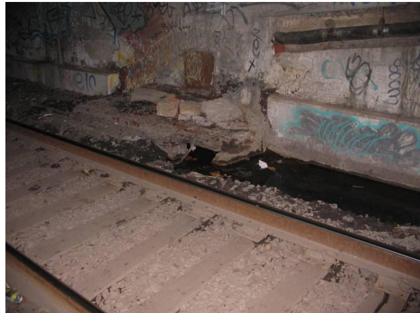
MP 1.4 (NE02) MNR – Drainage at south entrance of tunnel
