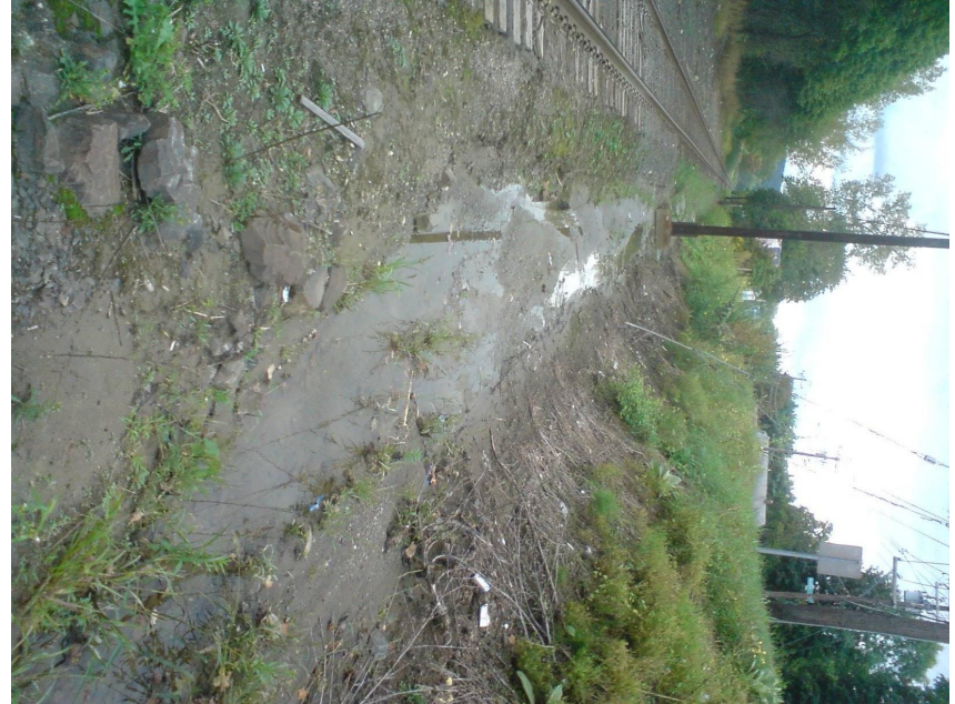
MP 21.7 (S) MNR – Drainage near AG Great Pasture Crossing
