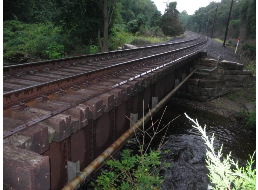
MP 6.64 (S01) - UG Stream OD – FO cable running along bridge
