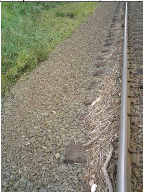
Debris along Tracks due to Flooding (MNR MP 21.3)
