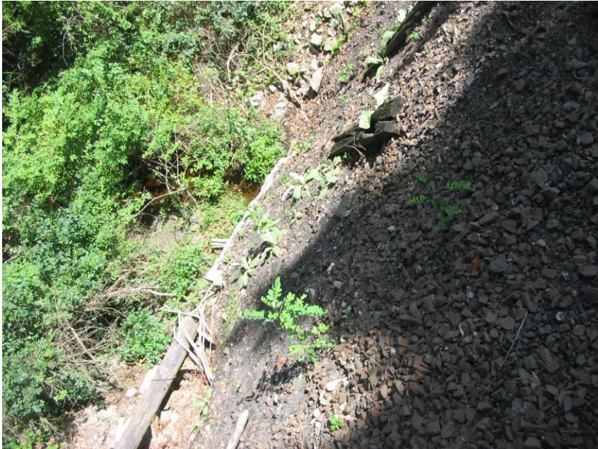
MP 14.6 (E) MNR - Washout
