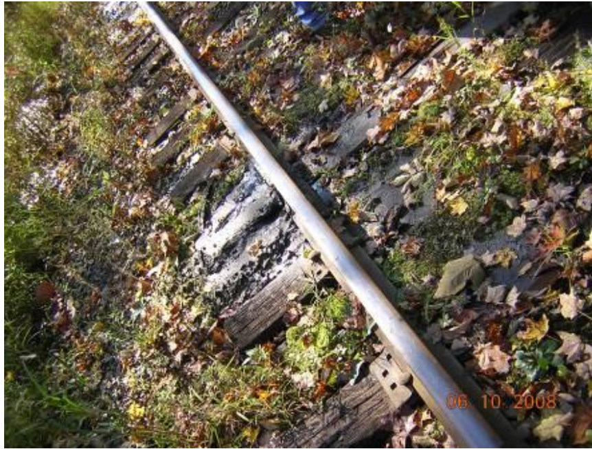
Figure 4 - Poor drainage on tracks HRR - Berkshire Line MP 3.1)
