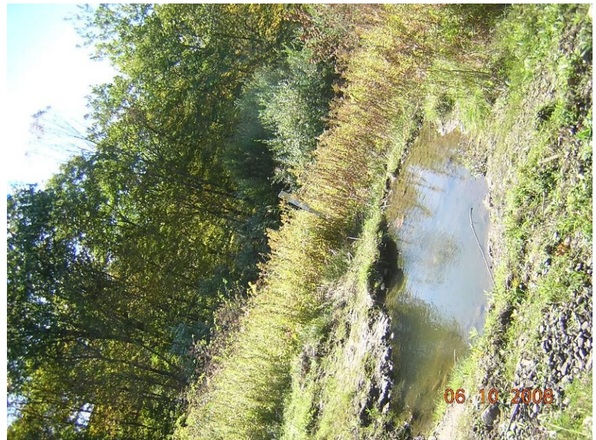
MP 4.8 (W) HRR – Gas pipeline
