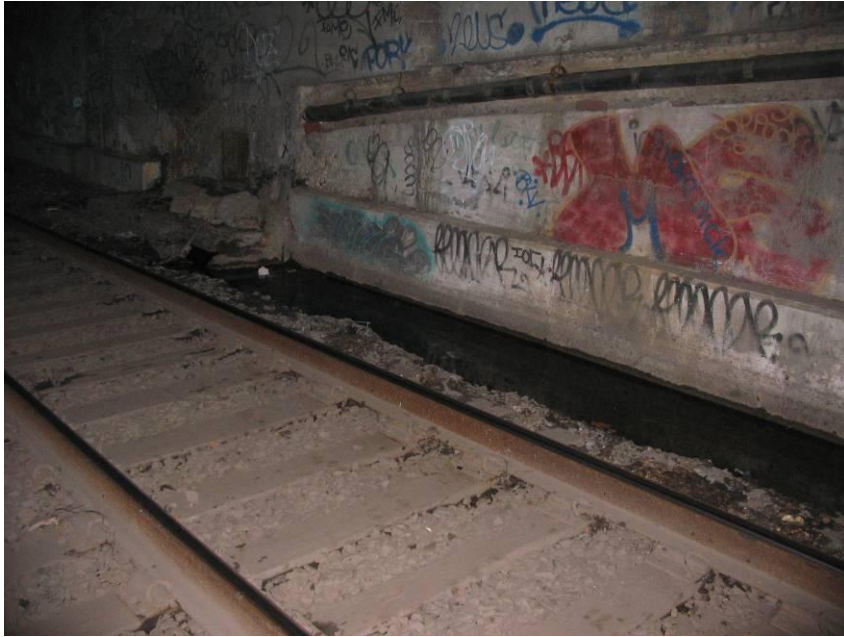
MP 1.4 (NE01) MNR – Drainage at south entrance of tunnel
