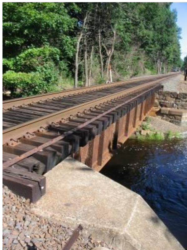
Figure 9 - Norwalk River (MNR MP 8.7) Bridge is in poor condition according to bridge inspection reports. Observed deficiencies include rust on steel beam supports.
