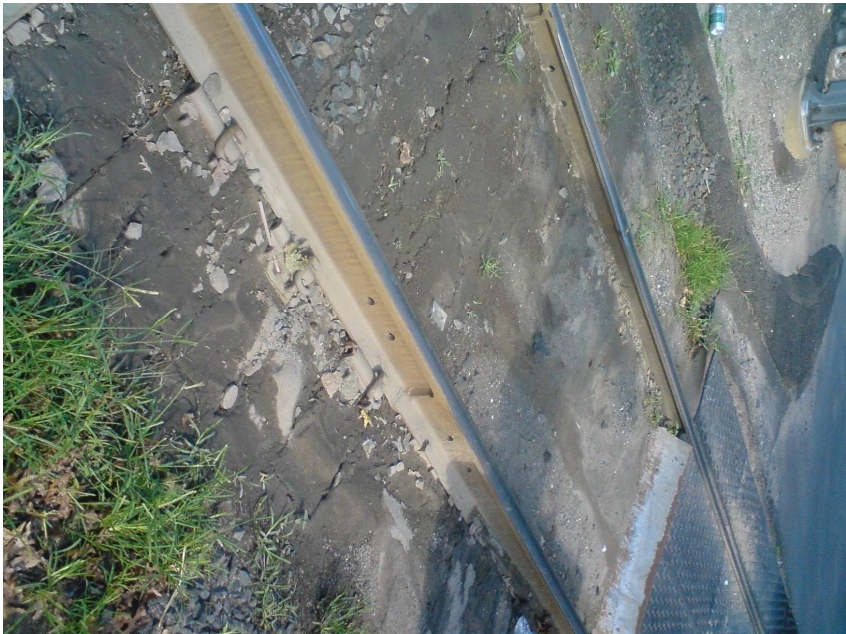
MP 22.21 (S) MNR – State of tracks at AG Shelter Rock
