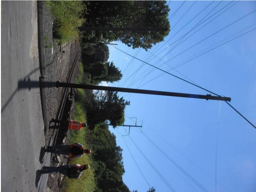
MP 4.93 (S01) MNR – OH Utilities at Kent Rd.
