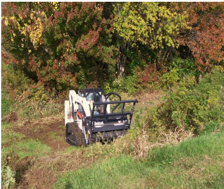
Bobcat with forestry attachment clearing vegetation adjacent to drainage system within bowl area
