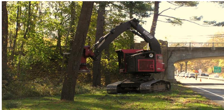
Feller buncher removing trees within the clear zone along the Merritt Parkway
