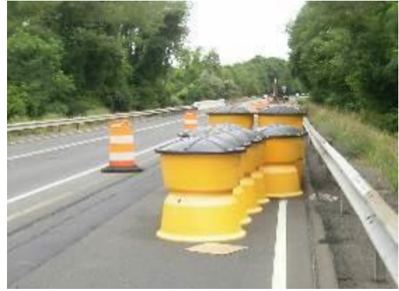
Temporary impact attenuation system is protecting blunt end of TPCBC. End delineator needs to be reattached.
