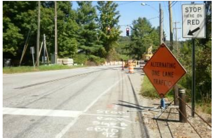
Stop bar and signs at approach to one lane traffic.
