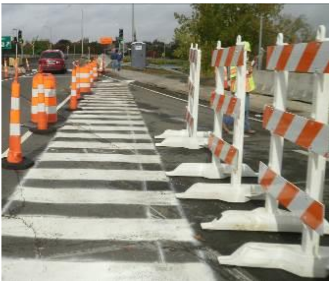
Crosswalk markings added for pedestrian guidance. A field decision was made to use traffic cones & drums, on left, in place of Type III Construction Barricades.
