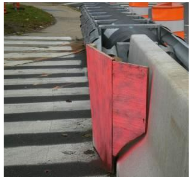
The end of the impact attenuation system in the temporary pedestrian walkway was framed out for protection.
