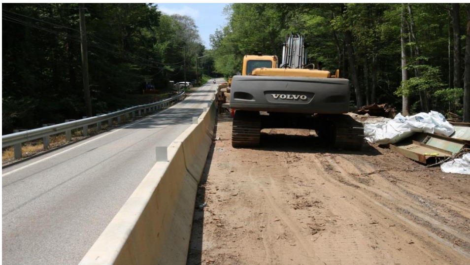
Photo 7: All equipment and materials was stored behind temporary barrier or at least 16 feet off of the roadway.
