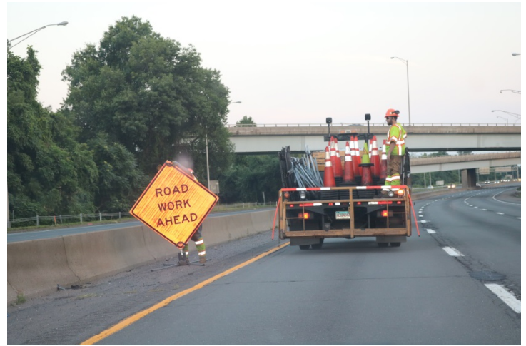
I-91 SB: A ROAD WORK AHEAD sign is installed only on the left side.
