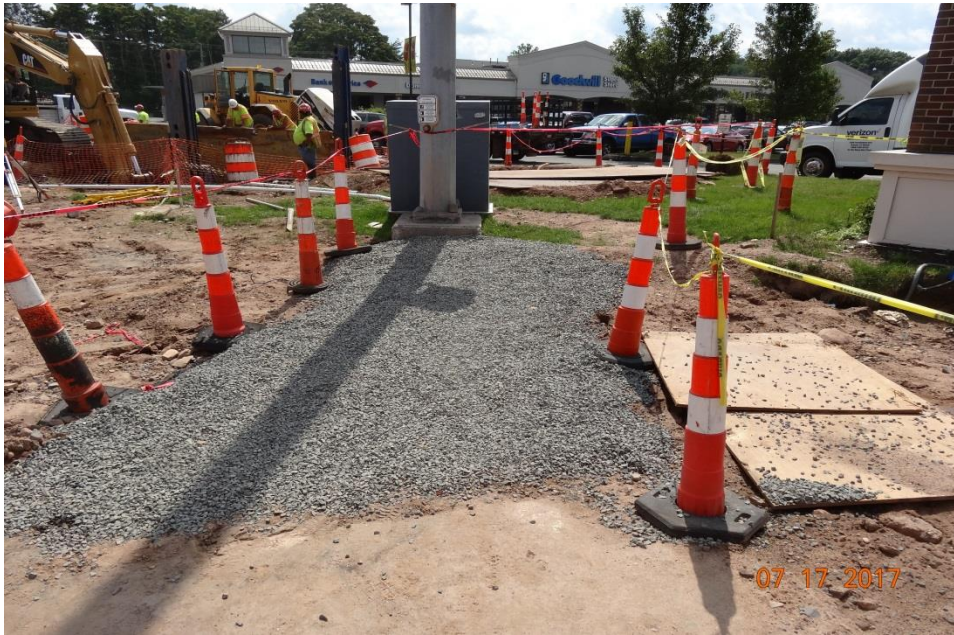
Photo 10: This temporary ramp to the push button located on the span pole was well formed, but it was done with loose ½ inch stone. A wheelchair would have trouble traversing through the loose stone. A more dense graded material that compacts to form a tight surface should be used.
