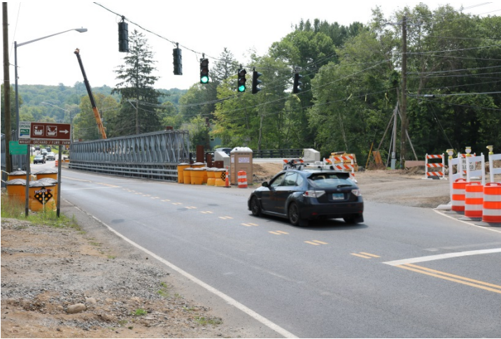
Route 74 EB (Tolland Stage Road): The temporary bridge with the temporary signal. There are impact attenuation systems protecting the ends of the bridge with DE-9 delineators on front.
