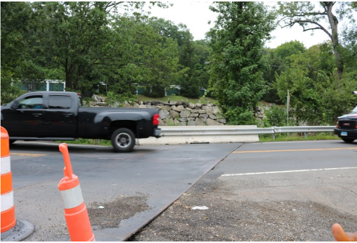
Route 7: Since metal beam rail posts could not be installed on the steel plates, a TPCBC is placed on the steel plate behind the guiderail with attachments.
