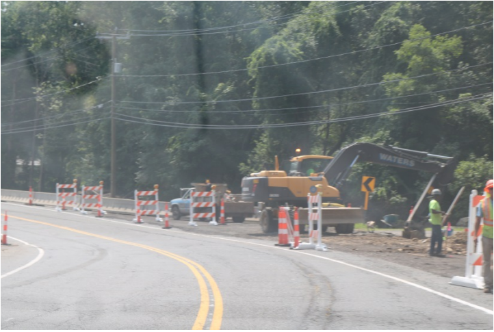
Route 74 EB (Tolland Stage Road): Approaching the project site around the bend in the road. There are Type III barricades that close the shoulder of the road.
