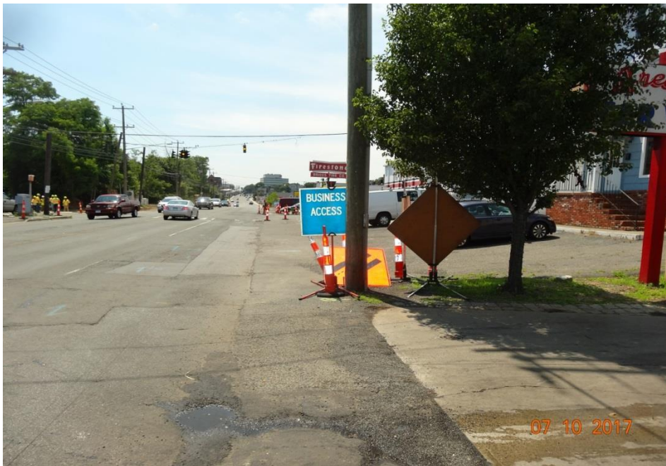
Photo 10: Route 1, SB. "Business Access" signs were placed as needed in front of business driveways that may be obscured (even slightly) to inform motorists and pedestrians that they are still open during construction.
