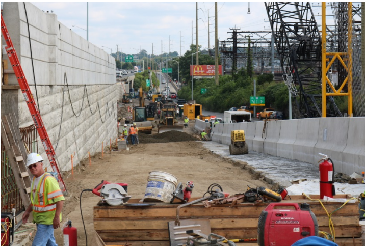
This is the work area on the newly installed bridge to be the new Exit 8 Ramp.
