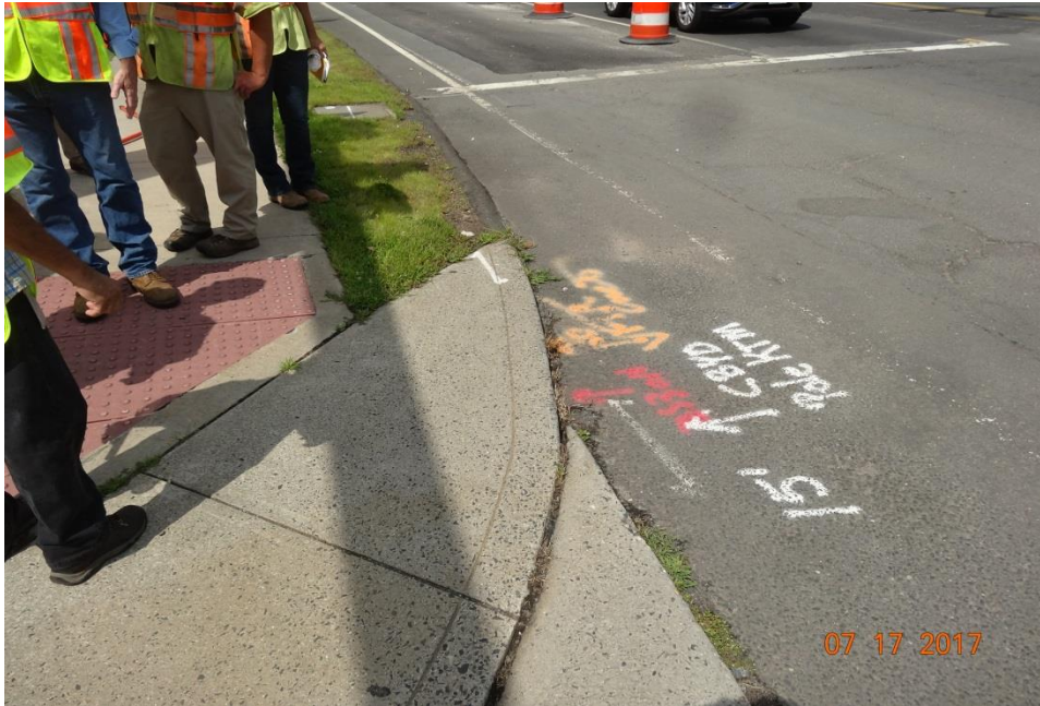
Photo 13: This is the ramp just in front of the closed sidewalk (in Photo 12). You can't see it in this picture but the driveway concrete apron to the right has a 2 inch lip. Because side walk users are being diverted across this apron in order to cross to the sidewalk on the other side of the roadway, this "lip" should be wedged with a little bit of HMA so that wheelchairs don't potentially get hung up on it.
