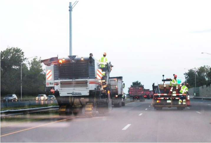
I-91 SB: The equipment and dump trucks are stationed in the left lane. The RRB continued despite the lanes being closed to ensure motorists don't pass the sign truck and come into the left lanes where the equipment is.
