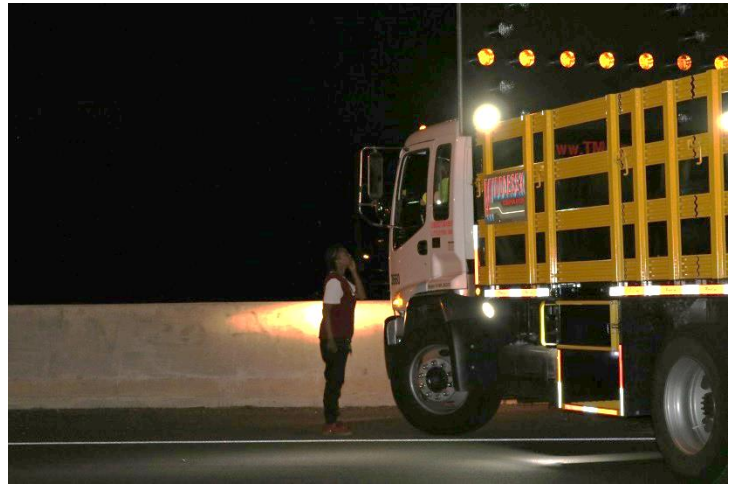
I-84 EB, Exit 45: A sign truck is closing the on ramp while the sign crew installs the pattern and a motorist had to voice her opinion to the truck driver.
