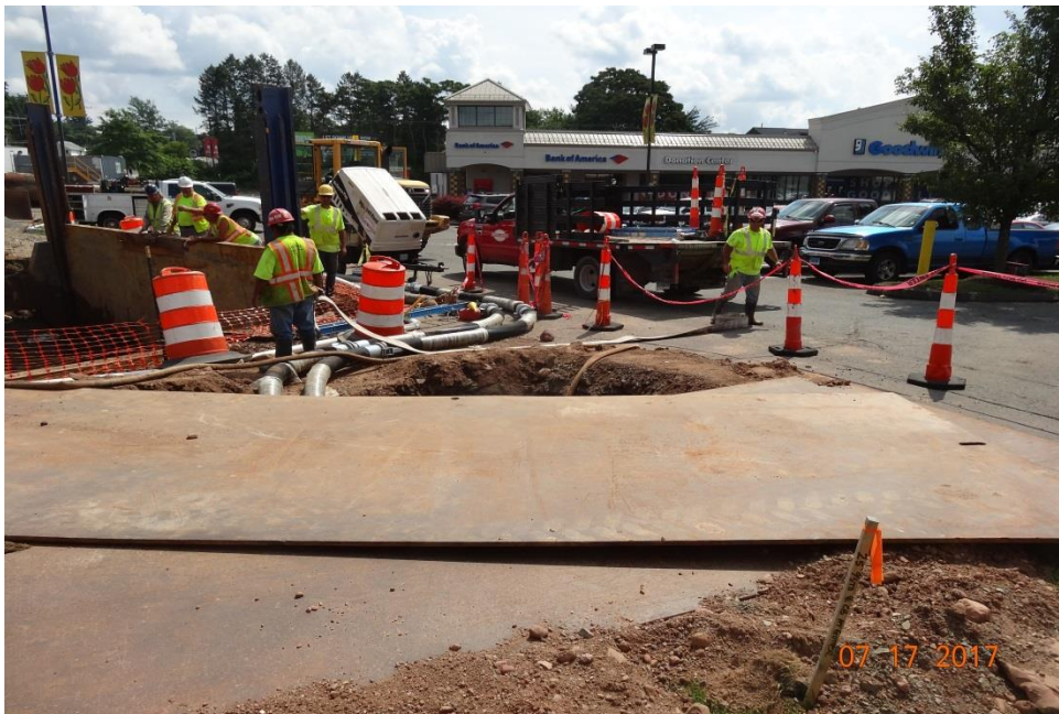
Photo 11: Here, the Contractor makes good use of sheeting to cover and protect excavated areas.
