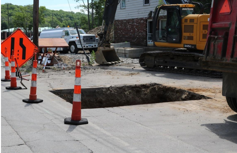
Photo 9: Here, the Contractor had just completed excavation of a small pit, 10'x12'x6'deep. The protection around the pit is inadequate. Pedestrians or anyone walking through this area are susceptible to falling in. Better protection is needed to fully block off this pit to anyone passing through this area.
