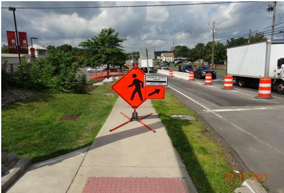
Photo 12: This sign was well placed showing a closed sidewalk and indicating an alternate route (detour) to the sidewalk across the street.
