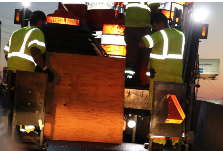
The Contractor has the signs mounted on plywood which is an acceptable rigid material to use.
