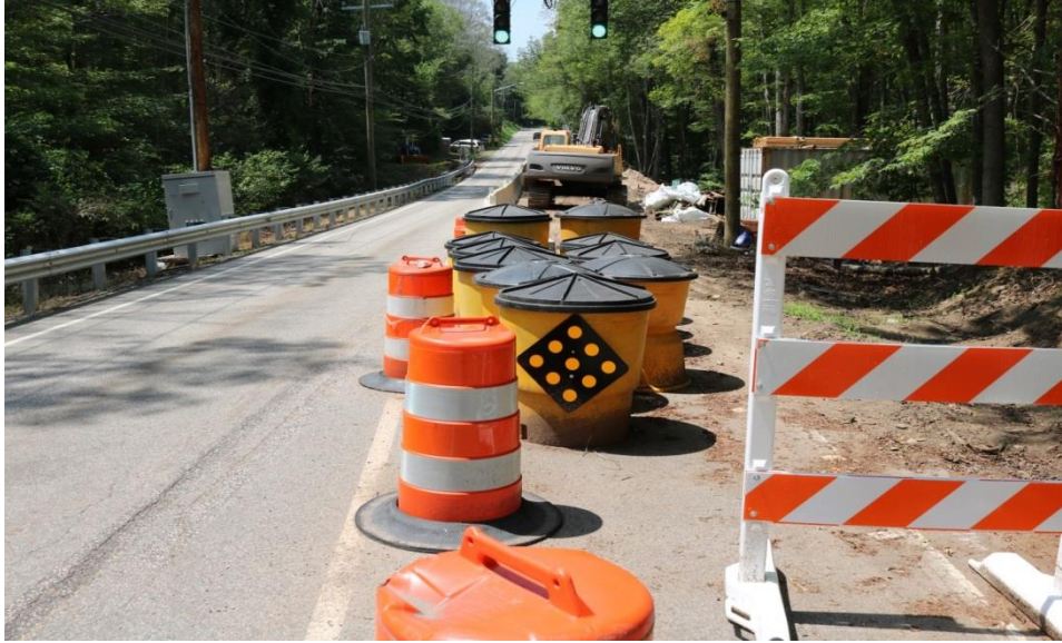
Photo 6: The work site is well delineated, protected, and bounded so as to keep motorists and pedestrians out of the work zone. The DE-9 sign has been replaced with new sign No. 50-5032
