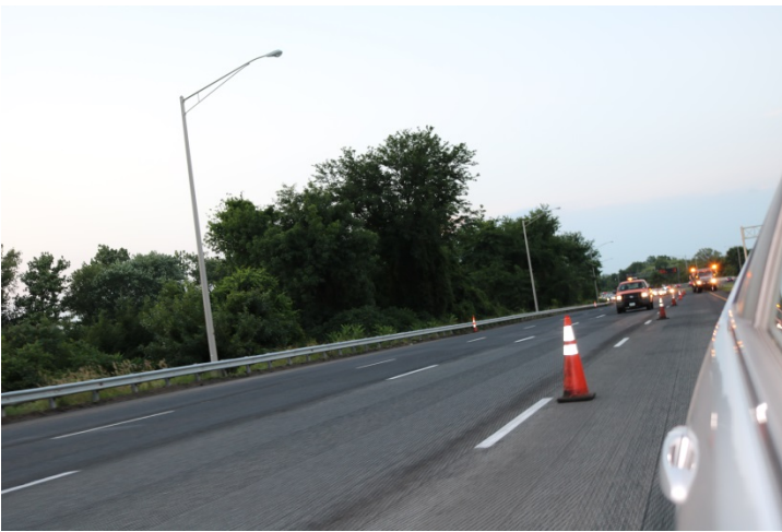
I-91 SB: A Rolling Road Block is used to slow traffic in all four lanes while the entire pattern is being installed. State Police, TMAs, and Maintenance vehicles are used to slow traffic. The RRB started at 7:47 PM.
