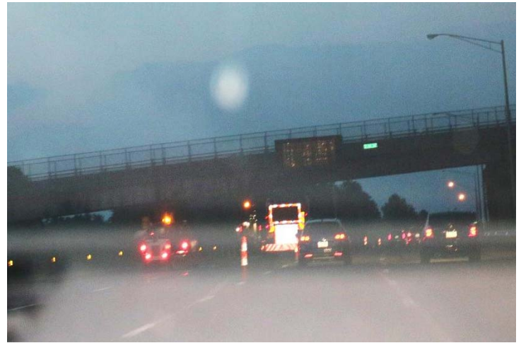
I-91 NB: The VMS over the northbound side didn't display any messages about the work zone below.
