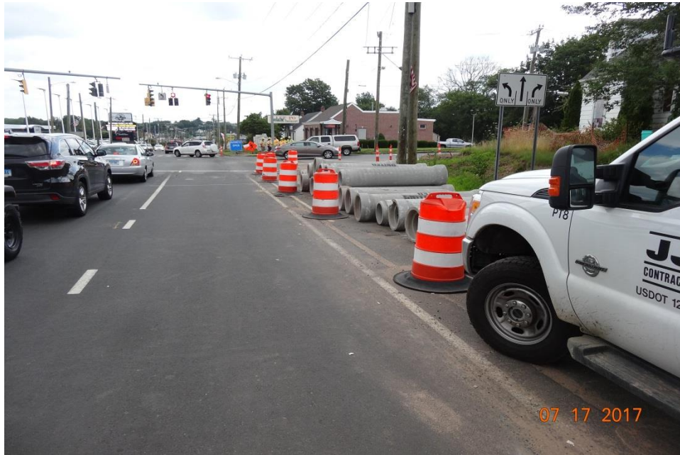
Photo 17: Like Photo 15, this concrete pipe was stored right along the edge of the travelway.
