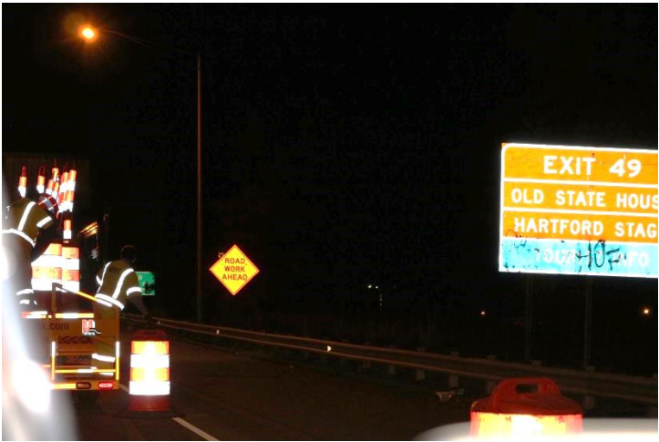
I-84 EB: The taper of the pattern is started with traffic drums. There is a post-mounted sign with an attached warning light on the right.
