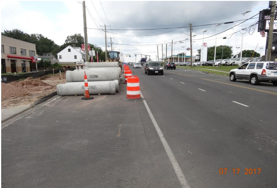
Photo 15: Here materials are stored unprotected right along the edge of the travelway. All materials and equipment must be stored a minimum 16 feet off of the roadway or behind concrete barrier.
