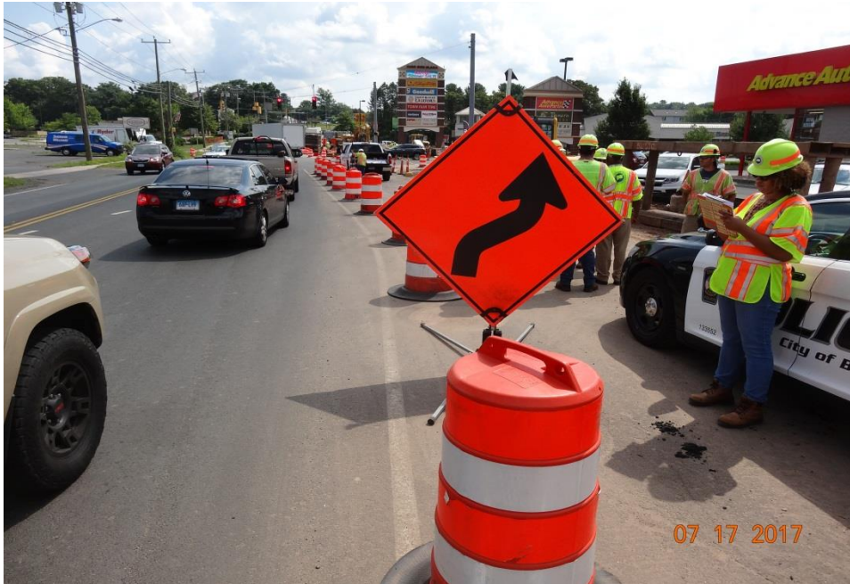
Photo 8: Photos 8 and 9 showing a sign made from corrugated plastic board. Several signs throughout the project were made of this material. All signs should be made of plywood or aluminum sheeting. Corrugated plastic board signs tend to warp and get bent over time. This detrimentally affects their reflectivity at night. In addition, this sign encroaches a little on the travel way. It could possibly get clipped by a passing vehicle.
