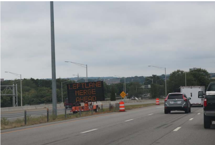
I-95 SB: The second frame state "LEFT LANE MERGE AHEAD".
