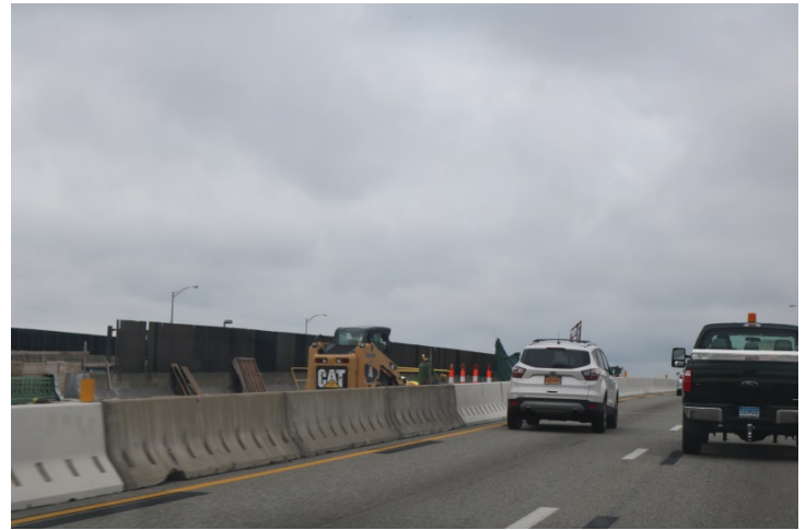
I-95 SB: This is the work zone within the median behind TPCBC.
