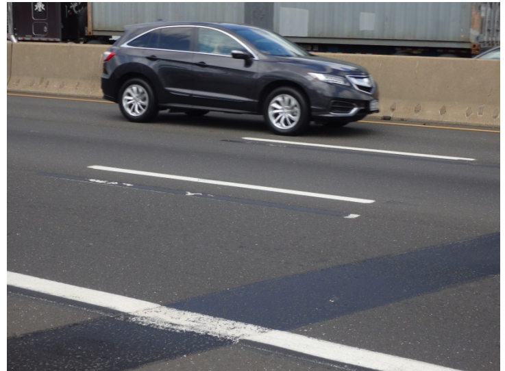
On I-95 pavement markings covered with black aggregate cover-up resin pavement markings are starting to wear and should be refreshed.
