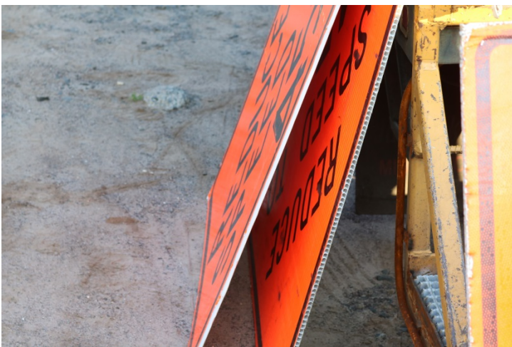
The construction signs are mounted on waffle board which is unacceptable material. The waffle board reduces the reflectivity of the signs.
