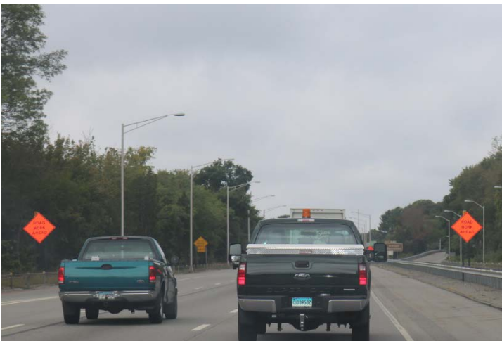
I-95 SB: Next, the ROAD WORK AHEAD signs are mounted on both sides of the road
