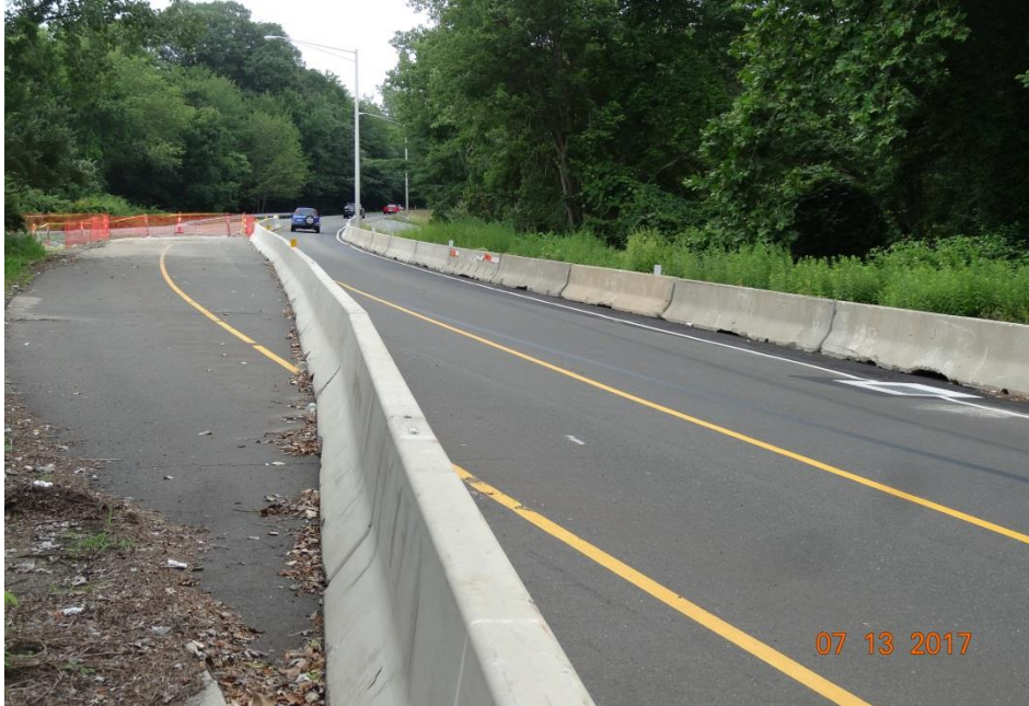
Photo 9: This is the connector ramp from 15 S to 25 N. Temporary concrete barrier was used to shift traffic to one side of the ramp. Stage 2 will shift the traffic back to the left side in order to complete the installation of the tunnel.
