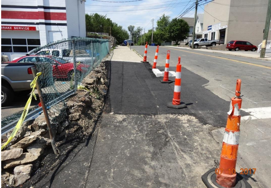
Photo 9: Stuart Road at Route 1. Here, the Contractor has maintained the condition of the side walk during reconstruction by surfacing the affected area with temporary asphalt. Also, notice that the cone closest in the photo is in poor condition. As cones and barrels deteriorate they should be removed from the project and replaced accordingly.
