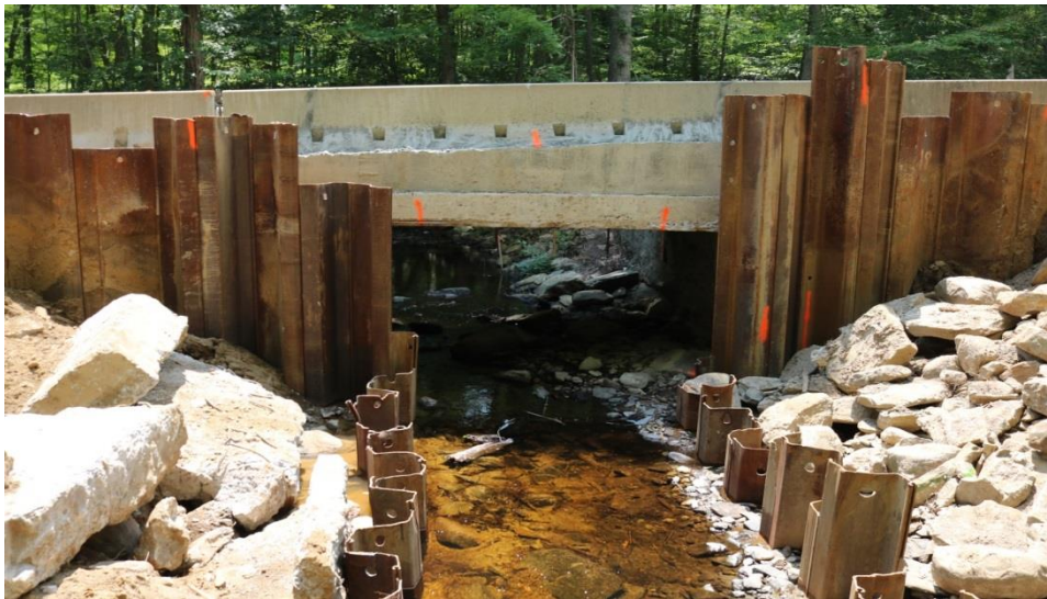
Photo 9: Here, temporary concrete barrier is well "pinned" to the existing bridge deck.
