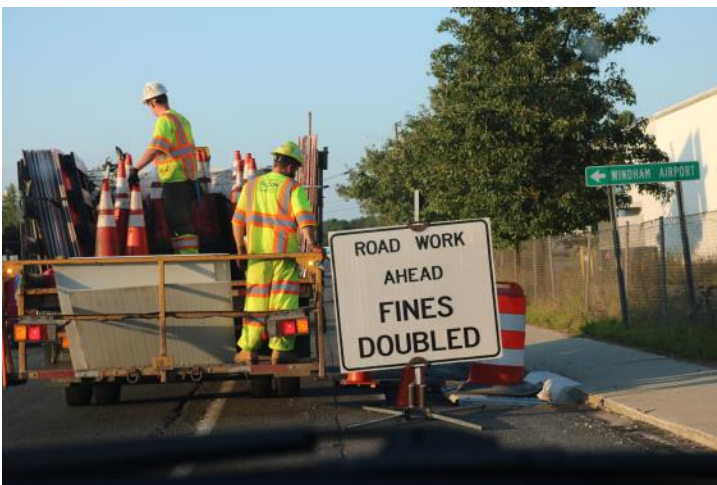
Route 6 EB: The first sign to be placed is a FINES DOUBLED sign.
