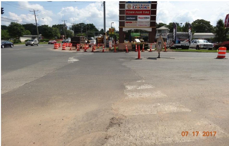
Photo 7: If key traffic markings are eradicated by construction activity they may need to be re-established before the final pavement surface is placed. Here a cross walk was almost completely removed by a large drainage trench. Drivers unfamiliar with the area may not recognize that this is a designated crosswalk area that will be frequented by pedestrians.
