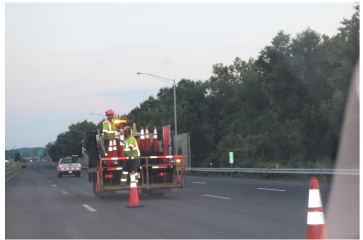
I-91 SB: The taper for the center left lane is being installed.
