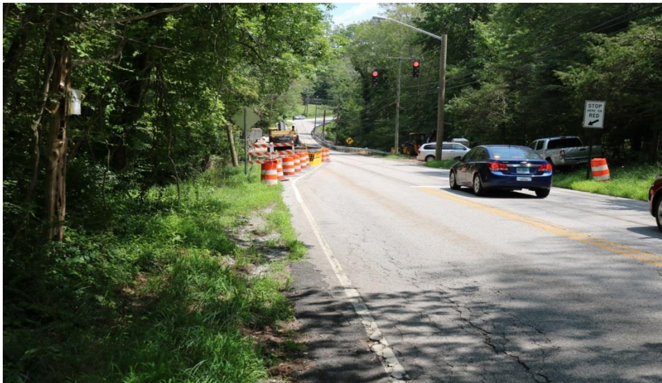
Photo 3: The temporary signalized one way traffic control system is well suited for the project and working well.
