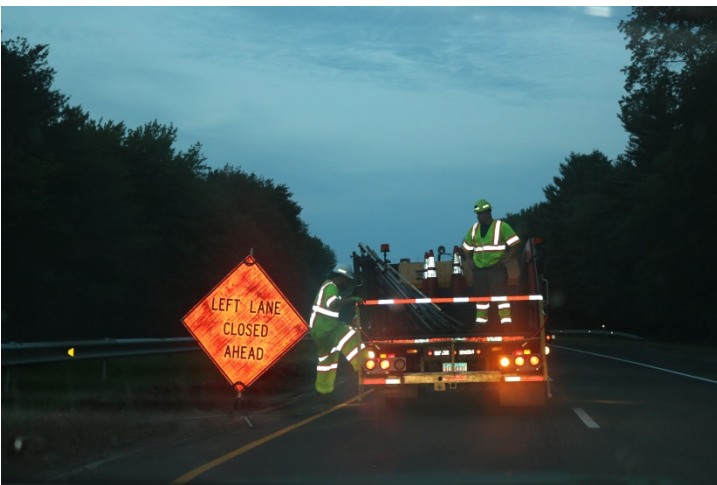
Route 15 NB: The next sign to state LEFT LANE CLOSED AHEAD posted only on the left side of the roadway.
