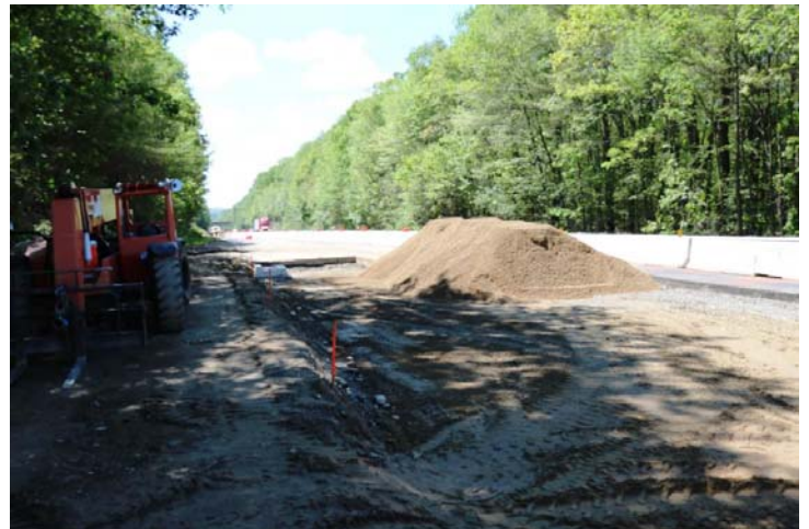
I-395: The work zone is protected by TPCBC. Material, as shown, is stored behind the barrier.
