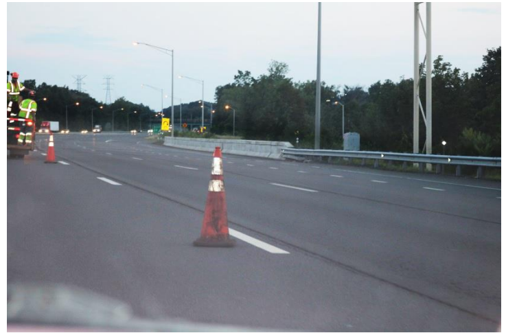
I-91 SB: The cones being used are 36 inches which is the minimum required height for Maintenance projects. However, the quality of the cones is marginal with a number of scuff marks and dirt on them.
