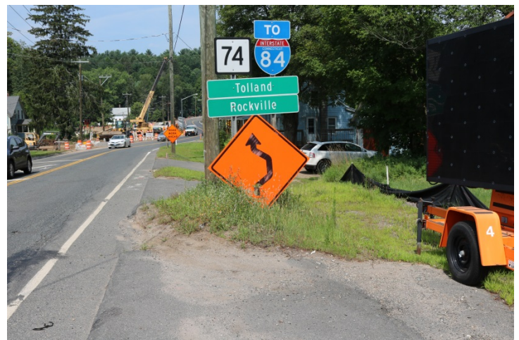
Route 74 WB: This reverse S-curve sign is posted on plywood which is an acceptable material but it is posted too low for motorists to see well.
