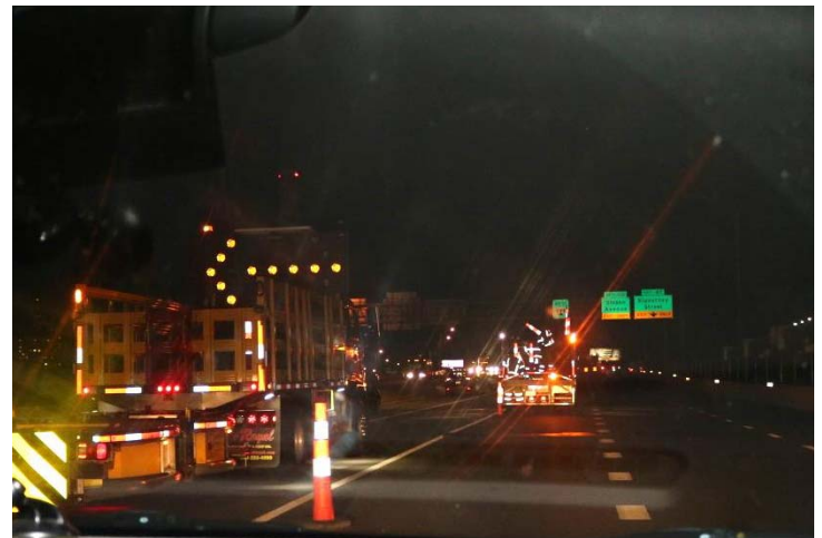
I-84 WB: A crash truck advising motorists to merge left was providing extra protection for the sign truck while the crew installed the devices for the tangent of the pattern.
