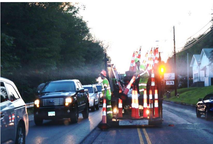
Route 63 NB: The sign crew placing cones while the SB side is shifted in a reduced lane.
