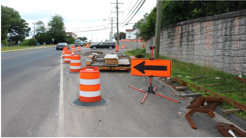
Photo 19: Another photo of equipment and materials stored too close to the travelway.
