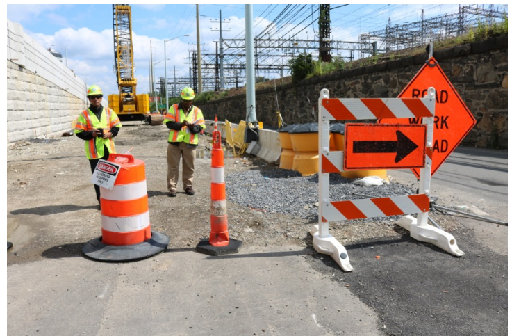
The barricade has an arrow sign on it directing traffic to proceed to the right around the barrier. The leading end of the barrier has an impact attenuation system to protect it.
