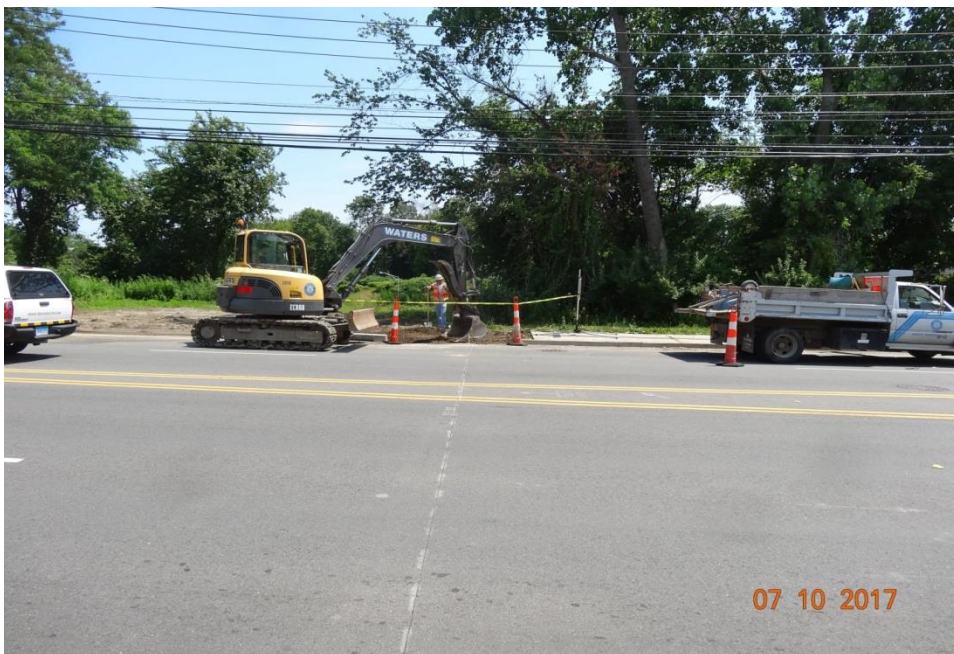
Photo 6: This is a photo of the work zone area (see photo 5) from across the road. Here, the use of warning tape helps better delineate the work area to construction workers and potential pedestrians, bicyclists, etc....
