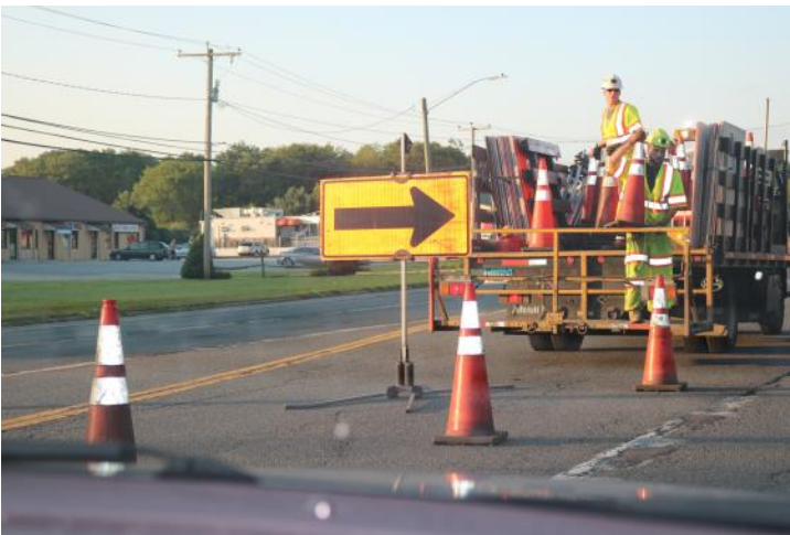
Route 6 EB: A temporary arrow sign is installed to direct traffic to merge right. According to the Work Zone Guidelines for Maintenance Operations, the sign should be a high mounted internally illuminated flashing arrow.
