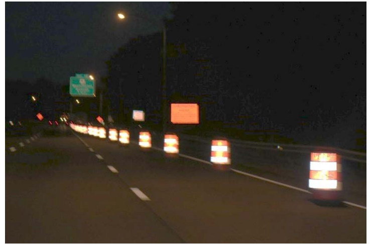
I-91 SB: The liability sign for the project is posted after the start of the pattern not before the advance warning signs closer to the project limits.
