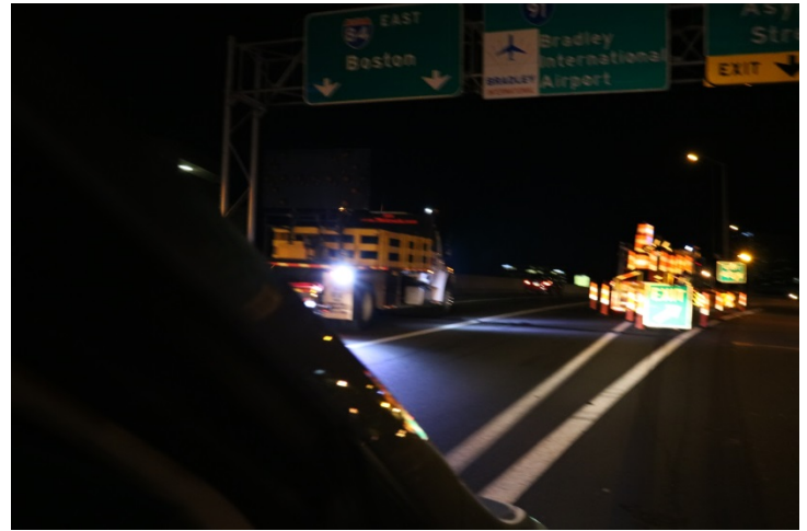
I-84 EB: The pattern leads up to an exit and a temporary exit sign is placed in the closed lane.
