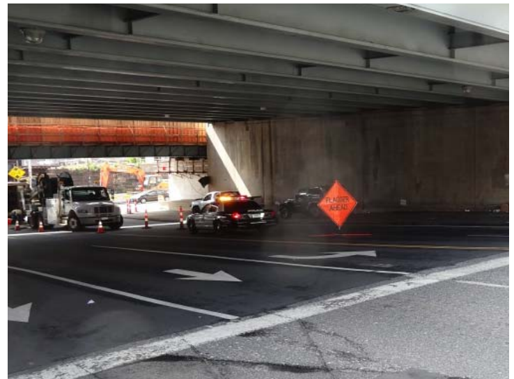
Atlantic Street: There is a “Flagger Ahead” sign placed just before the utility work area, however, there is no flagger just a municipal police officer.
