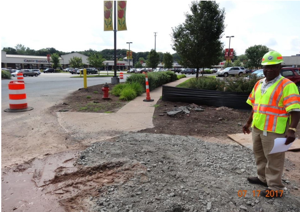
Photo 6: Here a cone was used to shut down a sidewalk. A sign (sometimes accompanied by a barricade) should be used to close a sidewalk and inform sidewalk users that the side walk is closed. In addition, if a sidewalk is shut down a temporary or detoured sidewalk route needs to be established.
