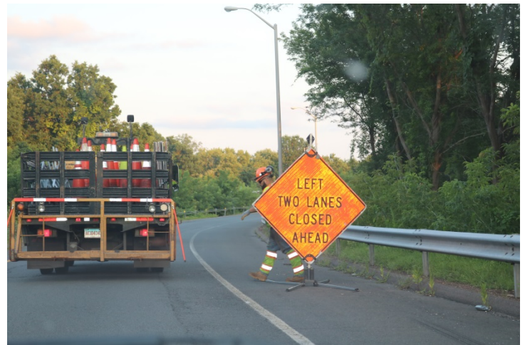
I-91 SB Exit 25: A LEFT TWO LANES CLOSED AHEAD sign on the ramp.
