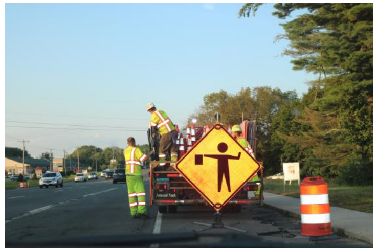
Route 6 EB: Although the project is using State Police for awareness and to direct traffic, they place a flagger sign to make people aware of trafficperson ahead.
