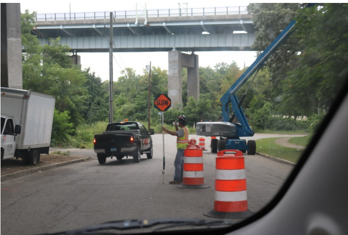
Crystal Avenue: A flagging operation is set up to assist with the alternating traffic pattern.
