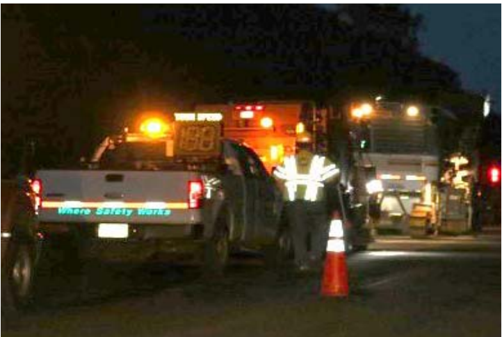
Route 15 NB: The Contractor's truck is placed in the pattern. It has a speed trailer mounted on it to help calm traffic.
