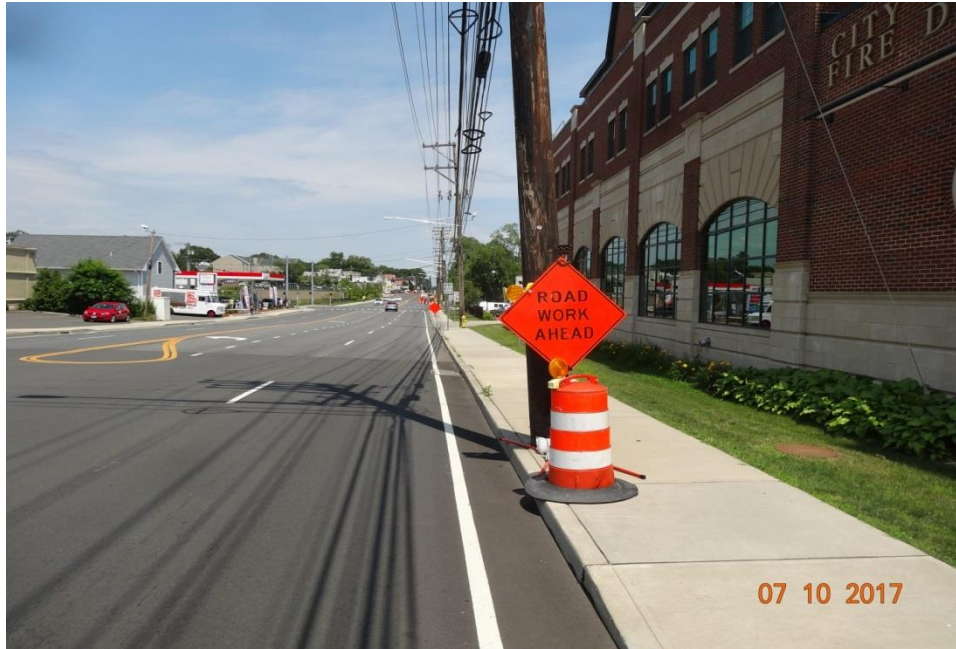
Photo 3: More lead in signs, northbound, Route 1, approaching the work zone. Although there appears to be enough room for pedestrians to pass, a minimum width of 36 inches is required. Also, the attached flashing warning lights are not crashworthy compliant. The Contractor may submit a certification of crash tests to be approved if they are going to be used on portable signs and barrels. If struck by vehicles the lights could become detached and become projectiles.
