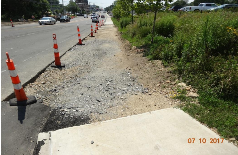
Photo 7: Looking south on Route 1. This sidewalk section is being reconstructed. When reconstructing existing sidewalk areas, the existing condition and functionality must be maintained or improved while the new sidewalk is being built unless a pedestrian detour is provided. The temporary condition of this sidewalk may not be adequate for some pedestrian groups.
