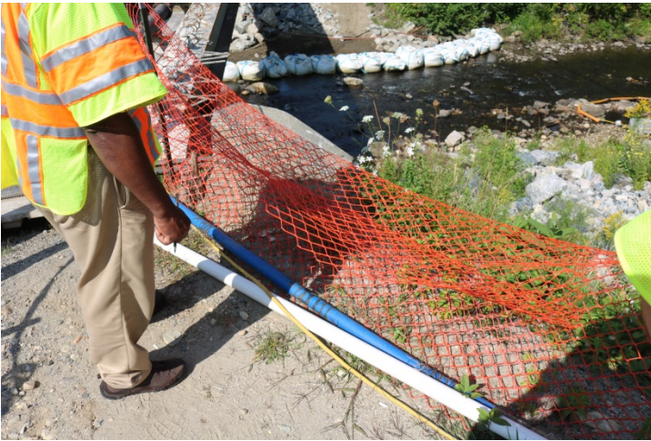
The project closes access to the bridge by securing this construction fencing in front of it.
