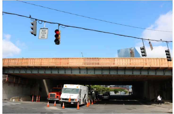
Atlantic Street: Utility work is in the left southbound lane. Traffic cones are used to close the lane and municipal police are assisting with traffic control.
