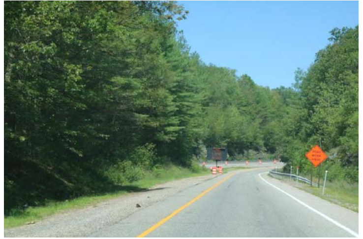
I-395 NB, Exit 94 On-Ramp: A post-mounted ROAD WORK AHEAD sign with barricade warning light and a Changeable Message Sign.
