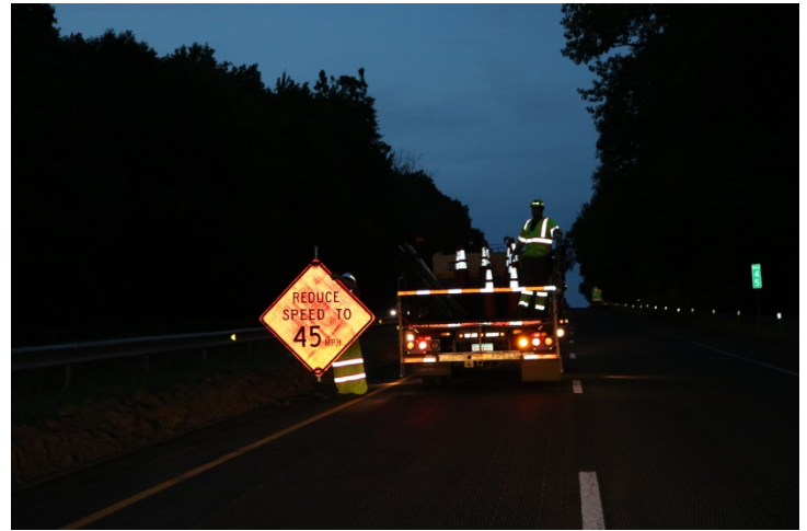
Route 15 NB: The Contractor still uses the REDUCE SPEED TO 45 MPH signs which are a good traffic calming device.
