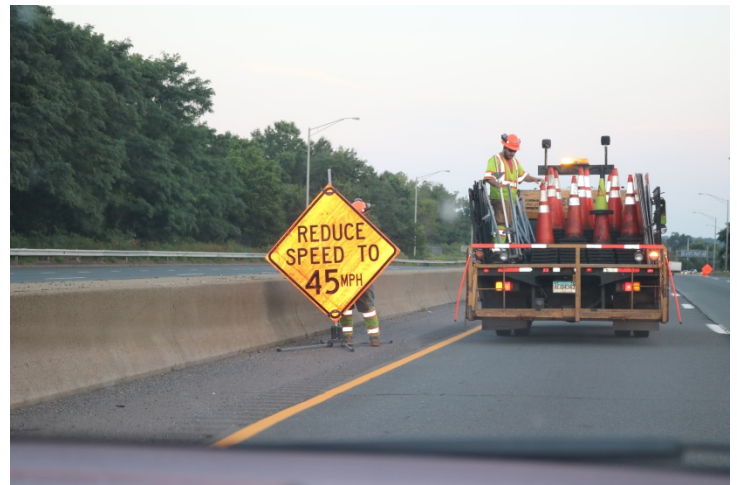
I-91 SB: Maintenance uses the REDUCED SPEED TO 45 MPH sign which have been discontinued by CTDOT Traffic Engineering for construction work zones because it is deemed not enforceable by law.
