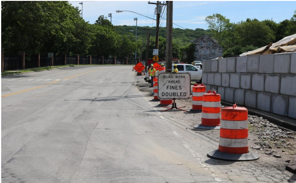
Photo 6: The space for lead in signs is limited at the beginning of Crystal Lake Road heading east. The Contractor did a good job spacing and arranging the signs to alert motorists of a road work area ahead.
