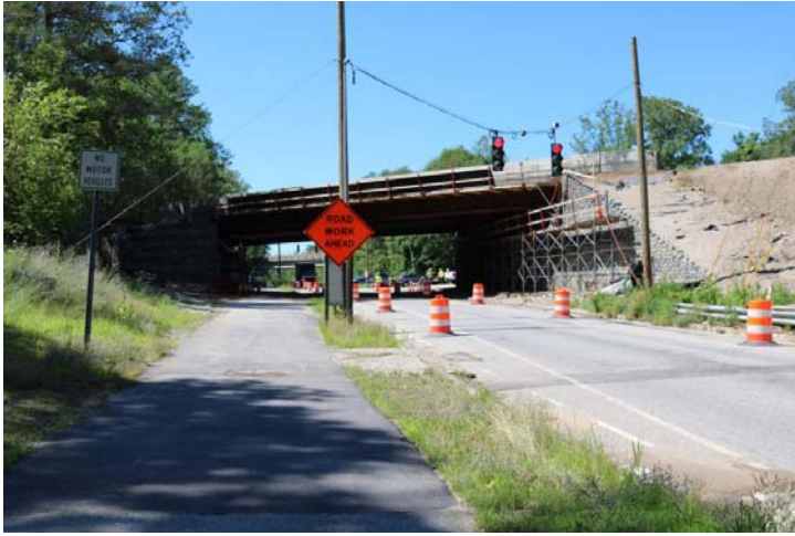
Tracy Road: This is the work zone as a motorist approaches from the west side. There is the temporary signal above, traffic drums closing the shoulders and closing the eastbound side. The ROAD WORK AHEAD sign is for the multi-use pathway.
