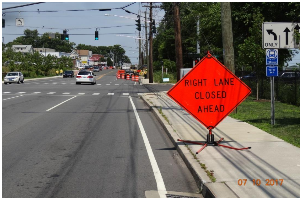
Photo 4: This lead in sign, Route 1, NB is partially blocking the sidewalk. The sign should be moved to the right and placed just on the edge of the grassy area.
