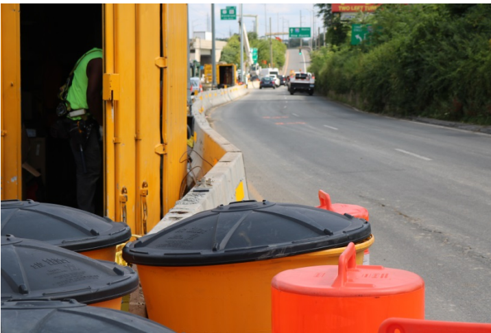
South State Street: The alignment of the TPCBC is skewed preventing divergent vehicles to be directed back to the roadway if impacted.
