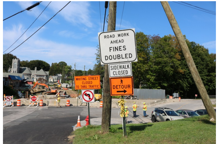
On Holabird Avenue just before the road closure signs are posted stating "Fines Doubled", "Sidewalk Closed", pedestrian detour, and "Whiting Street Closed to Thru Traffic".
