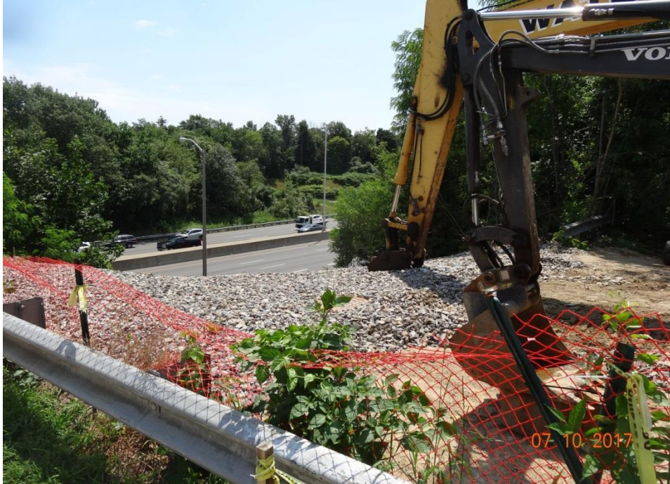
Photo 11: This is an area just off Route 1 where drainage was installed and tied into the drainage system along I-95, SB. The pre-existing condition included a guiderail that provided a barrier between the top of the slope and the I-95 right of way. A fence, temporary concrete barrier or Type 3 barricades should be installed, matching or bettering the system that was there before construction to keep workers, pedestrians, and vehicles from driving or walking and possibly falling down the slope into the right of way to I-95.
