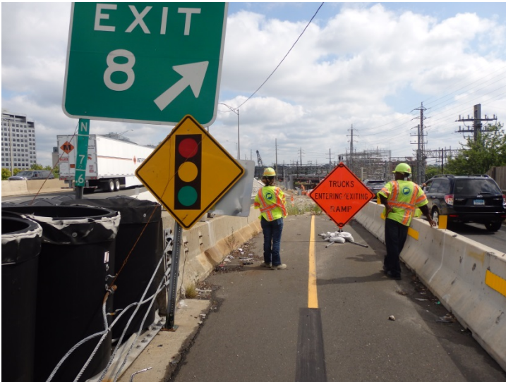
I-95 Exit 8 Off Ramp: There is a temporary signal sign right when a vehicle exits the highway. The impact attenuation system is in disrepair and needs to be attended to.
