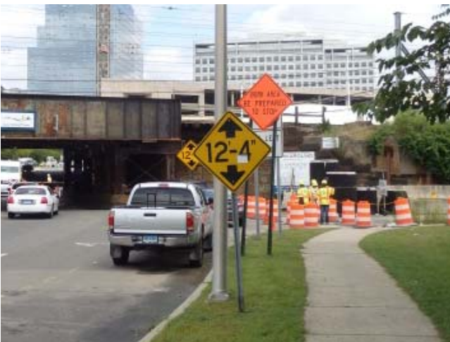
Atlantic Street: A post-mounted sign before the work zone stating "Work Area, Be Prepared to Stop".
