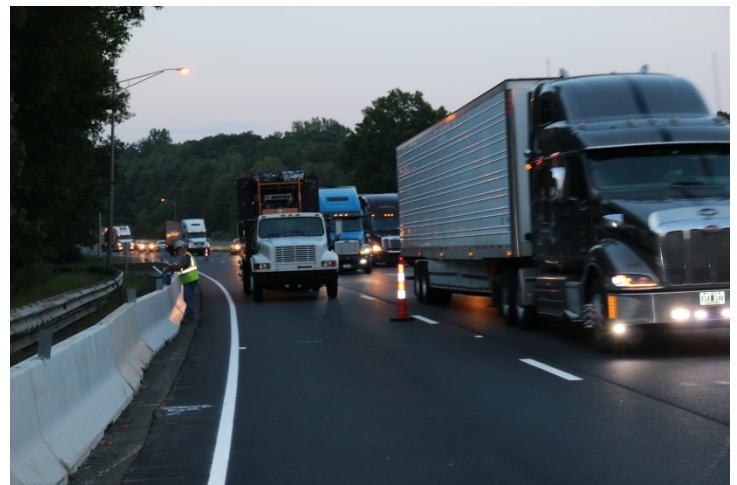
I-91 SB: A crash truck with a flashing arrow is placed in the closed lane.
