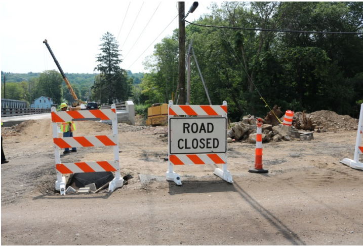
Barricades with ROAD CLOSED signs on front close the entrance to the new bridge.
