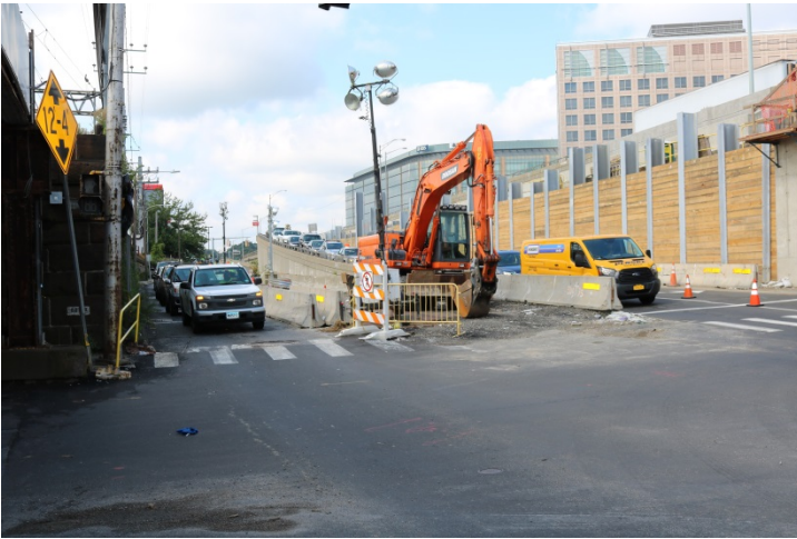
South State Street and Exit 8 Off Ramp: There is TPCBC and Type III barricades to close off the work area in between.
