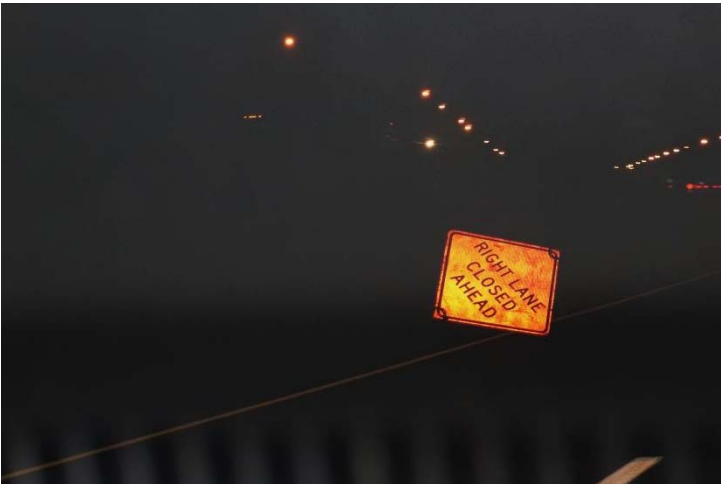
I-91 SB: A construction sign was knocked over after traffic was let through.
