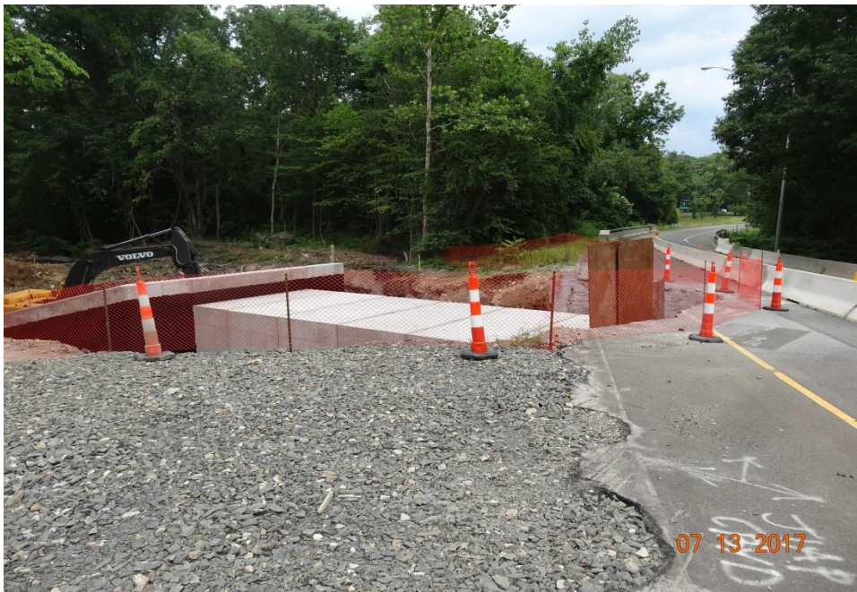
Photo 4: Fencing and cones are used here to delineate and protect the excavated area while the precast tunnel sections are being installed.
