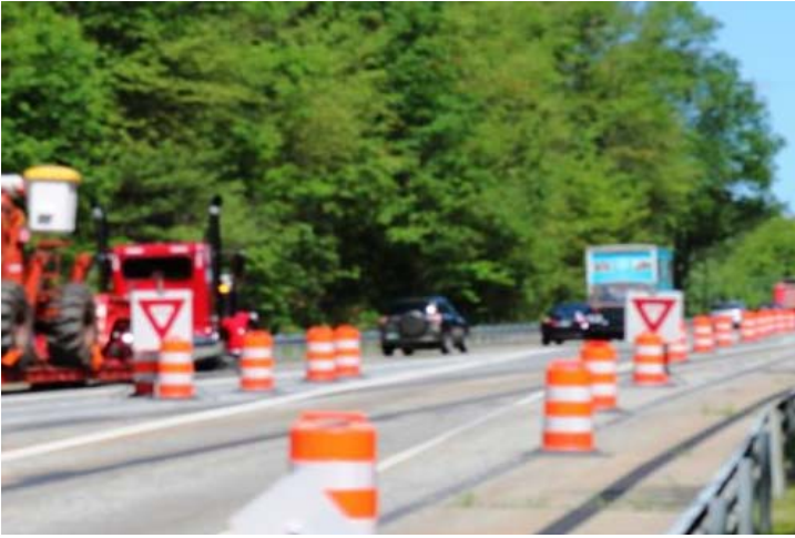
I-395 NB, Exit 94 On-Ramp: The yield signs added to the traffic pattern to help assist motorists merge onto I-395 with the lane closures.
