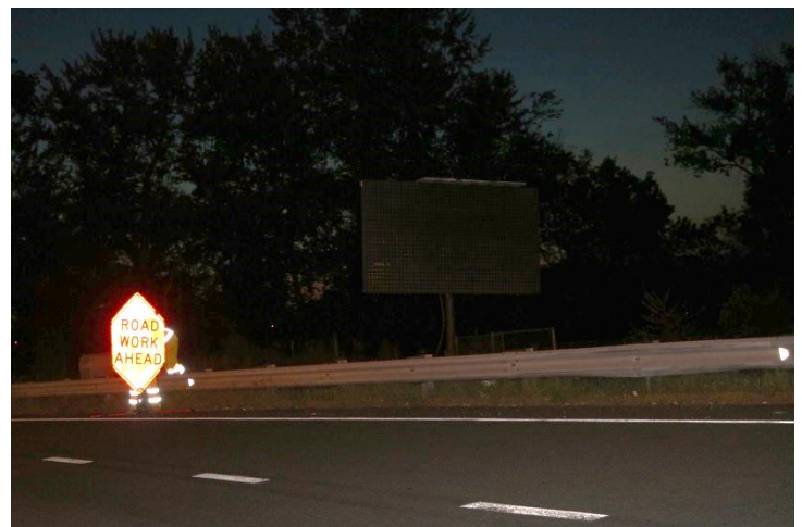
I-84 WB: The next sign is a ROAD WORK AHEAD sign with the sides cut down to keep it from infringing in the lane.
