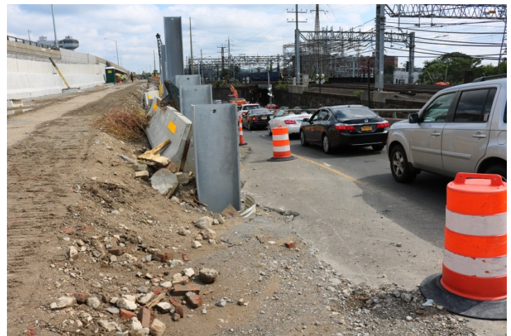
The edges of the H-piles used for the embankment support are unprotected and need to be protected as a blunt object.
