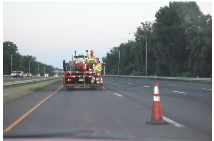
I-91 SB: The far left lane is closed and the tangential of the pattern is being installed.
