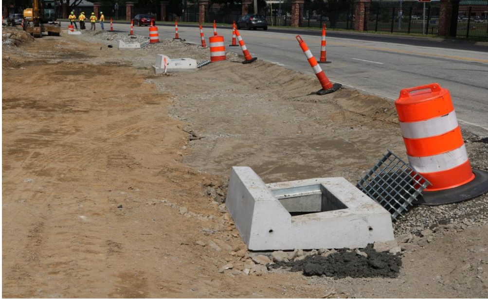
Photo 11: These new basins being set are within the 16 foot clear zone and are protruding high enough above the surrounding ground to create a potential hazard to motorists if left like this overnight. The drop-off is rather abrupt and too close to the travel way once the pattern is taken down. And although these basins had been worked on earlier, the grates were left off of several of them while they were not being worked on. If the basin is left unattended the grates or some other protection should be placed over the opening.
