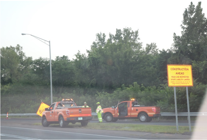
I-91 SB: A legal sign post-mounted for the project after the advance warning. The Maintenance vehicles block oncoming traffic while the sign crew installs the pattern.
