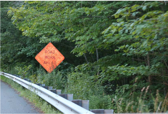
Route 63 NB: The post-mounted ROAD WORK AHEAD sign is worn with heavy smudges. This sign is in unacceptable condition and needs to be replaced.
