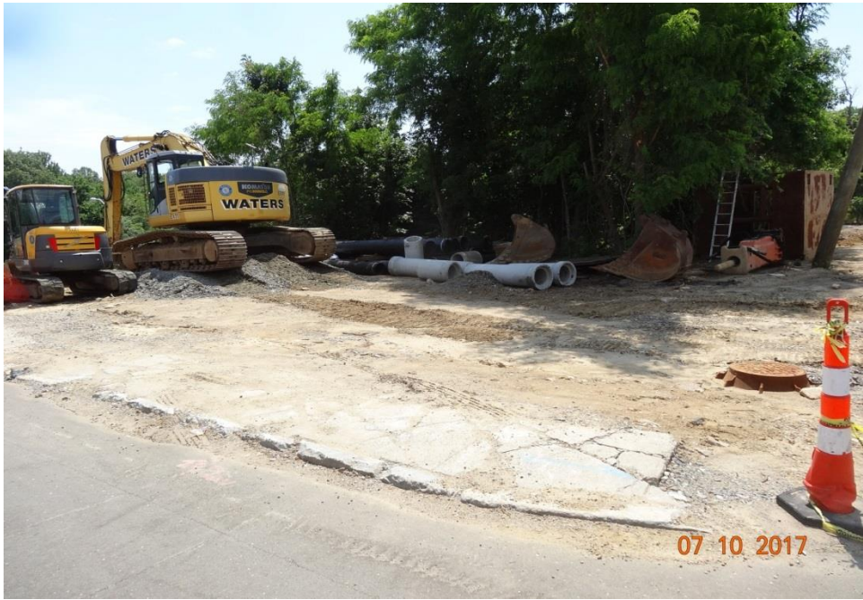
Photo 14: Same area as photos 11, 12, and 13. This is an area where equipment and materials are stored for use on the project. Everything here, except the small backhoe noted in Photo 13, is stored well outside the required 16 foot clear zone.
