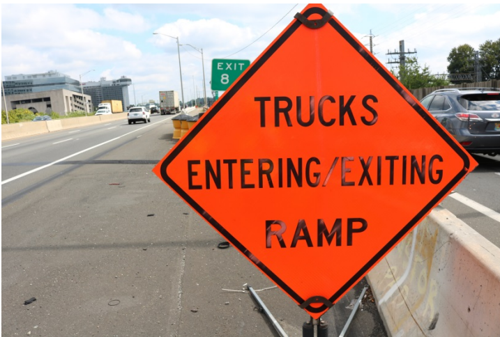
I-95 Exit 8 Off Ramp: There are construction signs informing motorists that trucks may be entering/exiting the ramp.
