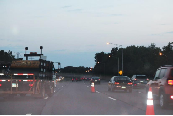
I-91 SB: The RRB finished at 8:08 PM when the full pattern was installed allowing the traffic to proceed through.
