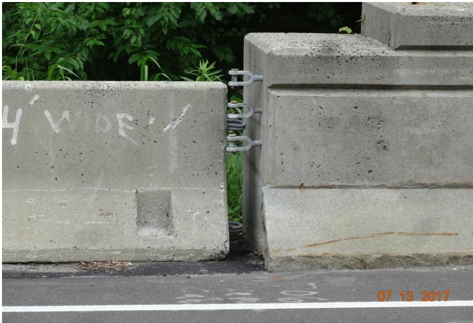
Photo 10: A temporary connection was not made where the temporary concrete barrier meets the bridge parapet on the north side of the connector ramp from 15 S to 25 N.
