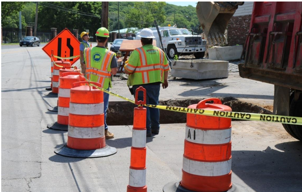
Photo 10: Here is the same area after the Contractor made some adjustments. The area is now well delineated and prevents a potential clear pass-through by pedestrians or others passing along the edge of the roadway.
