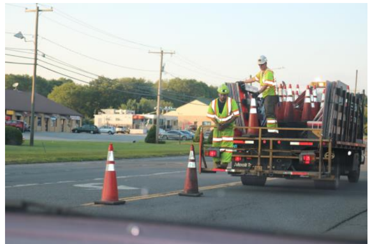
Route 6 EB: The taper for the pattern is started. The traffic cones are 36 inches in height.
