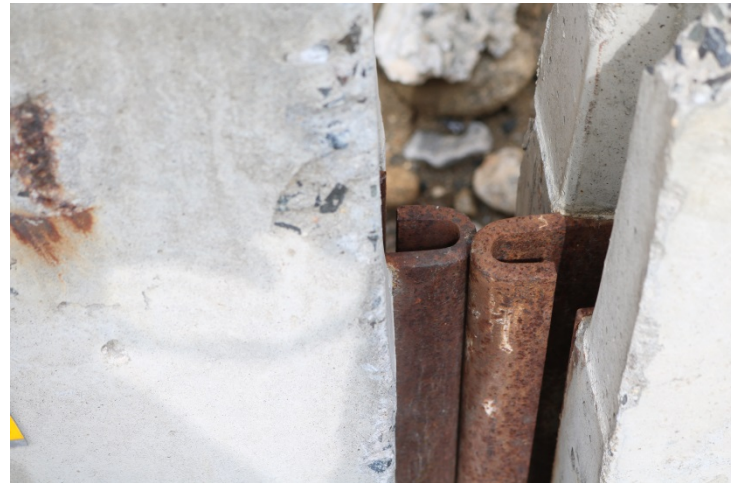
The sections of the TPCBC aren't connected at their joints. If impacted, a vehicle could displace a section and hit the blunt side of another.
