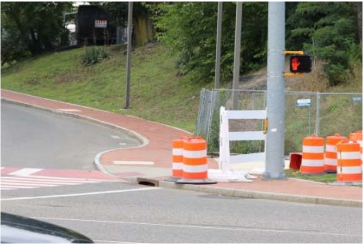
Atlantic Street: Type III barricades and traffic drums were used to close the sidewalk on the west side of the street.
