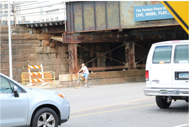
Atlantic Street: A bicyclist is proceeding through the work zone with traffic.
