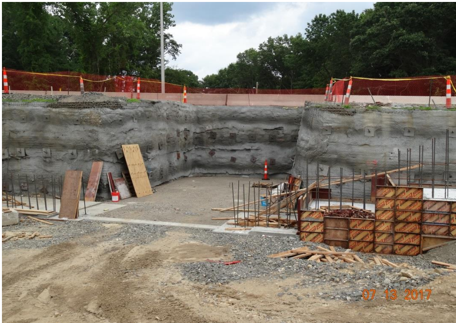
Photo 8: This is the second tunnel area being constructed to go under a connector ramp from Route 15 S to Route 25 north. Construction fencing and cones were used here also to protect and delineate the excavated area.
