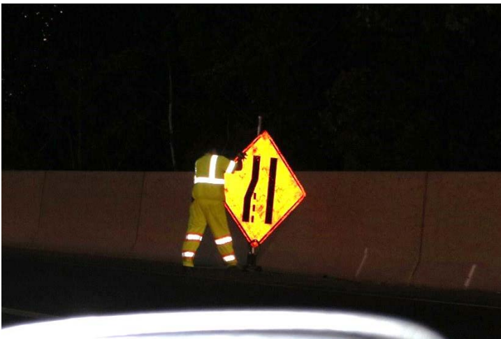
I-95 SB: The last sign to be installed on both sides is the merge right depiction.
