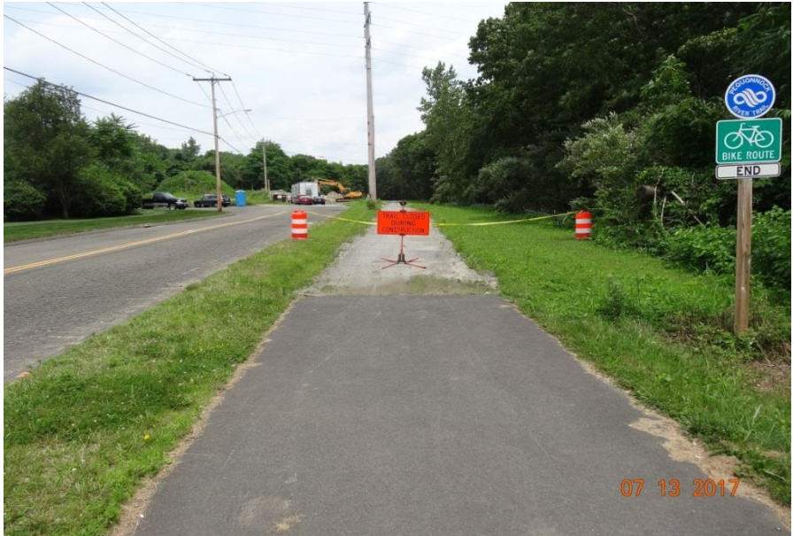
Photo 1: This is the “end” of the existing multi-use trail and the beginning of new trail construction. A sidewalk closed sign was installed. Type 3 Barricades were also put in place approximated 150 yards further down the new trail to help discourage vehicles from driving into the project site.
