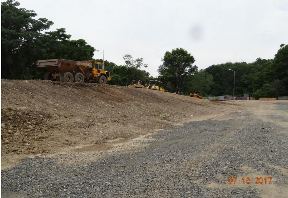
Photo 7: More storage. Lots of room.
