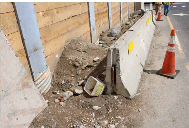
I-95 Exit 8 Off Ramp: The TPCBC is missing a section causing the exposed end to be a blunt end.
