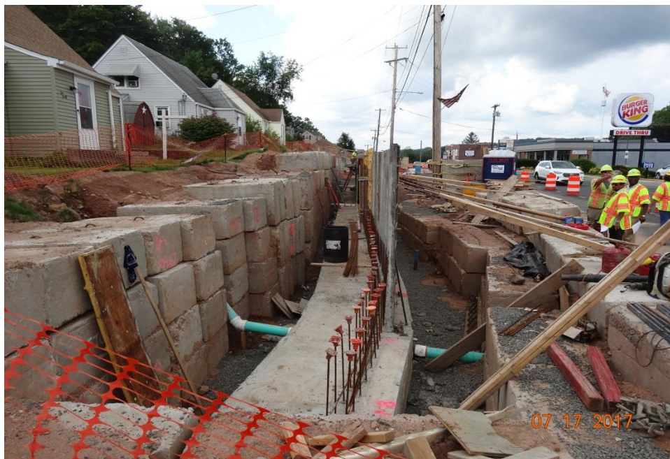
Photo 18: Here the Contractor has installed construction fencing around the back and sides of the excavated area to prevent anybody from walking into this potential hazard.
