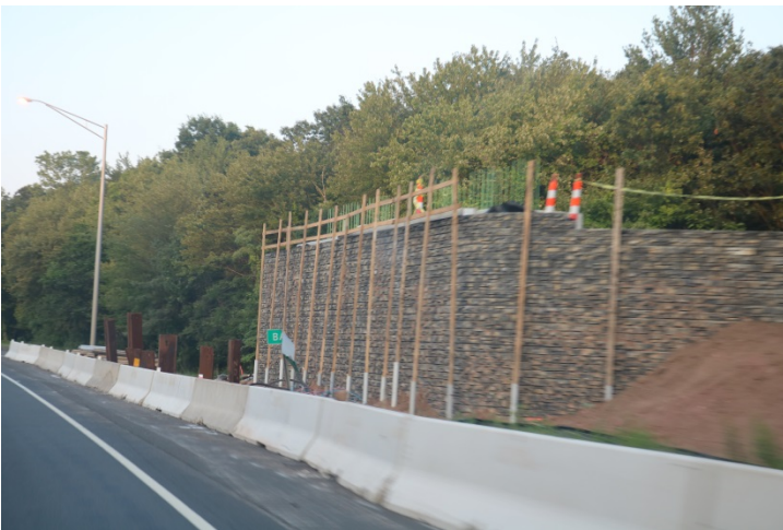
I-91 SB: The GRS-IBS abutment for the bridge on Bassett Road being replaced over I-91.
