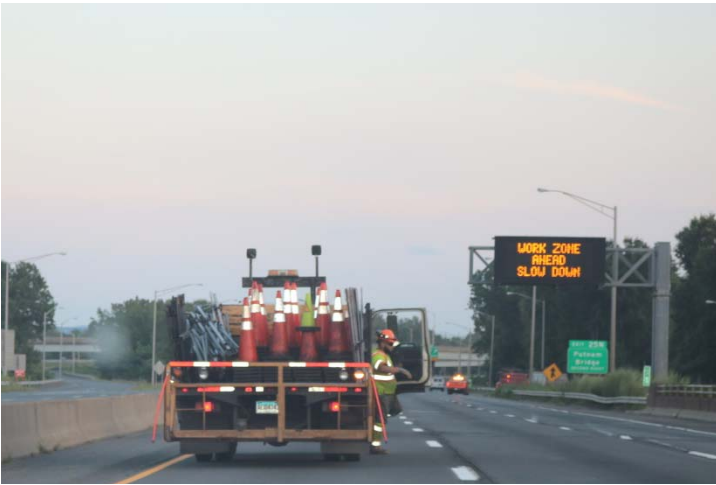
I-91 SB: A VMS overhead states WORK ZONE AHEAD SLOW DOWN on its first frame.
