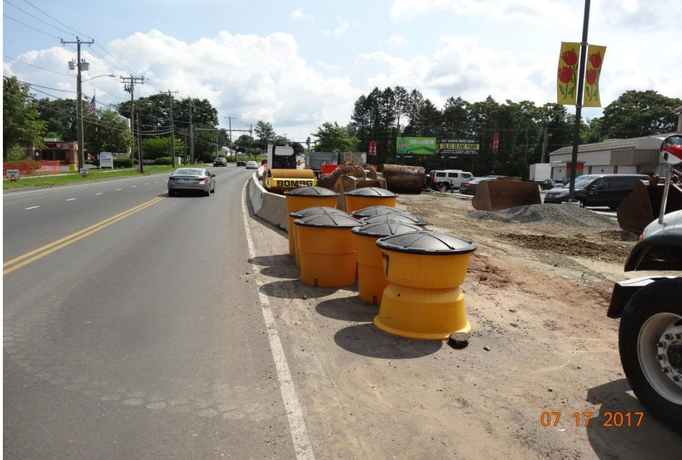
Photo 12: Shown here is an example of well stored equipment and materials behind temporary concrete barrier. The Inertial Drums should be delineated with Sign No. 50-5032.
