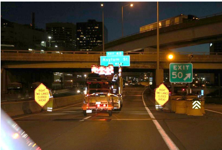
I-84 WB: The crew mounts signs on both sides of the roadway stating RIGHT TWO LANES CLOSED AHEAD.
