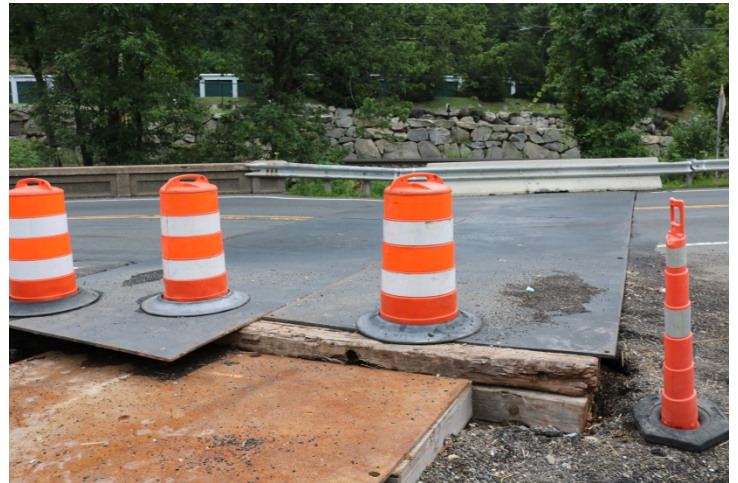
Route 7: The bridge which is being replaced. During the week the opening is covered with steel plates and edges are delineated with traffic drums.
