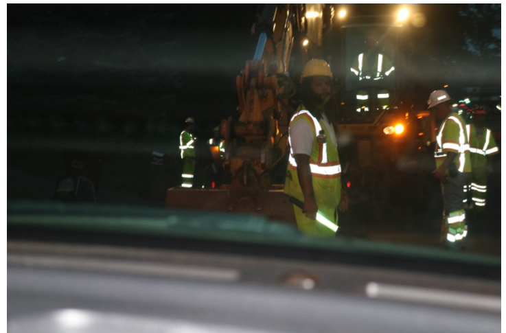
Route 63 NB: There's a uniformed flagger equipped with a traffic control wand is positioned at the work area to direct traffic around the operation.
