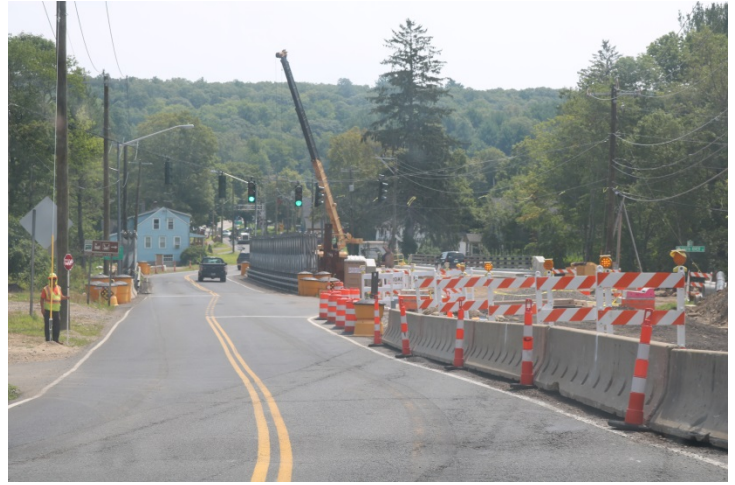
Route 74 EB (Tolland Stage Road): There is a flagger to stop traffic and allow construction traffic to enter and exit Route 74.
