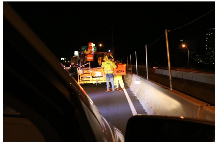
I-84 EB: An END ROAD WORK sign is mounted after the exit.
