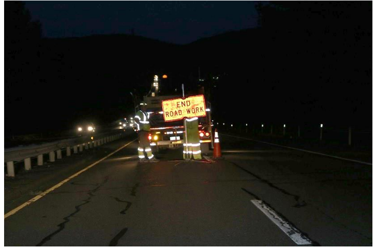
Route 15 NB: The last device placed was the END ROAD WORK sign.
