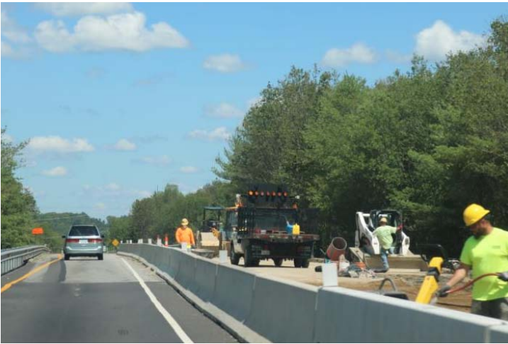
I-395 NB: The travel lane that’s open adjacent to the work zone. The work area has a flashing arrow showing a straight bar indicating the lane is closed.
