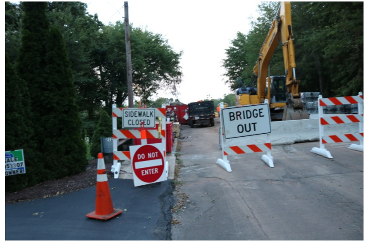
Bassett Road: The road leading up to the bridge is closed. There are signs posted on Type III barricades stating BRIDGE OUT and SIDEWALK CLOSED.
