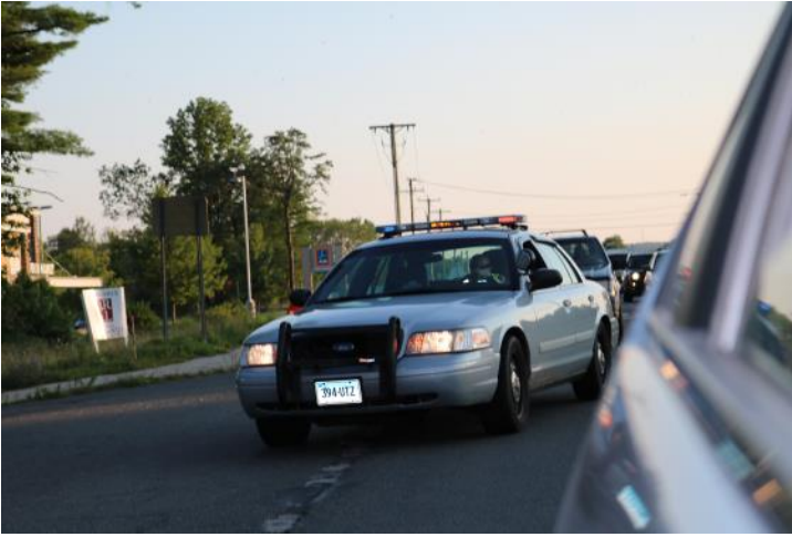
Route 6 EB: The project uses a Rolling Road Block while installing their traffic pattern.
