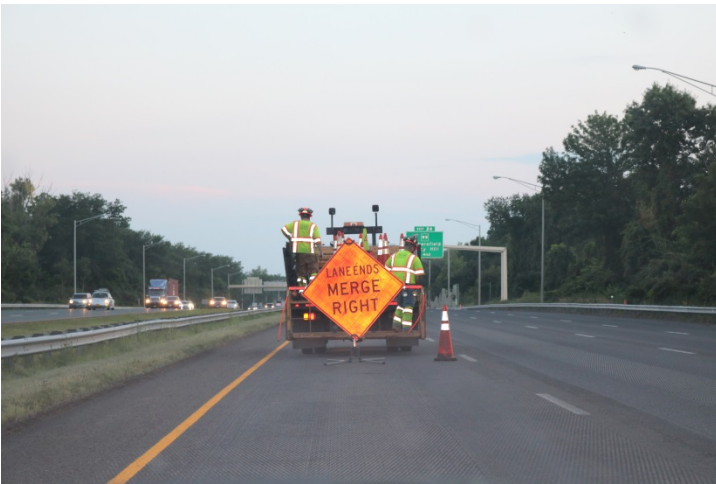
I-91 SB: A LANE ENDS MERGE RIGHT sign installed in the closed left lane before starting the taper for the center left lane.
