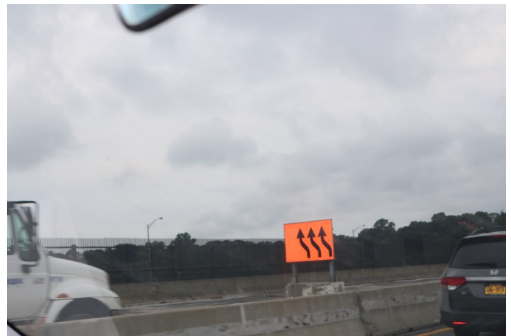
I-95 SB: After the work zone, a traffic shifted to the left sign is posted.
