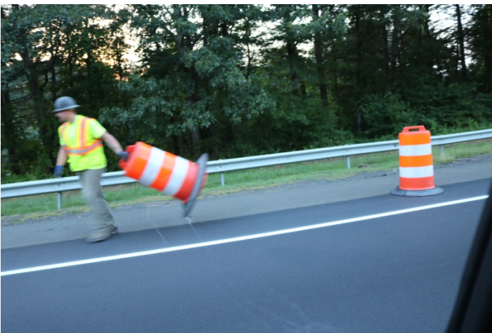
I-91 SB: The taper for pattern is being installed with the workers off the truck and a crash truck protecting the crew while on the road.
