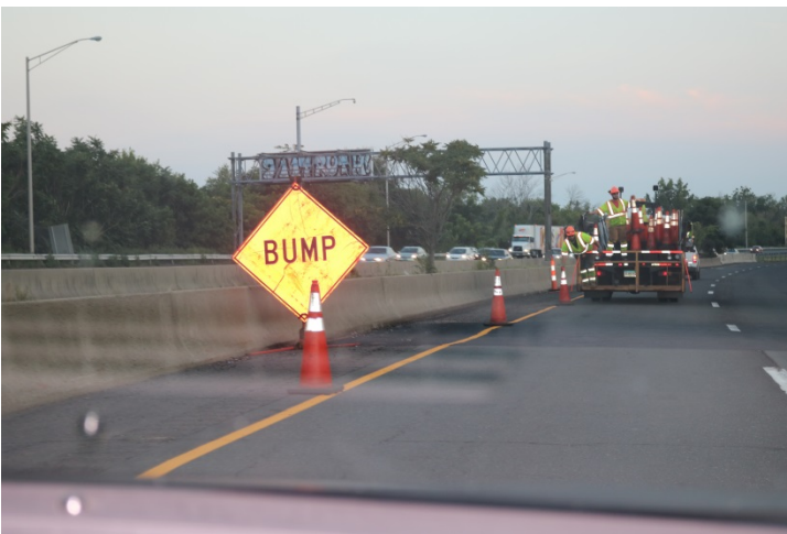
I-91: Another temporary sign installed for a semi-permanent condition.
