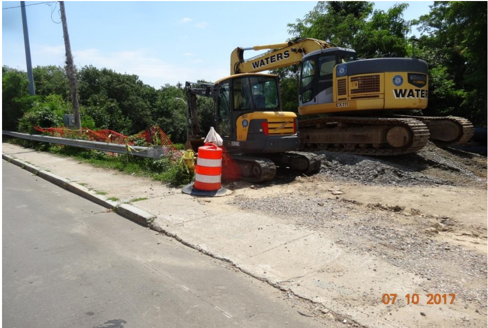
Photo 13: This is the same area as photos 11 and 12. An attempt to use equipment to block off the slope to I-95 has resulted in a potential clear zone hazard. All equipment and materials are to be stored a minimum of 16 feet off of the roadway.
