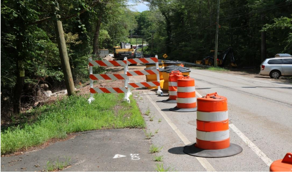
Photo 4: Type 3 Barricades are well placed to prevent any one walking down the road from wandering into the work area.
