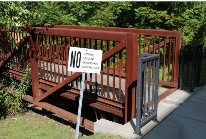
The pedestrian bridge that crosses the river on NCCC's campus is a part of the pedestrian detour.
