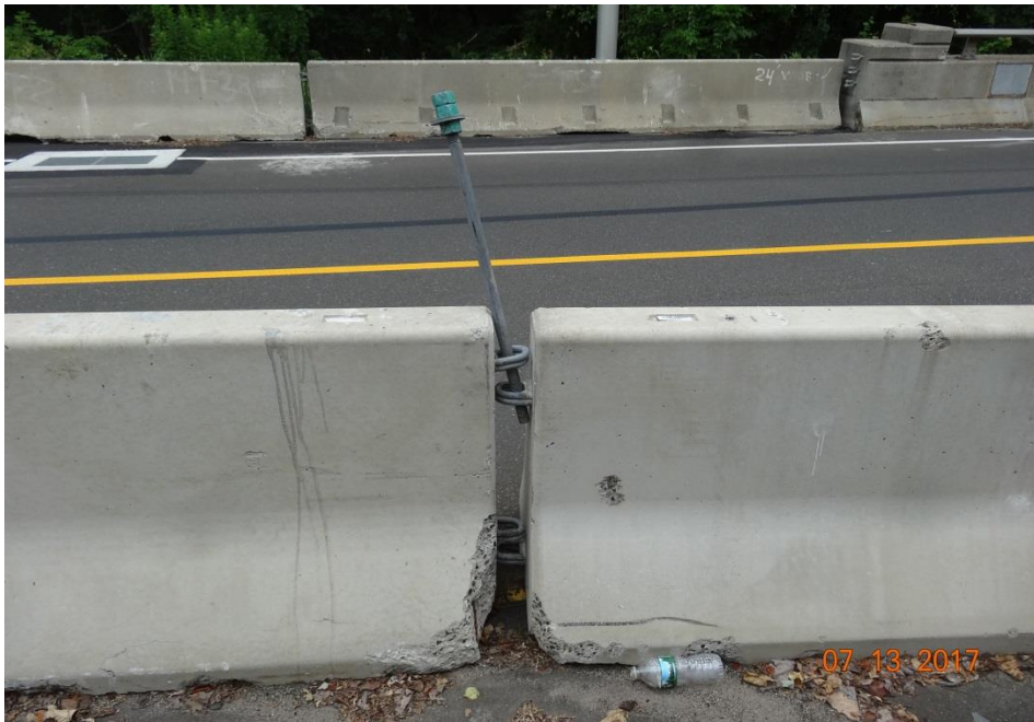
Photo 12: The connection rods for the temporary concrete barrier were not locked down with a threaded nut on the bottom of the rod.
