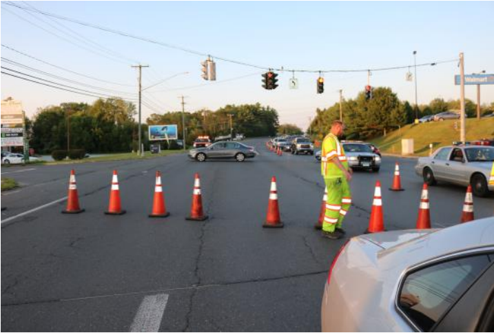
Route 6 WB: To prevent traffic from turning into the closed lanes, traffic cones are placed across the lanes at the intersection.
