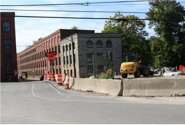
This is work zone behind TPCBC on Holabird Ave and Northwestern Connecticut Community College (NCCC) parking lot.
