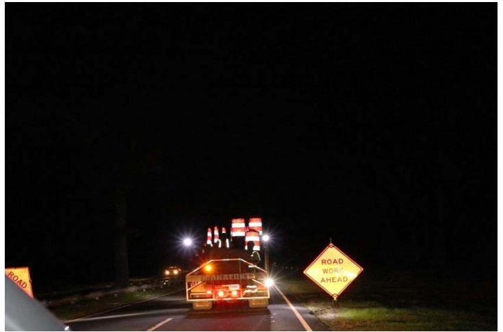
Route 15 SB: The first advance warning signs to be installed are ROAD WORK AHEAD on both sides of the roadway.
