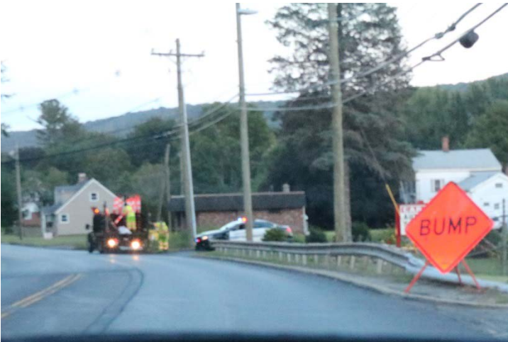
Route 63 NB: The temporary sign placed is to notify motorists of the BUMP in roadway.
