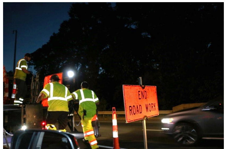
I-95 SB: Finally, an END ROAD WORK sign is placed at the end of the pattern only in the closed left lane.
