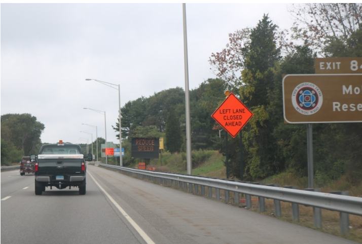
I-95 SB: Next is the LEFT LANE CLOSED and behind is a CMS stating "REDUCE SPEED" on its first frame.
