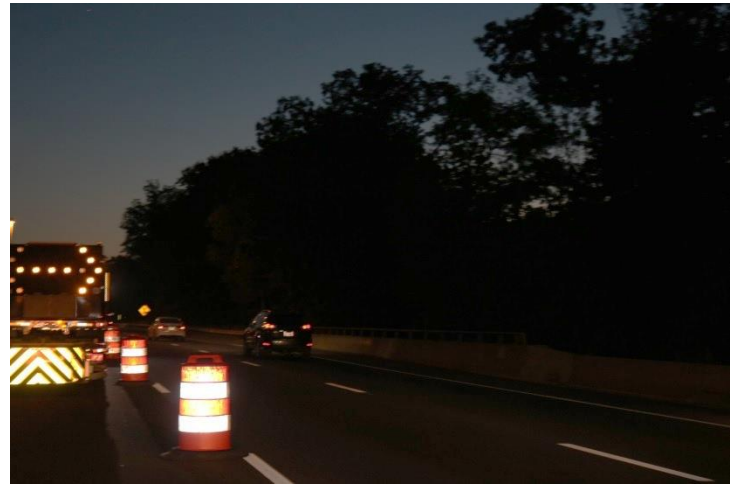
I-95 SB: Within the taper a TMA is parked with a flashing arrow directing traffic to merge right.
