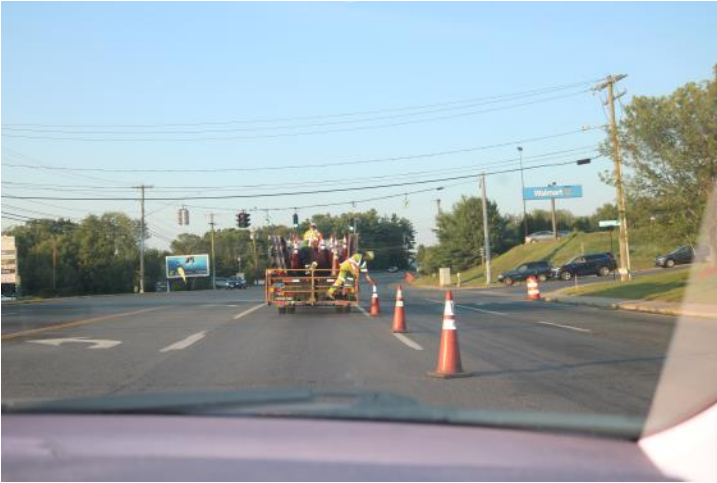
The traffic pattern is closing the WB lanes, shifting the WB traffic to the left EB lane and having all EB traffic into the right EB lane.
