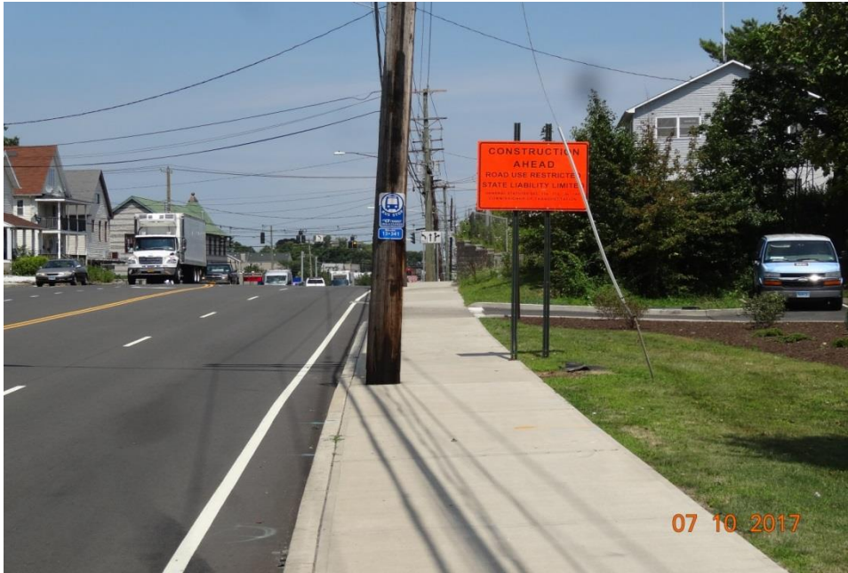
Photo 1: Photos 1 and 2 showing work zone approach signs along Route 1, north, mounted just at the outside edge of the sidewalk allowing enough room for pedestrians to pass.
