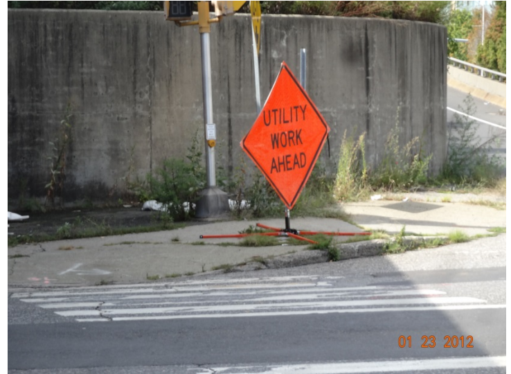
A construction sign stating “Utility Work Ahead” is used but it’s placed on the sidewalk blocking the path for pedestrians.
