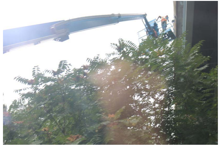
Crystal Avenue: A boom man lift is set up on the road to assist with work on the side of the bridge overhead.
