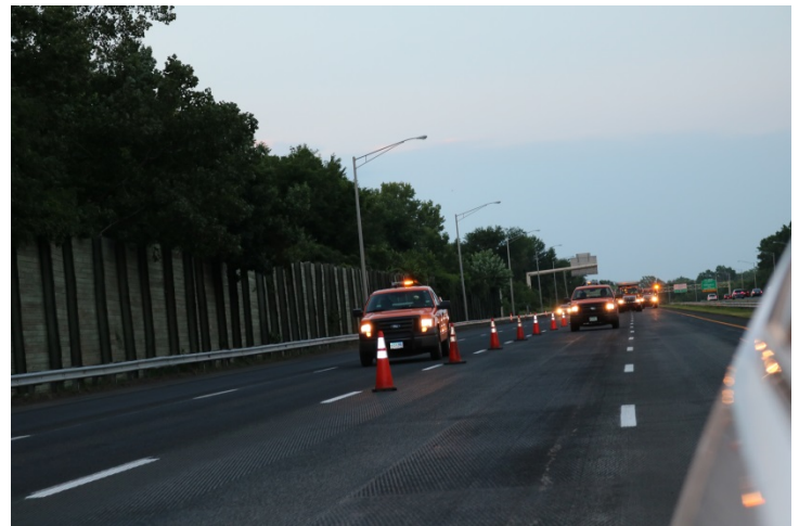
I-91 SB: Although the far two left lanes are closed, the Rolling Rod Block continues.
