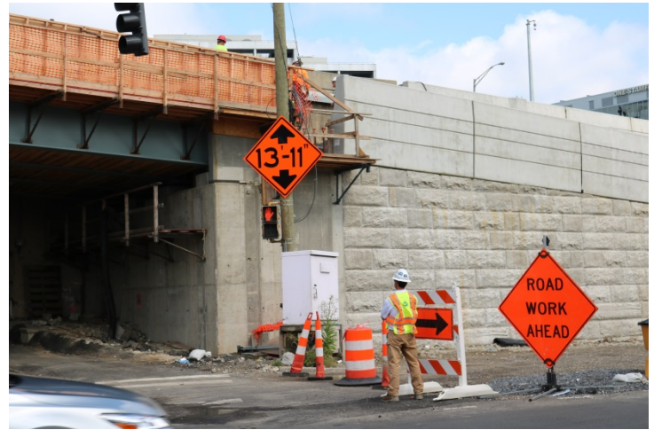
Atlantic Street: There is a construction sign advising the clearance under the new ramp. The entrance to the work area is closed with a combination of traffic cones, traffic drums, and a Type III barricade. There is a construction sign stating Road Work Ahead.
