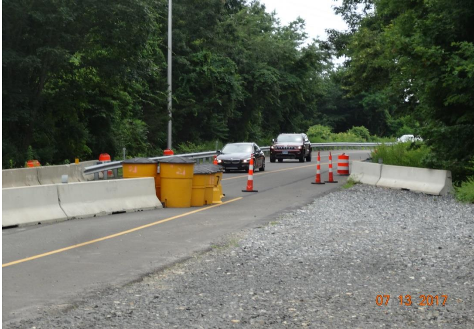
Photo 3: Route 25 South to Route 15 north connector ramp. Here, concrete barrier is installed to channelize and shift traffic to the southern half of the ramp. An opening was created to allow construction vehicles to enter and exit the work site.
