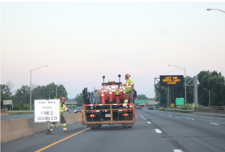
I-91 SB: The VMS's second frame states LEFT TWO CENTER LANES CLOSED . A FINES DOUBLED sign is installed only on the left side of the highway.
