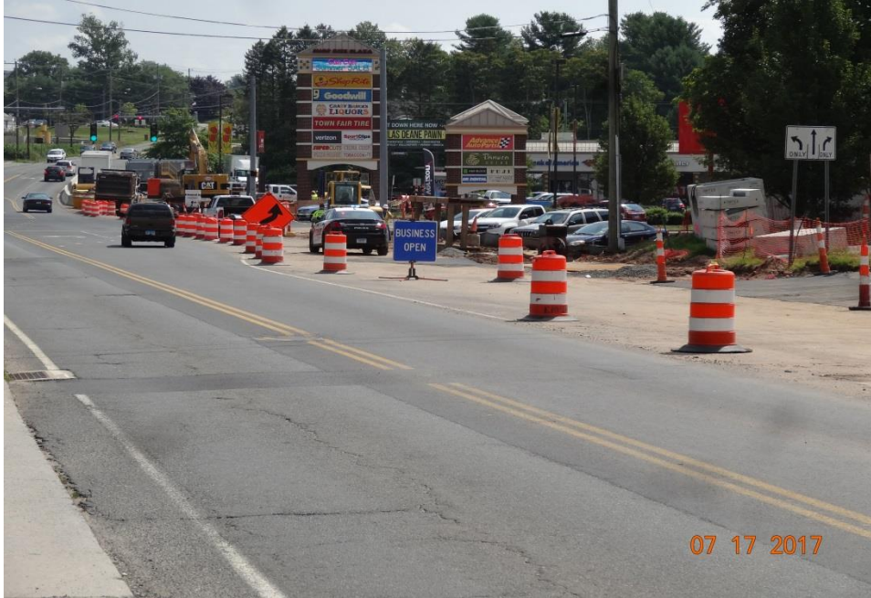
Photo 4: “Business Open” signs were well placed at several locations throughout the work zone.
