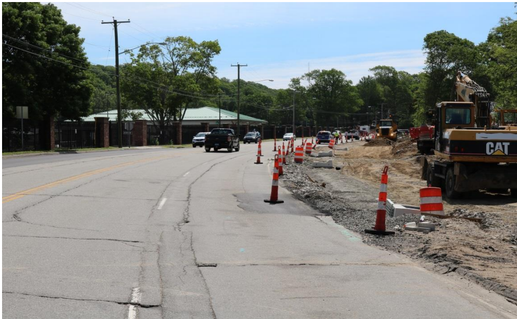
Photo 8: The taper to take the right lane was not well formed. As you can see from this photo, too many cones were left on the edge of the roadway. This muddles the delineation of cones as drivers approach the work zone. Any cones on the edge of the road should be removed from the vicinity of the taper to insure a clear sight line of tapered cones for traffic to follow.
