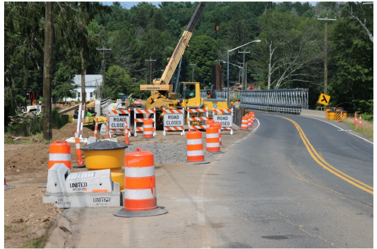
Route 74 WB: The work area with barricades closing the entrance to the new bridge and traffic drums delineating around it.
