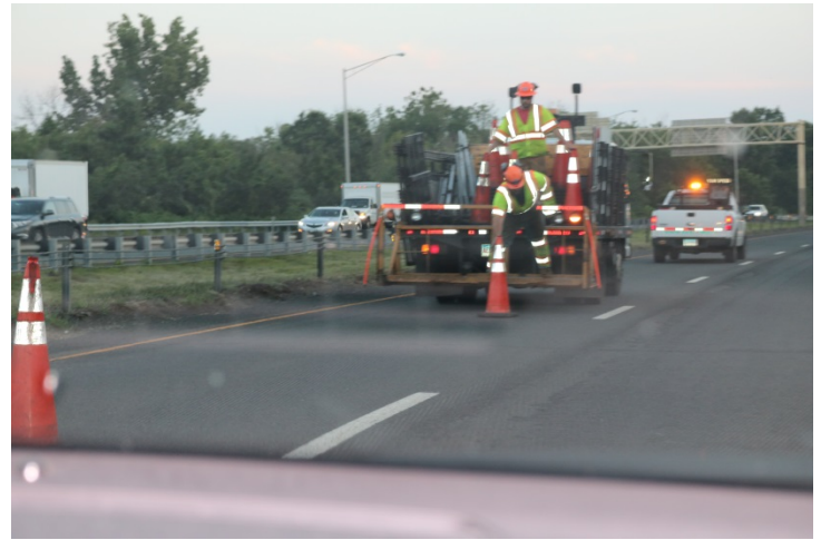
I-91 SB: The taper of the pattern being installed. The far left lane is closed.
