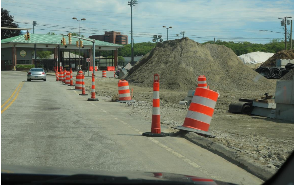
Photo 5: Military Highway access point to the Contractor's equipment storage and aggregate processing area.
