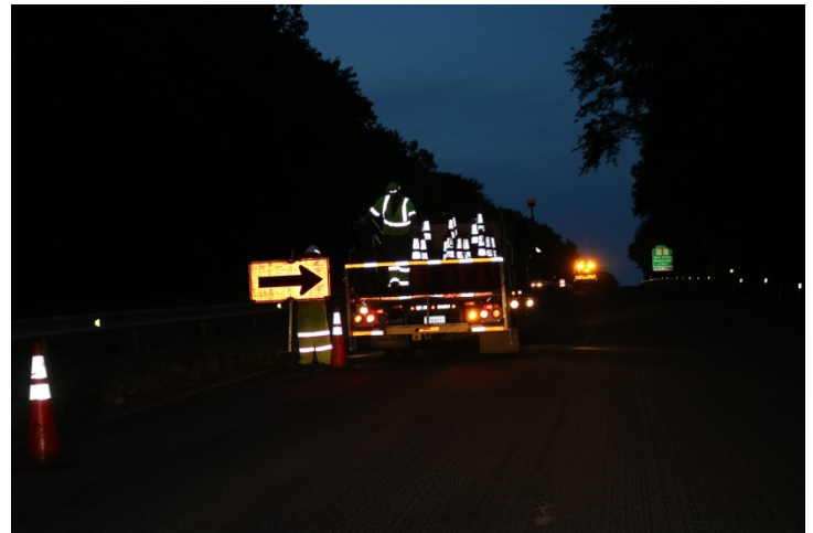
Route 15 NB: An arrow sign is posted instead of an internally illuminated arrow board.
