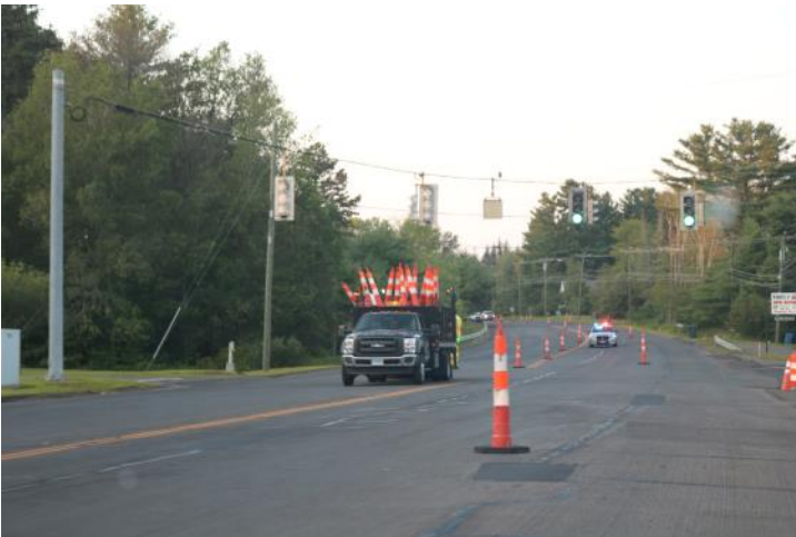
Route 6 EB: The sign crew placing the next row of cones to close the WB lane. The State Police is assisting.
