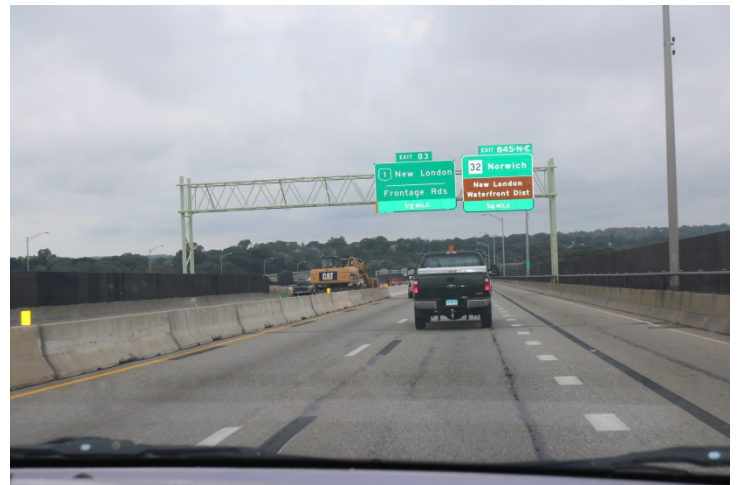
I-95 SB: The temporary pavement markings shifting the traffic right. However, the blackout paint doesn't match the color of the roadway.
