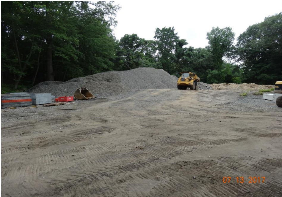
Photo 6: This is another equipment and materials storage area. Here the Contractor had plenty of room to set up a small crushing operation for the rock that was excavated from within the project.
