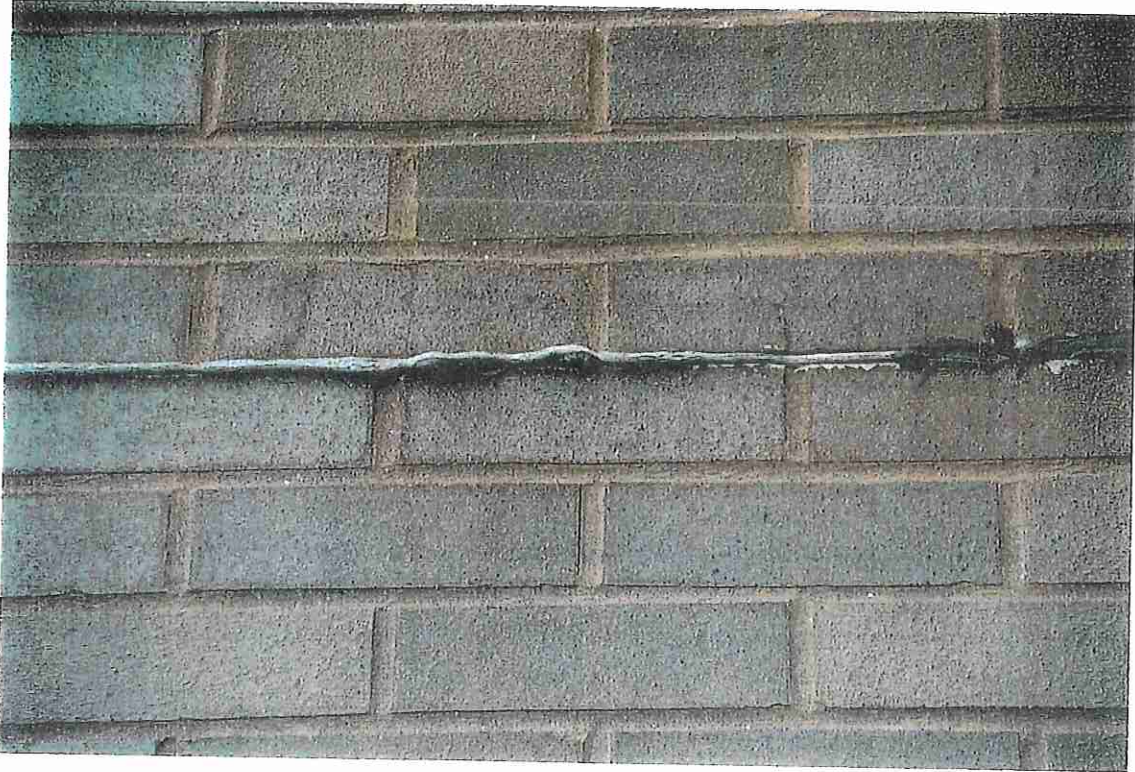
Photo No. 5 SEALANT AT SOFT JOINT BEING PUSHED OUT DUE TO THERMAL EXPANSION IN 16-4/2/98 BRICK VENEER.
