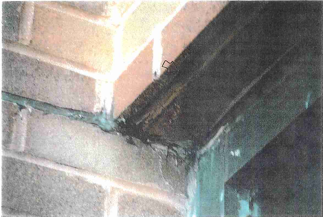
Photo No. 21 CLOSE-UP PHOTO OF WINDOW LINTEL. NOTE JOINT AT EDGE OF STEEL IS FILLED SOLID WITH SEALANT.
