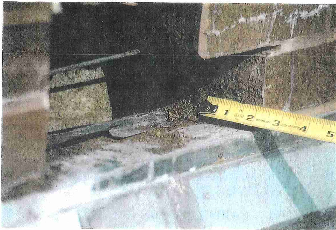
Photo No. 15 CUT NO. 2 - BASE OF PARAPET MAIN ROOF. NOTE FLASHING IS HELD BACK 12A-4/18/98 2" FROM FACE OF BRICK.
