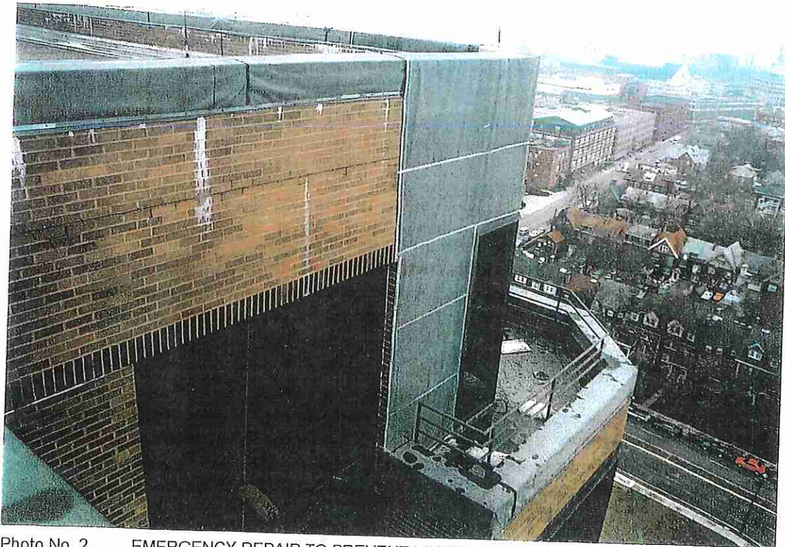
Photo No. 2 EMERGENCY REPAIR TO PREVENT LEAKS - FULLY ADHERED EPDM OVER COPINGS AND FACE OF WALL SECURED WITH TERMINATION BARS.
