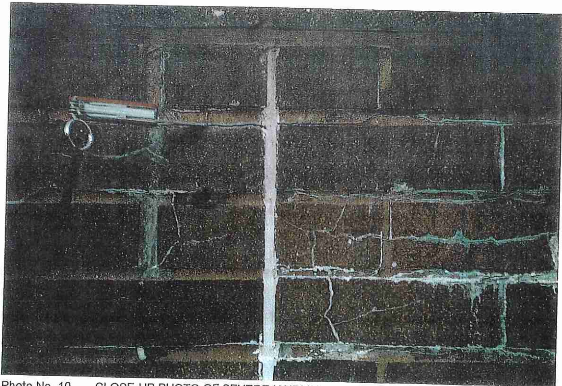
Photo No. 10 CLOSE-UP PHOTO OF SEVERE HAIRLINE CRACKING IN BRICK VENEER. NOTE DEFECTIVE MORTAR JOINTS.
