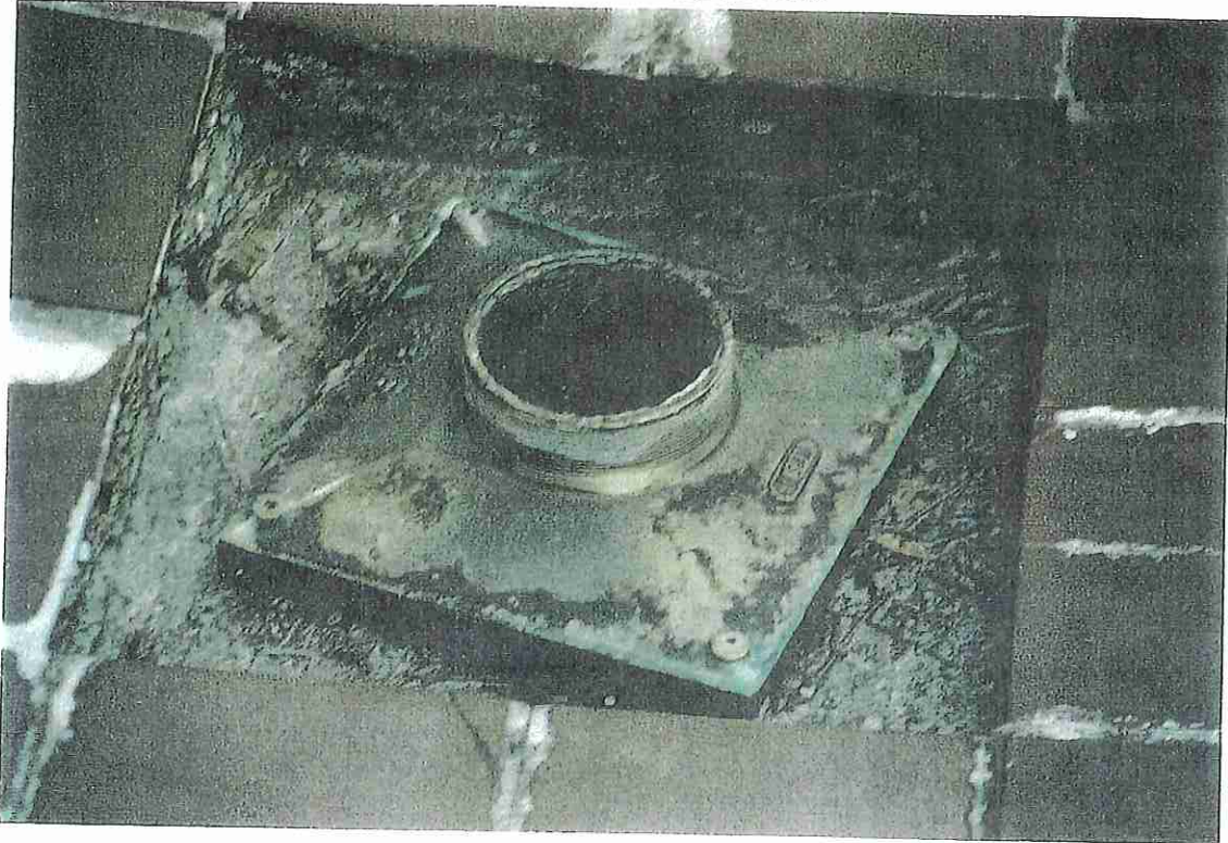
Photo No. 27 TYPICAL TERRACE DRAIN REMOVED TO ALLOW FOR DRAINAGE OF SUMP. NEW 13-4/2/98 DRAINS SCHEDULED TO BE INSTALLED LOWER.
