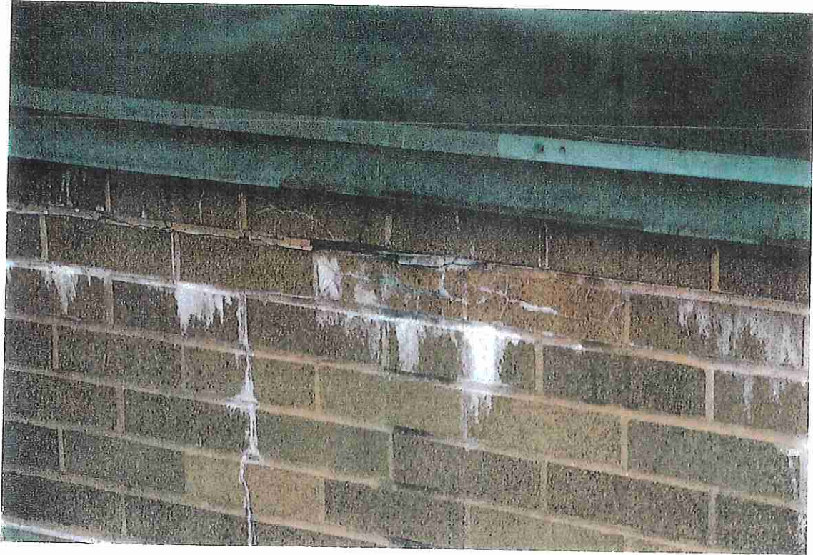
Photo No. 9 SEVERE EFFLORESCENCE DUE TO WATER INFILTRATION. NOTE DEFECTIVE MORTAR JOINT AND EPDM COPING COVER.
