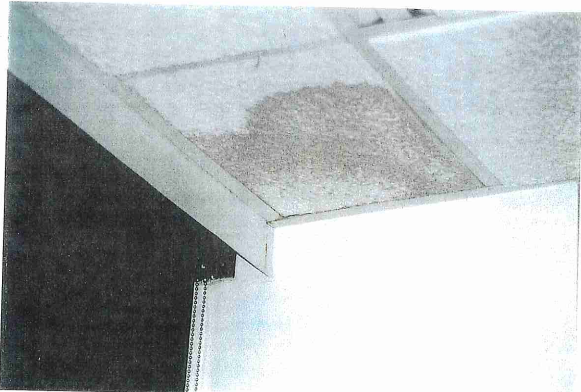
Photo No. 28 INTERIOR WATER DAMAGE AT WINDOW HEAD - 17 TH FLOOR. 18A-4/18/98
