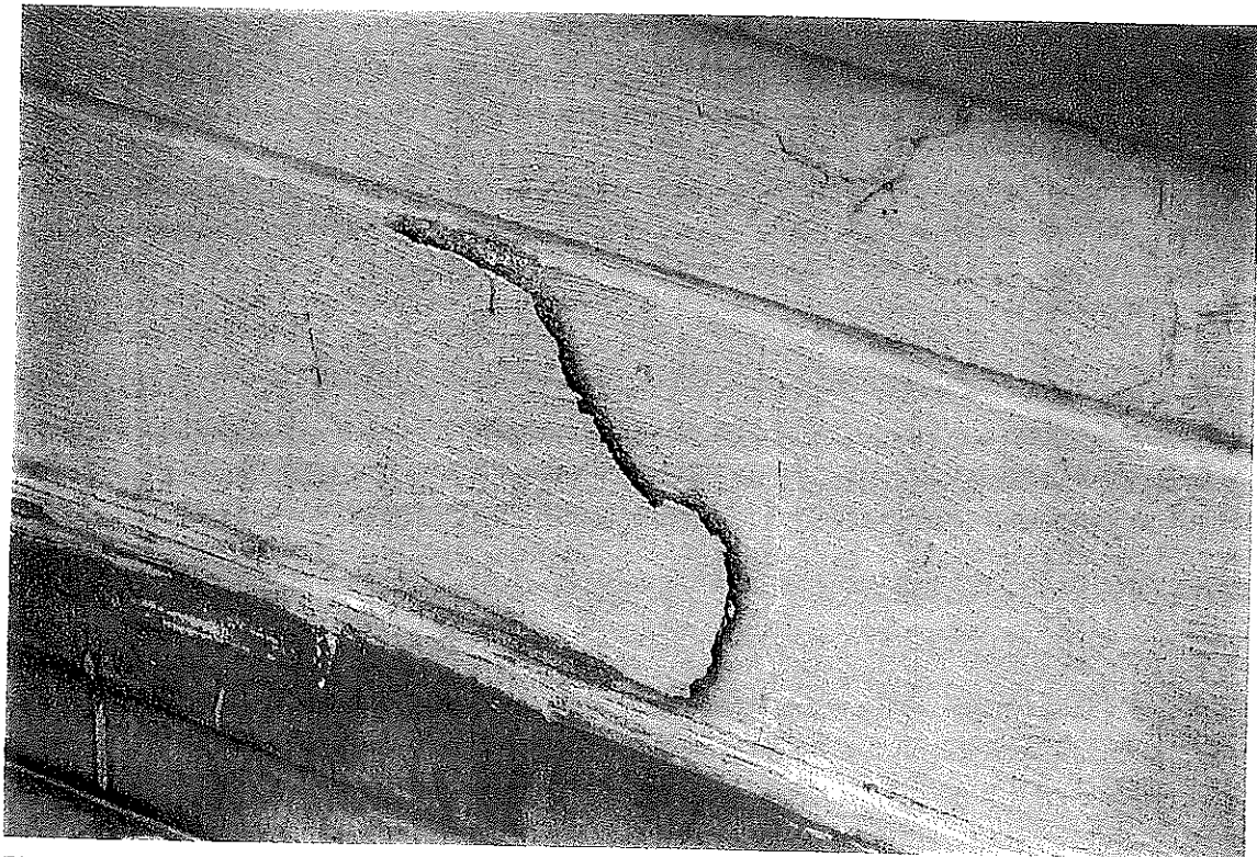
Photo No. 12 COATED INTERIOR FACE OF PENTHOUSE PARAPET WALL. NOTE SPALLED 10-4/2/98 MASONRY.
