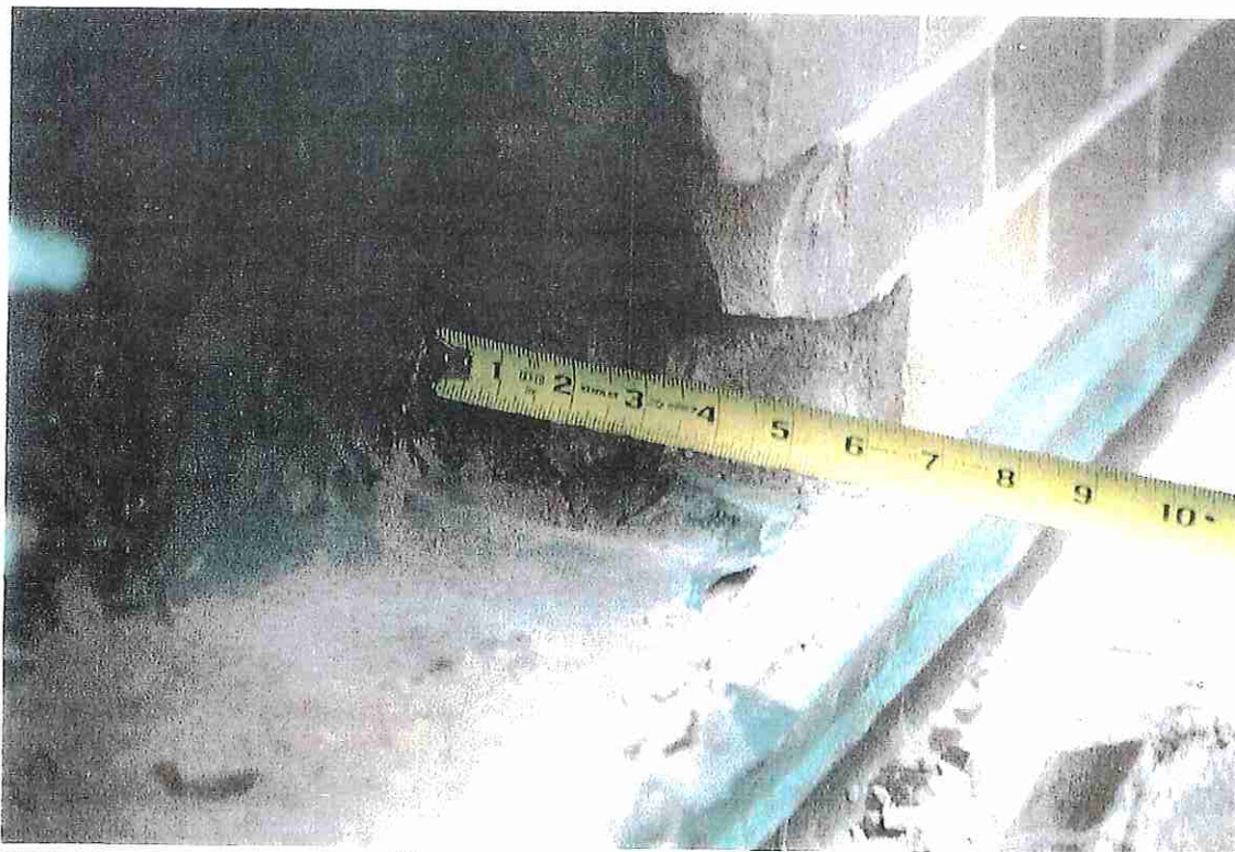
Photo No. 16 CUT NO. 3 - 17 TH FLOOR TERRACE. NOTE: 3" CAVITY WITHIN WALL AND 14A-4/18/98 FLASHING HELD BACK 1 1/2" FROM FACE OF BRICK.
