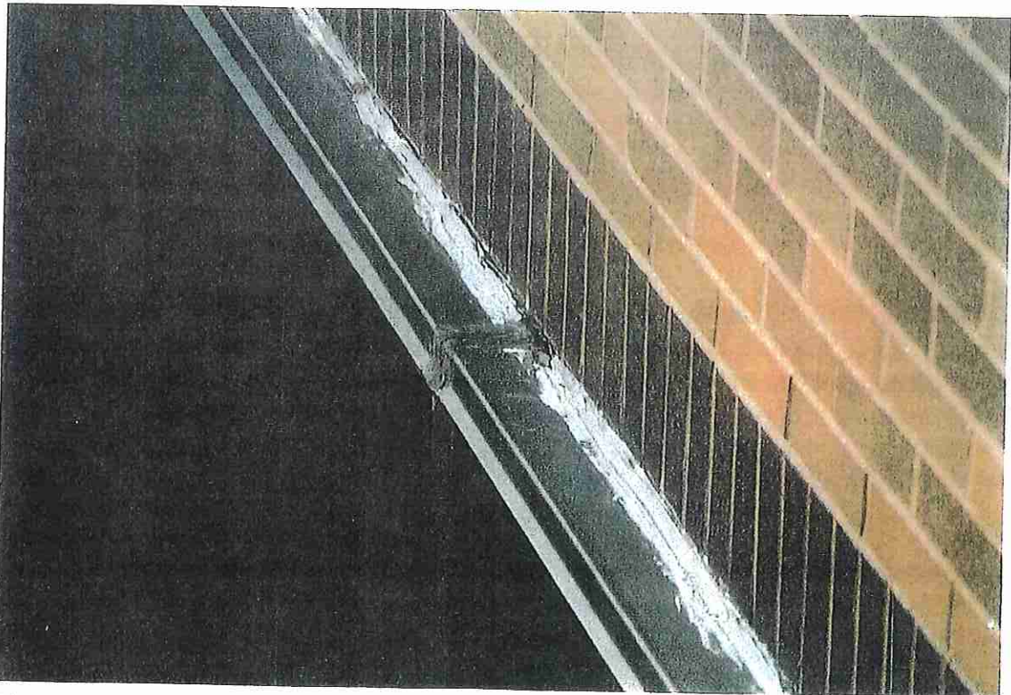
Photo No. 26 METAL CAP ON CURTAIN WALL TILTS BACK TOWARDS MASONRY AND PONDS WATER. NOTE POOR APPLICATION OF SEALANT AND OPEN SEAM.
