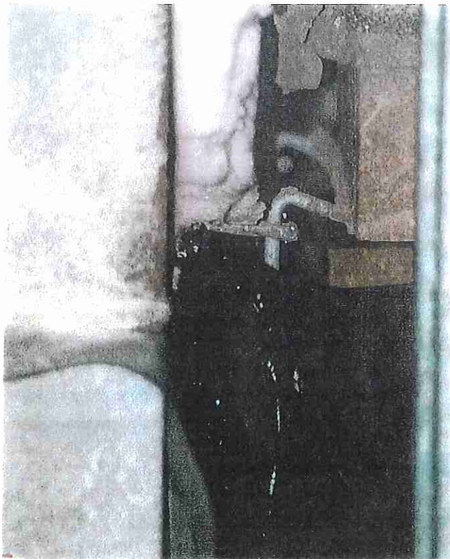
Photo No. 18 CLOSE-UP OF CAVITY WALL CONSTRUCTION. NOTE GALVANIZED MASONRY 17-4/2/98 ANCHORS AND FLASHING.
