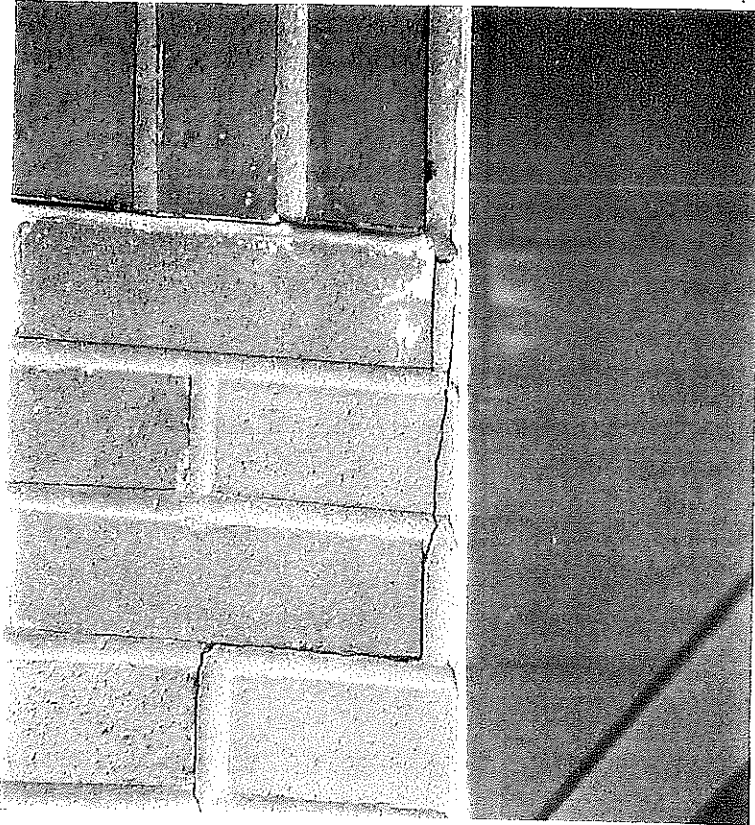
Photo No. 11 CLOSE-UP OF CRACK IN BRICK VENEER WHERE CURTAIN WALL ABUTS 19A-4/18/98 MASONRY.
