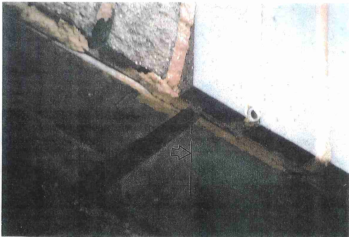
Photo No. 22 CLOSE-UP PHOTO OF LINTEL FLASHING CONDITION. NOTE FLASHING STOPS SHORT OF EDGE OF STEEL AND JOINT IS FILLED SOLID WITH MORTAR.
