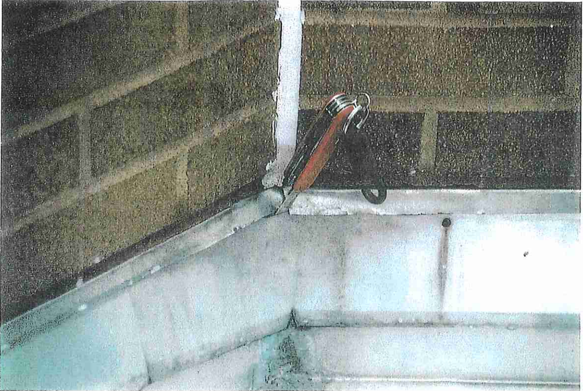
Photo No. 23 VOID IN SHEET METAL COUNTER FLASHING AT PARAPET WALL. 8-4/2/98
