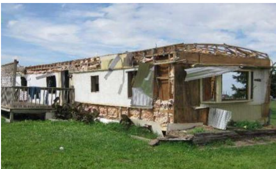
This manufactured home is missing the roof covering, and at least one wall has been compromised.
