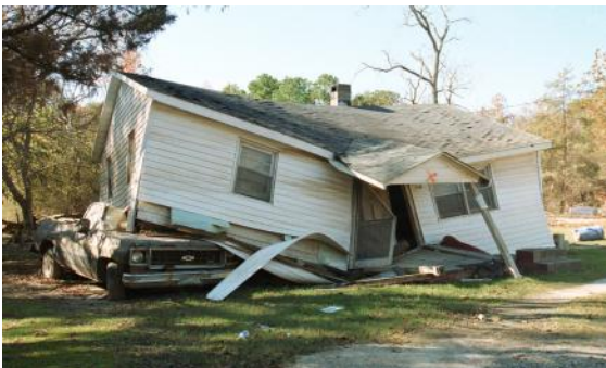
The roof and walls of this home have been compromised and it is off its foundation.
