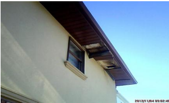
Damage to this soffit represents nonstructural damage to the roof.
