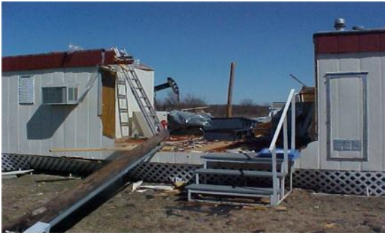
The manufactured home is missing the roof and at least two walls.
