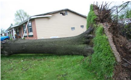
The residence has gutter and roof damage. The tree does not impact the damage level of the home.
