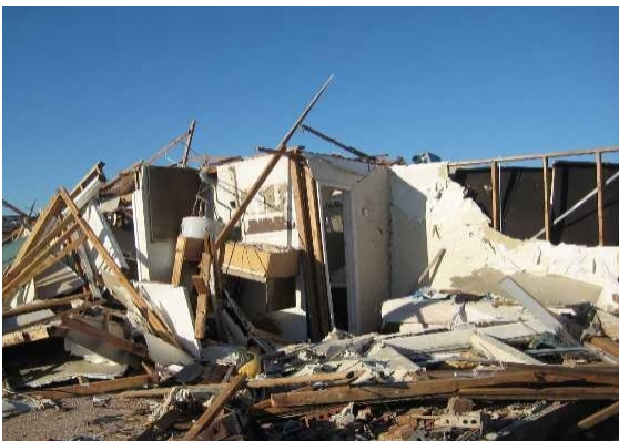
This residence has collapsed.
