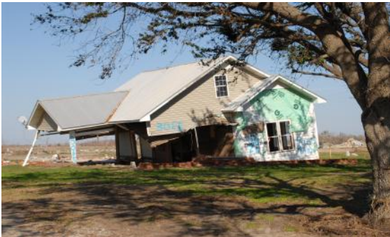
The foundation and two or more walls of this residence have failed.
