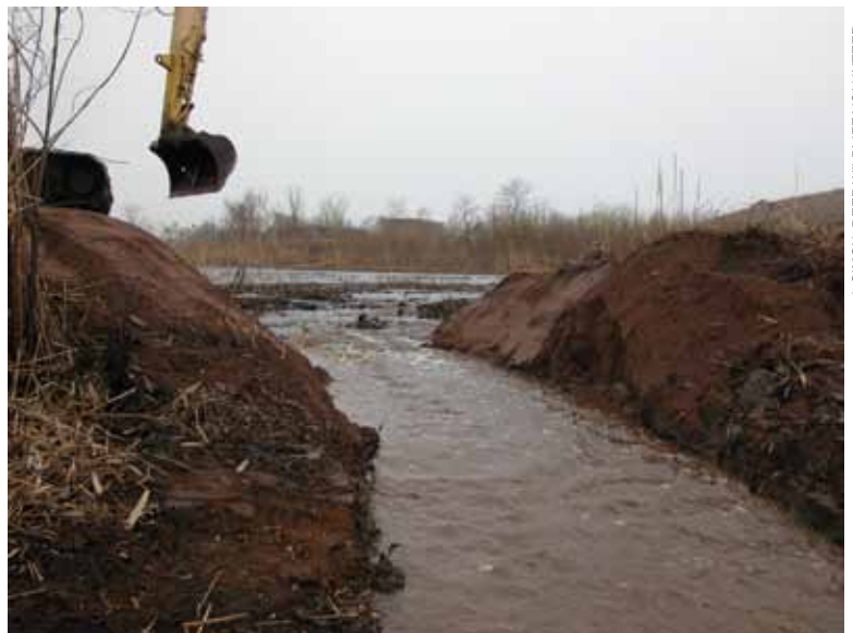
The WHAMM Program's excavator breaches a dike to restore tidal flow at the Little River marsh restoration site in New Haven/North Haven.
