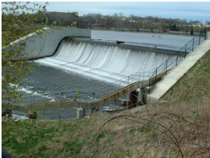
Dam and Fishway at Bunnell's Pond, Bridgeport (Source: C.Cryder, Save the Sound).
