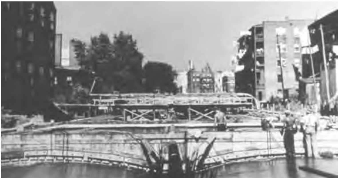
The Park River conduits during construction, circa 1942. (Hartford Collection, Hartford Public Library).
