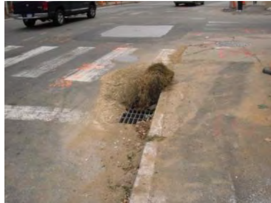
Figure 6-33. Poorly maintained catch basin grate in downtown Stamford
