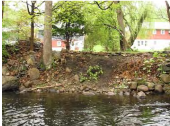
Figure 6-15. Eroded stream bank along Mill River
