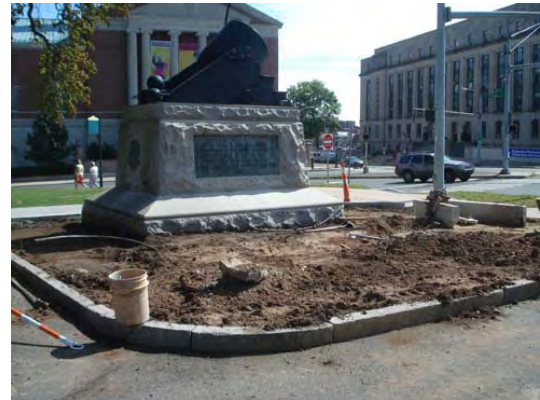
Figure 6.3.14 – Construction of a rain garden at Hartford Green Capitols Project. Source: Camp Dresser & McKee.
