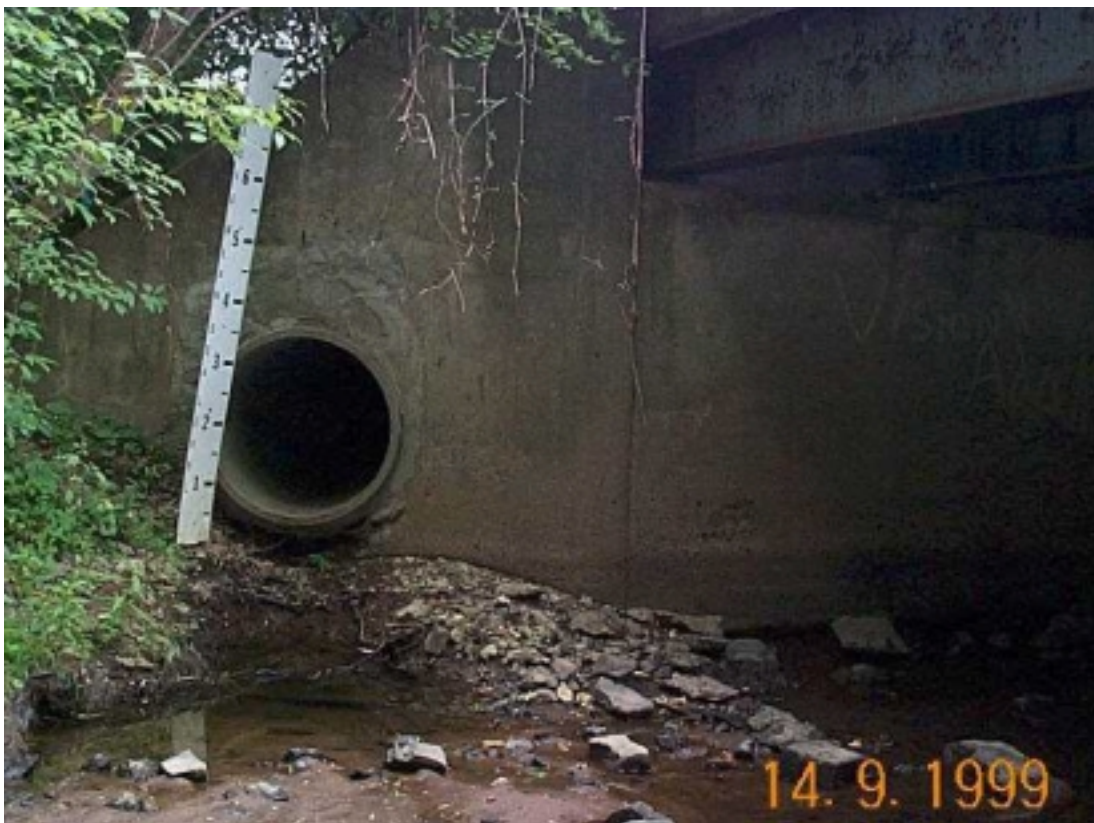
Farm River, East Haven, CT, August, 1999. Poorly constructed gaging station at a registered diversion. The staff gage is high and dry even though there is water in the channel, and the staff is leaning over, making any data collected from this gage inaccurate.
