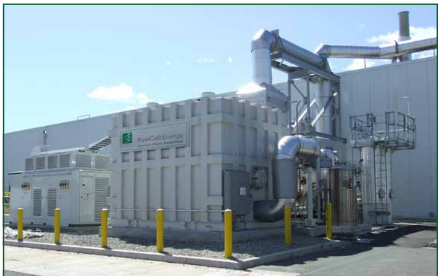
A FuelCell Energy installation at a commercial bakery in Bloomfield.
