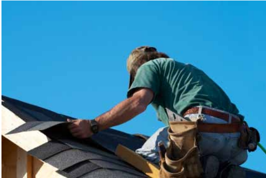
On average, a home re-roofing project can produce 4 tons of waste shingles
