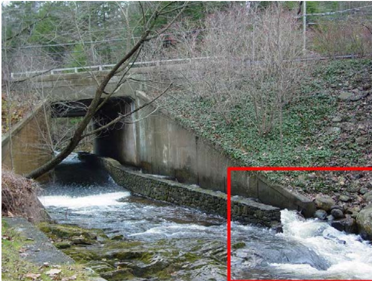
Figure 3. Pre-construction view of the fishway entrance and the downstream outlet of the culvert. Note the high velocities in both areas.
