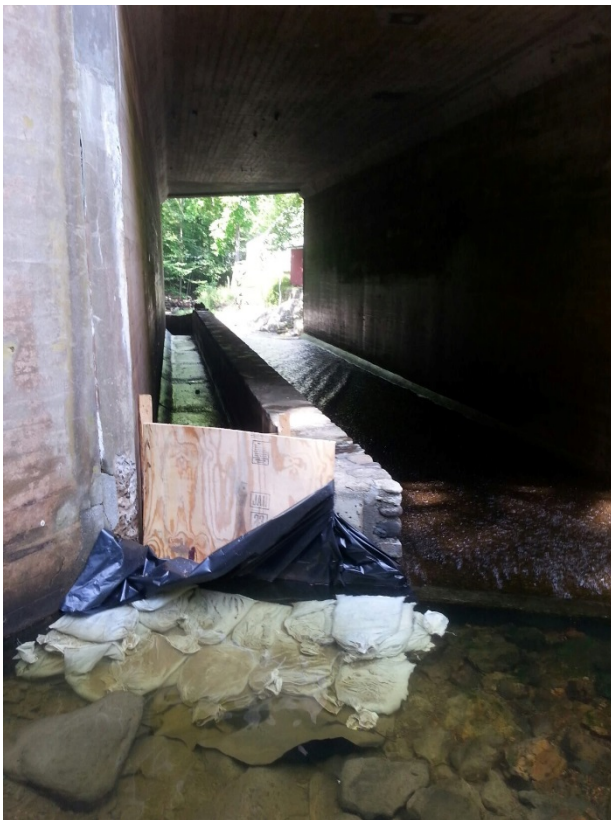
Figure 6. Cutting off the flow through the fishway to allow work to begin.
