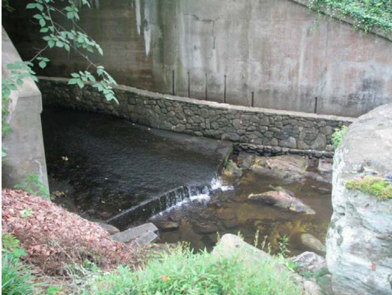
Figure 2. Pre-construction view of the downstream end of the culvert. Note the fast, shallow water flowing over the concrete bottom.
