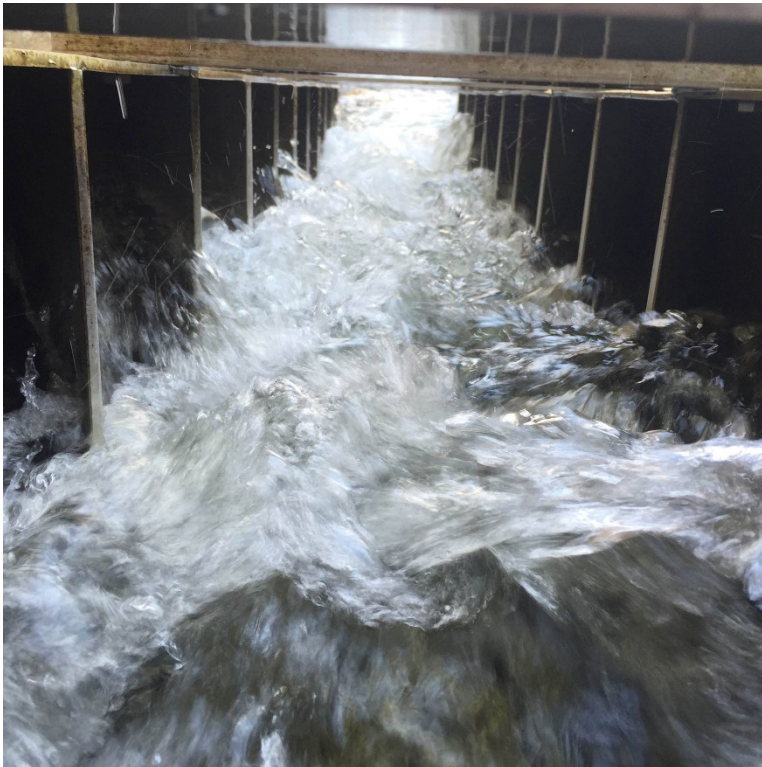
Figure 13. The baffles of the fish ladder allow native brook trout to more easily pass through the culvert and return to primordial spawning grounds.
