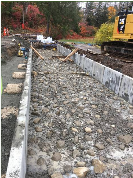
(left) Longitudinal view of the culvert at Chalker Brook after installation of the cobble weirs and grouted substrate.
