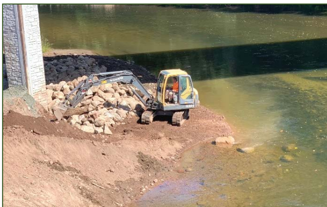
(Left) A contractor works to install the first “tooth” of a sawtooth deflector along the western bank abutment during low water conditions.
