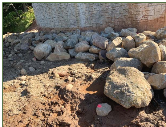
(Right) Post-construction view of a recently completed sawtooth deflector along the eastern bank abutment.
