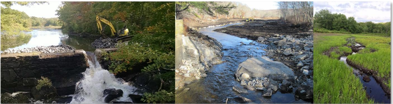
Ed Bills Pond Dam Removal - East Branch Eight Mile River Restoration, Lyme
