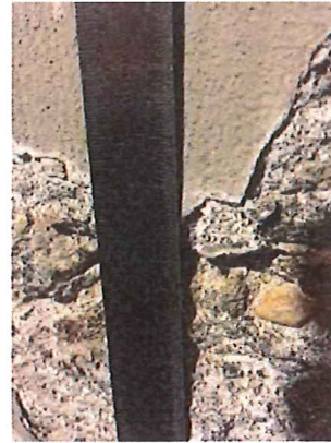
d) crack opening (>4mm)
