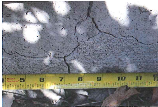
(c) wide crack opening
