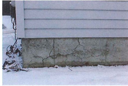
(c) map cracking
