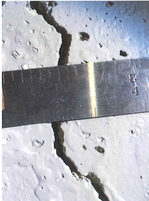
(c) wide crack opening
