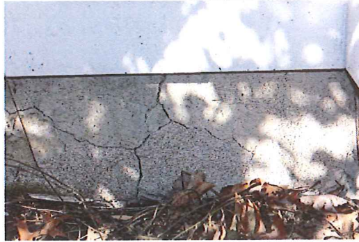
(b) map cracking
