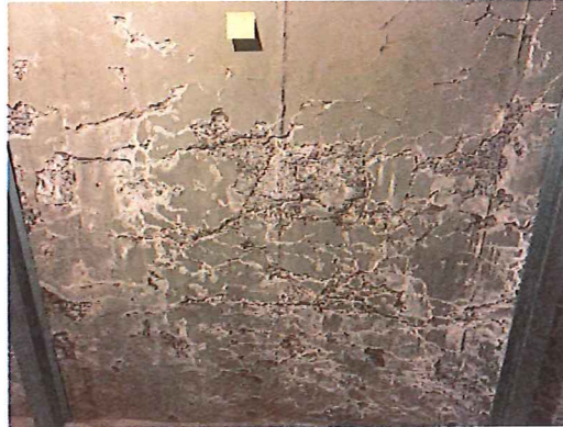
(c) map cracking
