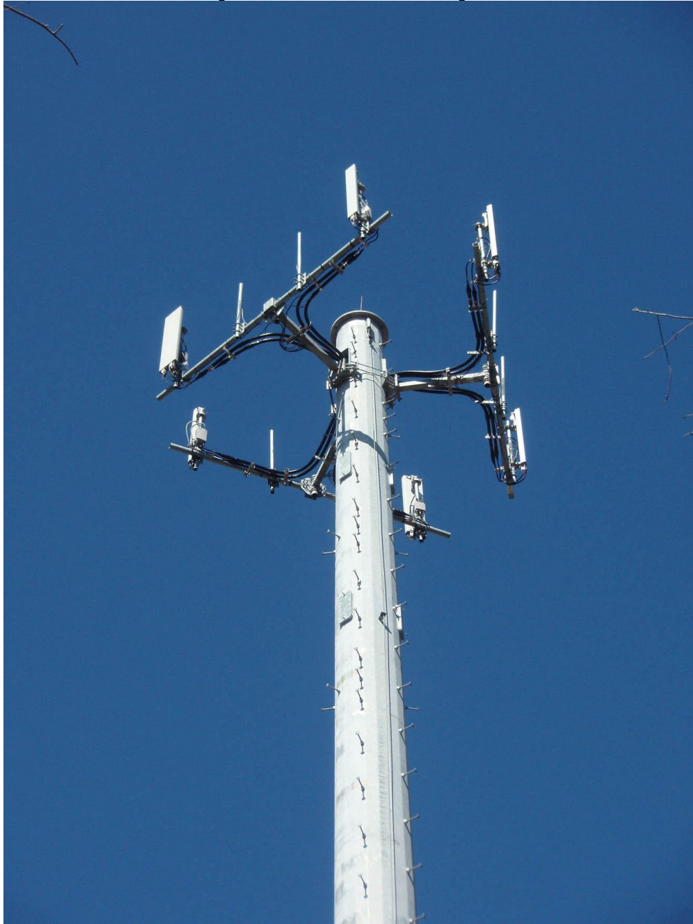
Close up of antennas mounted at top of tower
