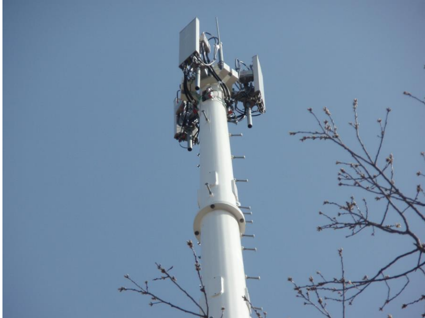
T-Mobile's antenna installation
