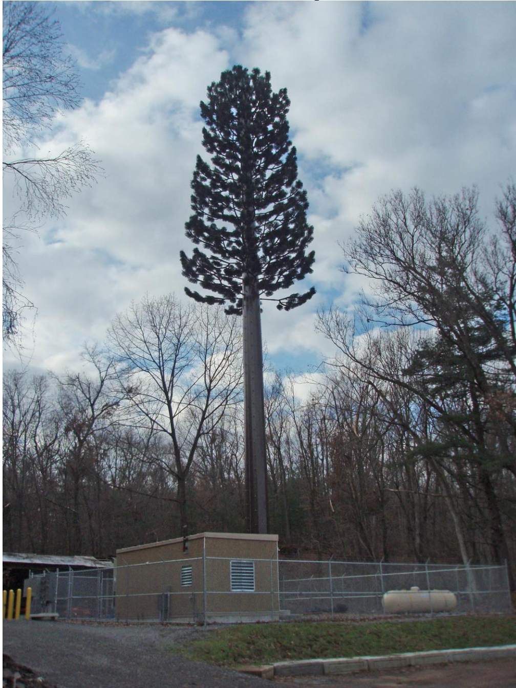
View of tower and compound
