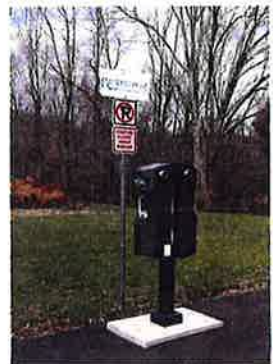
Electric Charging Station Pomfret Town Hall
