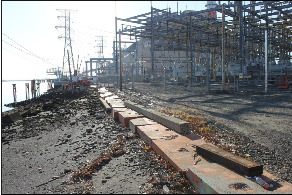
Figure 1-3: Existing Pequonnock Substation: Northeastern Boundary adjacent to Bridgeport Harbor (View to South)
