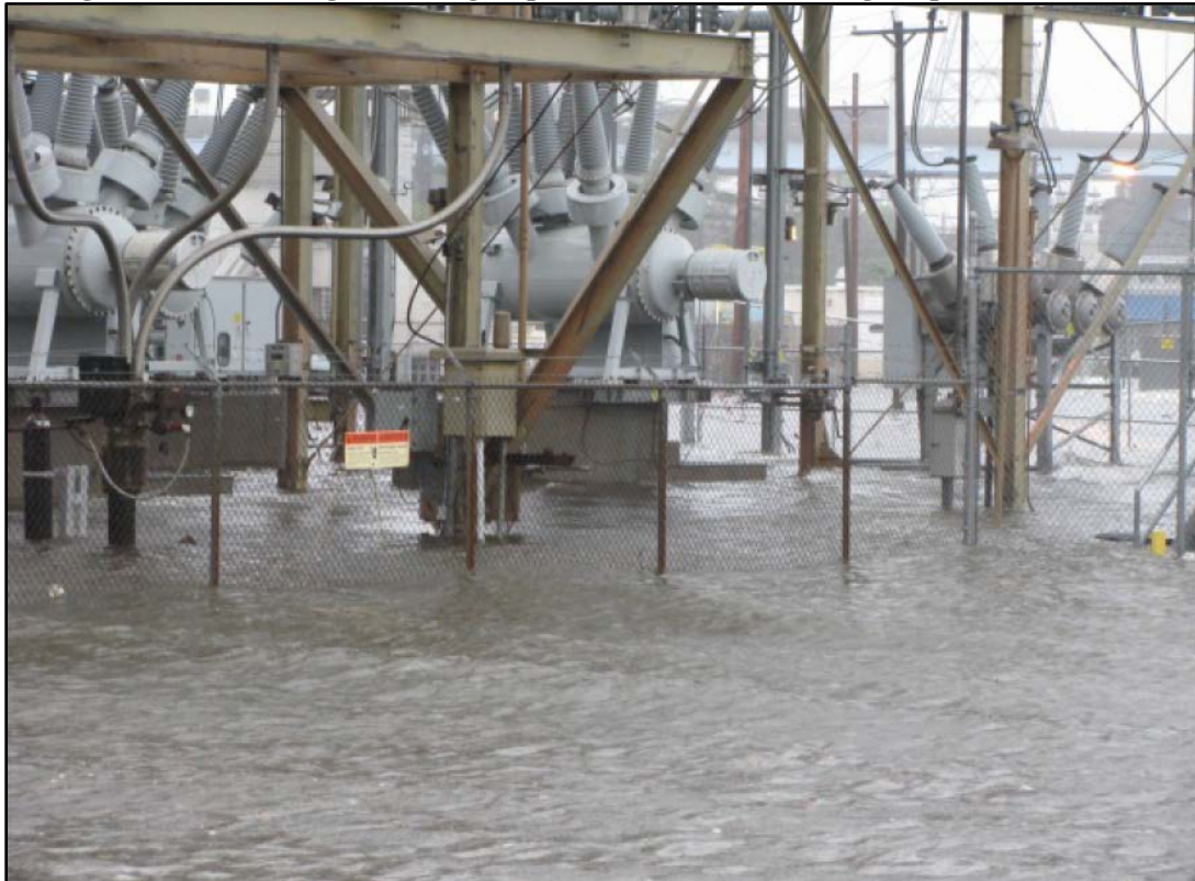
Figure ES-3: Flooding at Existing Pequonnock Substation during Tropical Storm Irene
