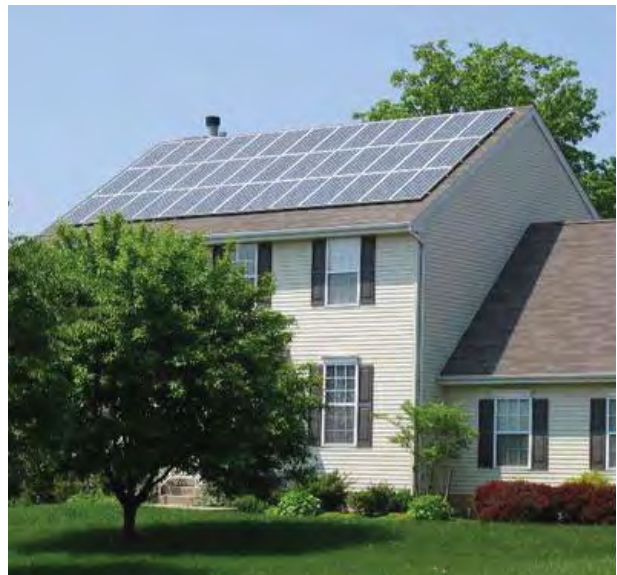
Roof-mounted solar panels | Source: Stantec
