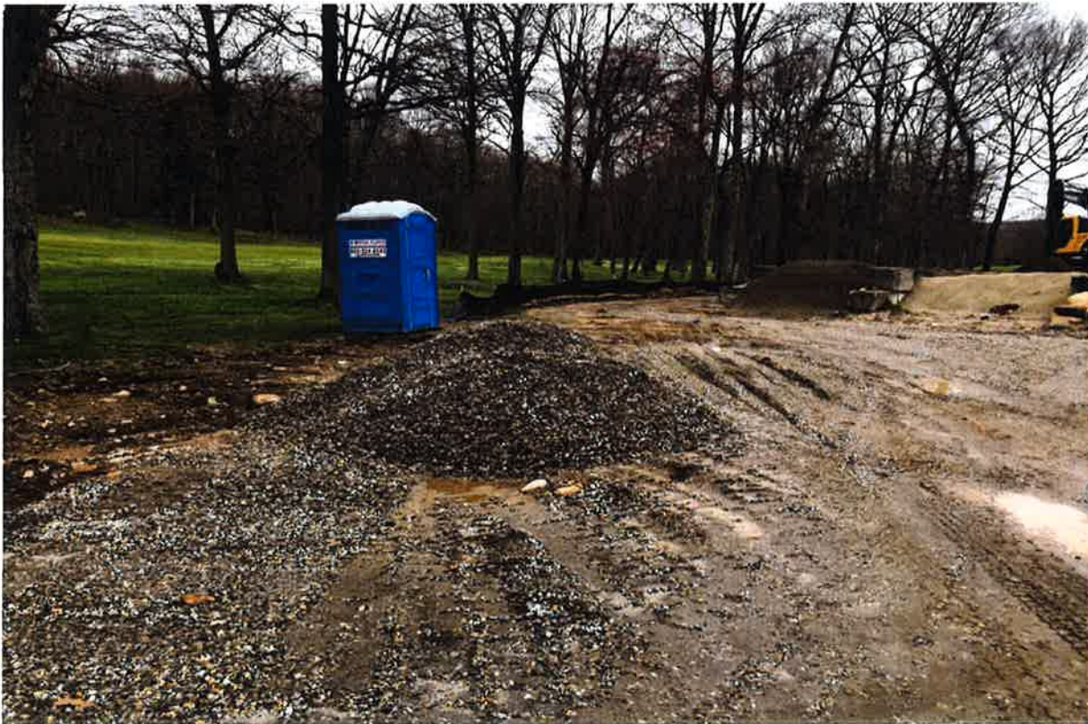
Photo 4: View of final utility trench backfill stock pile area to be removed.
