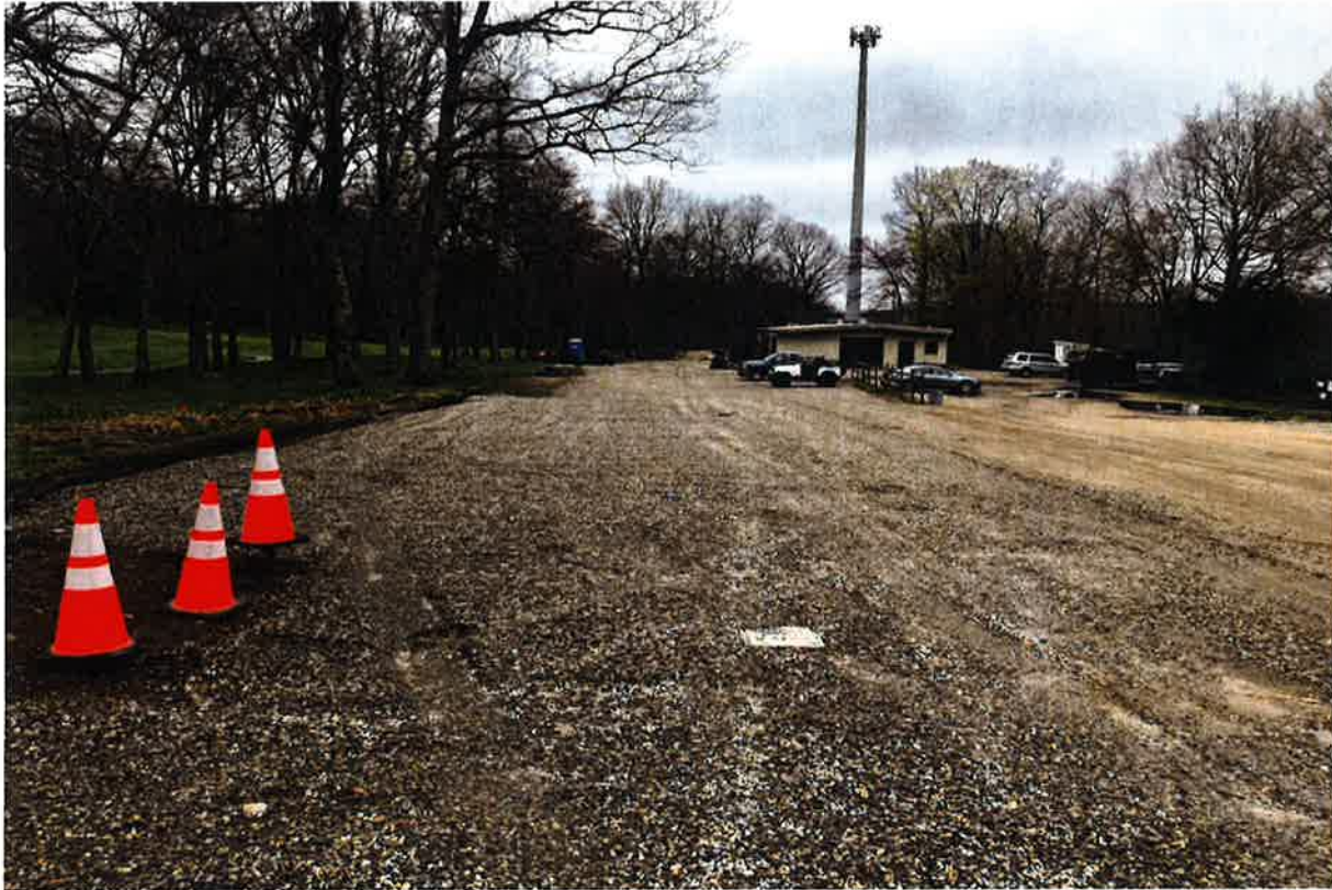
Photo 3: View of buried electrical work along access road.
