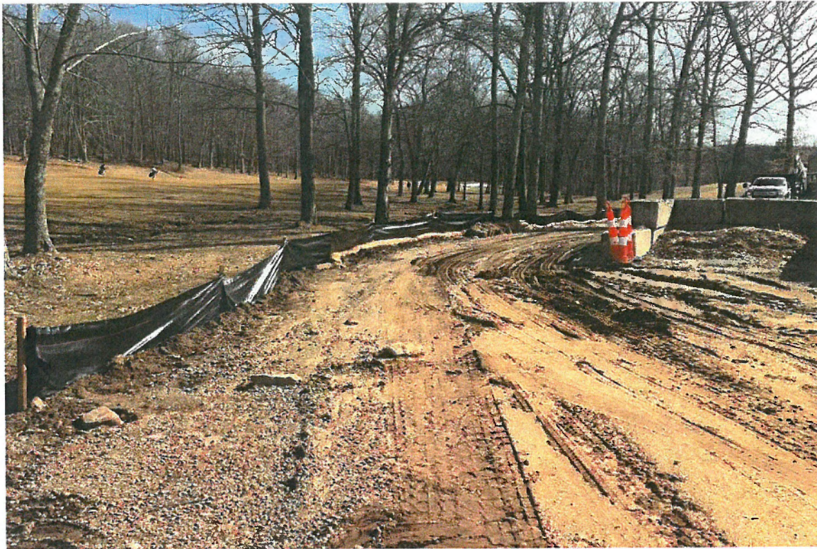
Photo 7: View of reinforced controls by bulk storage bins.
