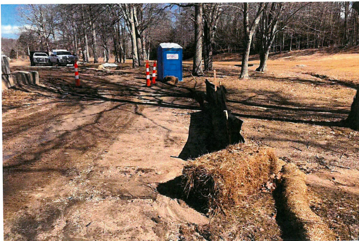
Photo 6: View of perimeter controls by bulk storage bins.
