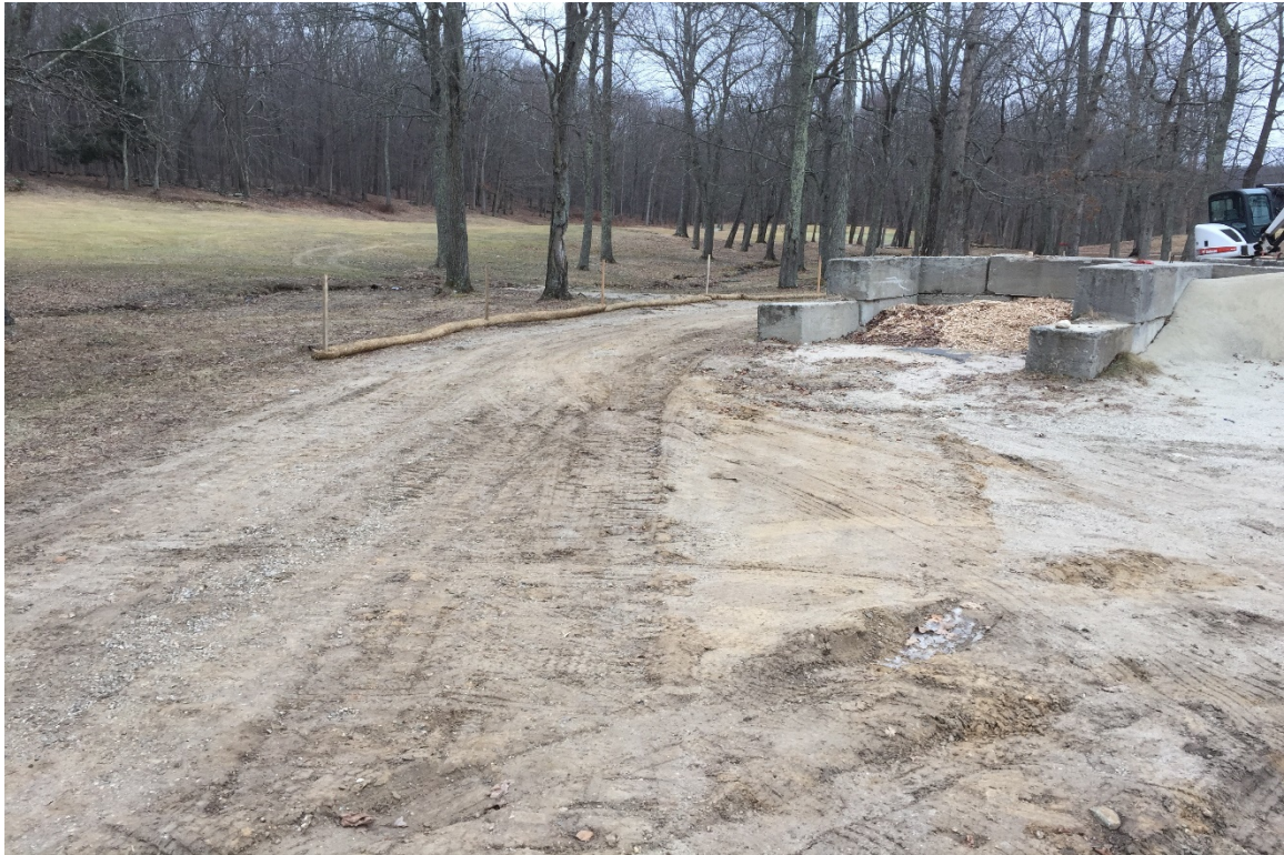
Photo 1: View of existing washout location near the bulk storage bins.
