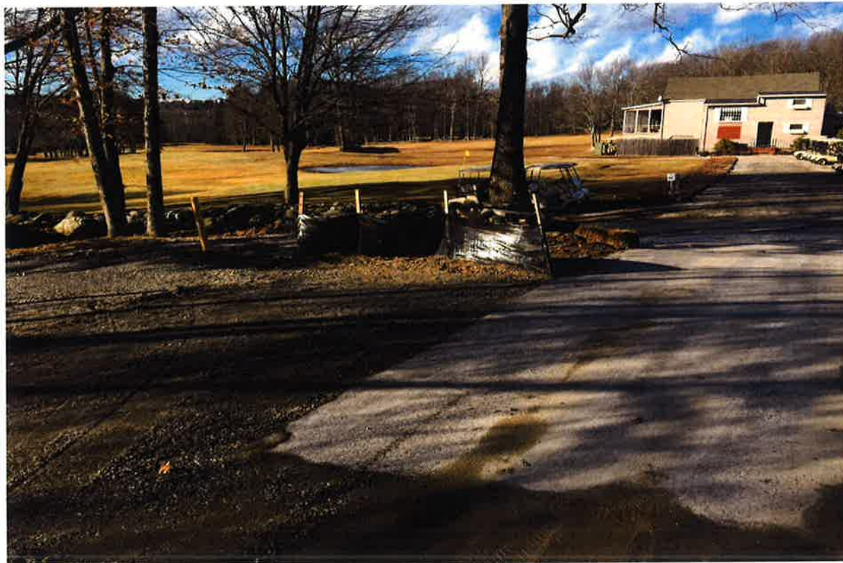
Photo 12: View of construction entrance with erosion controls installed. Photo taken on February 8, 2019.
