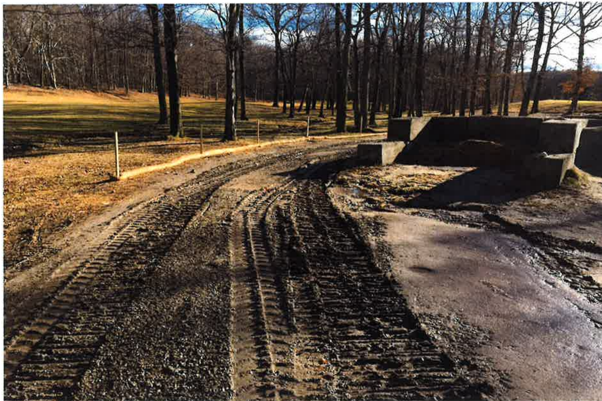
Photo 4: View of pre-existing washout by bulk storage bins. Photo taken on February 8, 2019.
