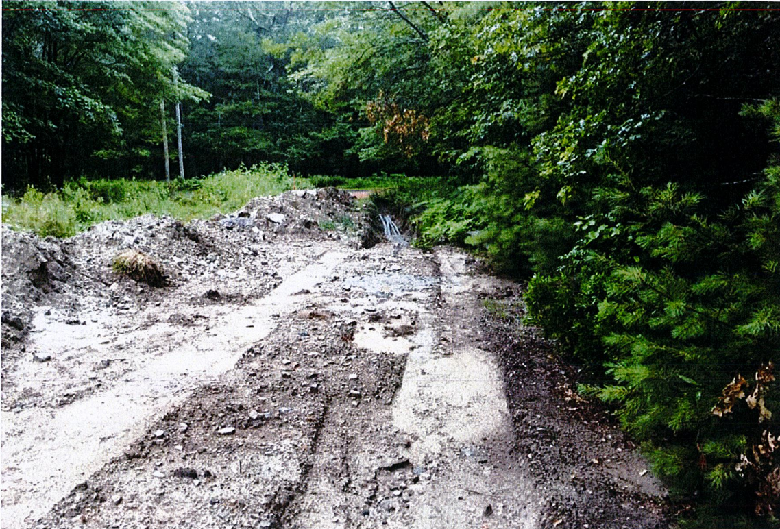
Photo 1: View of utility conduit trench looking west with Bailey Hill Road in background.
