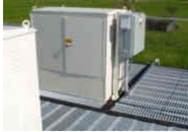
Package treatment plant
